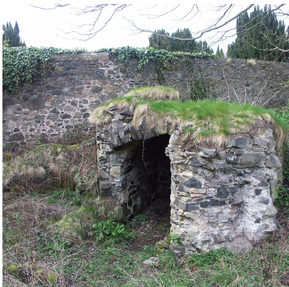
Fig. 3.25: Monimail Tower, Fife (CS27). The flat upper surface allows some moisture to penetrate through the capping. A thicker clay layer might have adequately improved performance.
