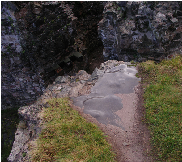
Fig. 3.32: Inverlochy Castle, Inverness-shire (CS21). Asphalt coated concrete cappings revealed after erosion of the soft capping by pedestrian traffic.
