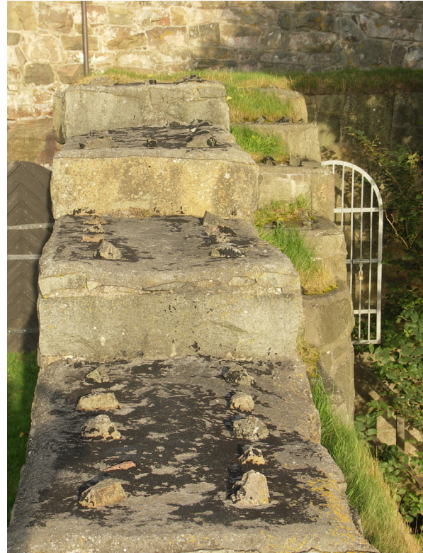
Fig. 3.29: Varberg Fortress, Sweden. Textured wallhead with bitumen remnants failed to withstand wind decay
