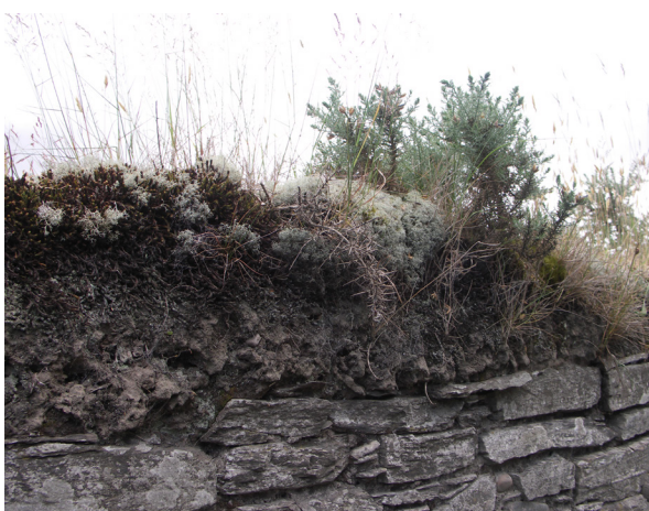
Fig. 3.54: Gordon Estate Walls, Moray. An old vernacular capping with a high arched profile giving steep sides.
