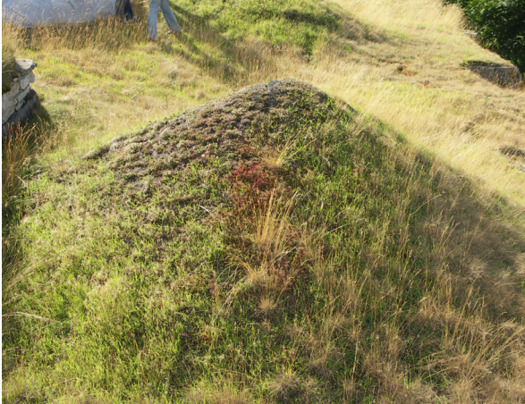
Fig. 3.9: St Nikolais' Church, Visby, Sweden. The effect of orientation on a site with high solar exposure and little ability to store moisture: sedum mats are failing on the south side, but stable on the north of shallow domes.
