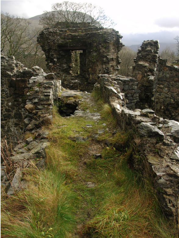
Fig. 3.20: Inverlochy Castle, Inverness-shire (CS21). The cappings are applied to the walkway surface but not to the parapets.
