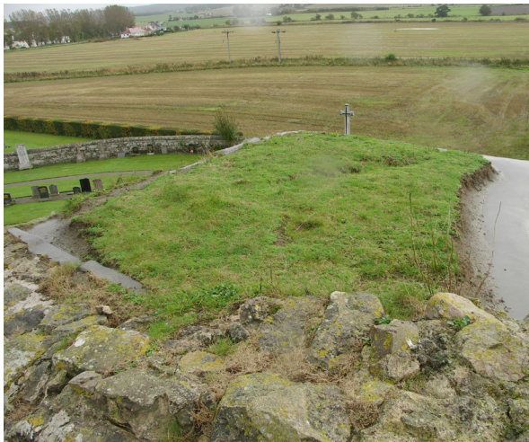
Fig. 3.56: Kinloss Abbey, Moray. Severe and progressive edge decay over an asphalt capped concrete cap.
