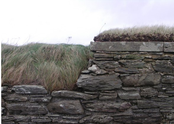
Fig. 3.27: Kilbrannan Chapel, Argyll (CS22). The smoothness of the dressed cope edges meant the soft capping stabilised ~50mm back from the edge, a feature not found on the rough raked wallhead.
