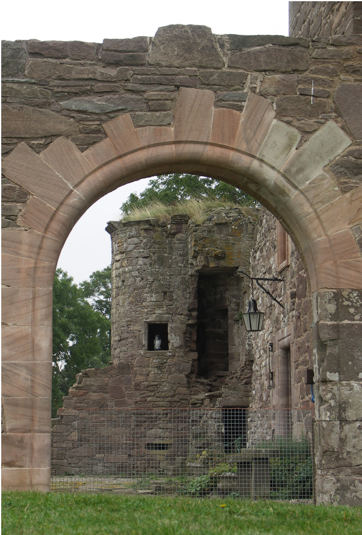
Fig. 9.1: Melgund Castle, Angus (CS26), where the role of vegetation in a restoration project was well considered.
