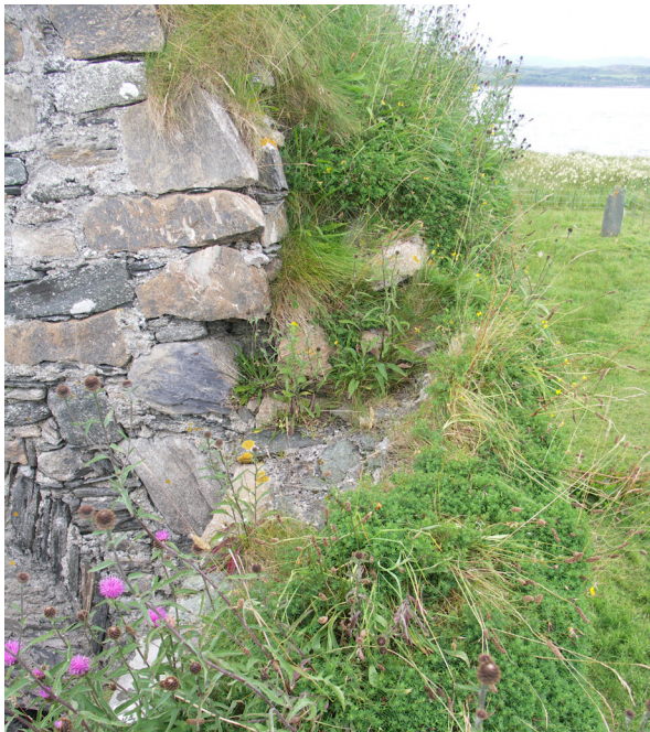
Fig. 3.16: St. Cormac's Chapel, Eilean Mor, Argyll (CS1). Localised effects are hard to predict. Wind currents here focus on an inner corner of the capping, scouring away any soil, while the exposed outside edge has stable, thick growth.
