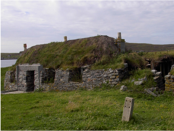
Fig. 5.4: Decaying Blackhouse, Berneray. A decaying roof deposits composted thatch and turf underlay.
