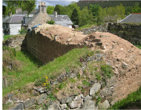
Fig. 2.26: Braemar Castle. The masonry wall face on the right is stained by soil washed off the failed capping.
