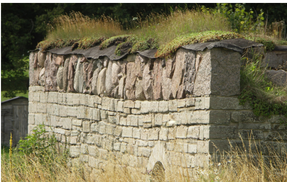
Fig. 3.59: Alvastra Monastery, Sweden. Sedums struggle to stabilise on a smooth, dark, impermeable membrane.
