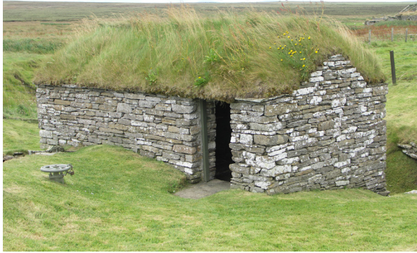
Fig. 4.26: Dounby Click Mill, Orkney (CS7). Roof renewed c. 1980 in a relatively sheltered location.
