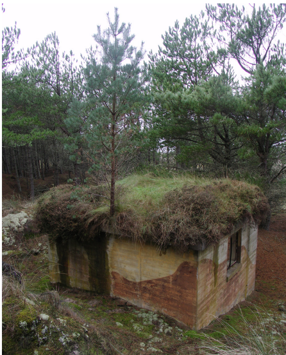
Fig. 3.47: Coastal Defences, Moray, constructed c. 1941. A tree invades the capping vegetation, which fulfilled the same camouflage function as that painted on the walls. This exceptional tree is a direct result of the bountiful supply of pine cones, shade and shelter provided by the surrounding forest.
