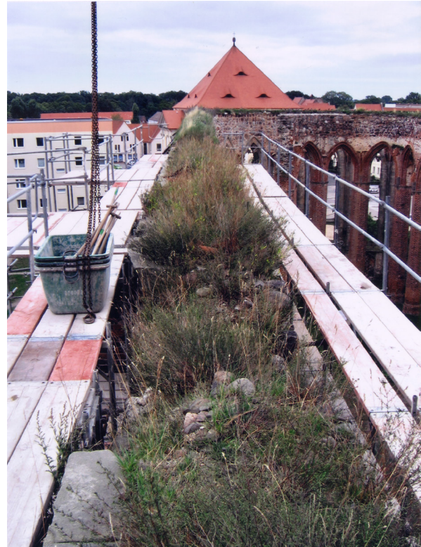
Fig. 7.30: St. Nicolai's Church. The natural vegetation did not give a stable wallhead.
