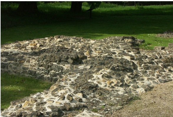
Fig. 2.9: Hailes Abbey, Gloucestershire, England. Hydraulic lime repairs to cement hard caps can be difficult and expensive. The process of removing defective cement can also be very damaging to weaker stone types.
