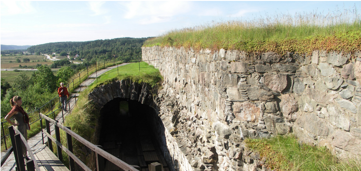
Fig. 7.8: Bohus Fortress, west Sweden, east facing walls. The soft cap achieves a stable edge, but the species clearly indicate this a modern conservation capping, rather than a natural or vernacular cap.
