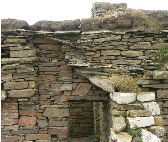
Fig. 2.21: Eynhallow Monastery, Orkney (CS18). Even dead cappings can protect loose masonry by their weight.
