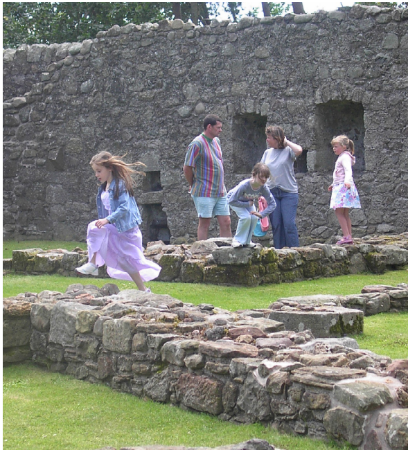
Fig. 2.17: Loch Leven Castle. Kinross-shire, Even on a manned site, rough racked masonry can suffer under the feet of visitors.
