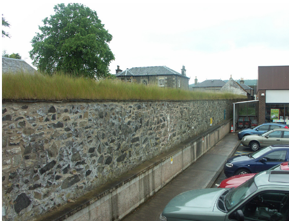
Fig. 2.38: Peebles Town Wall, Peebles, Peebles-shire. Commercial turf has resulted in low visual diversity, giving an even appearance, arguably appropriate for an urban setting.
