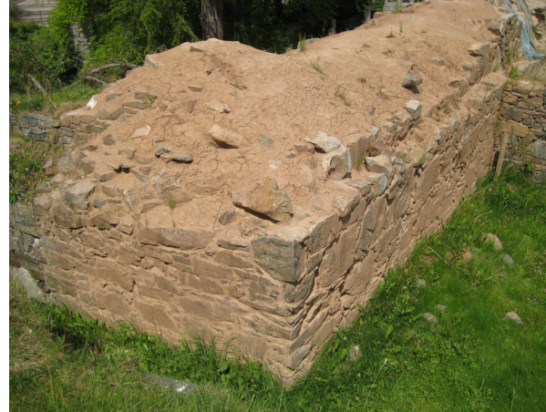
Fig. 3.10: Braemar Castle, Aberdeenshire. Following complete failure of the vegetation, the clay cap has dried and cracked. Such a surface could be colonised by more appropriate species in time.
