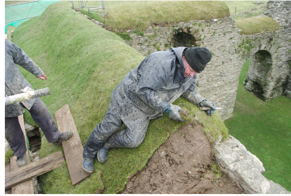
Fig. 3.18: Skipness Castle, Argyll (CS35). The soft capping varies in depth to provide a regular, water-shedding surface.
