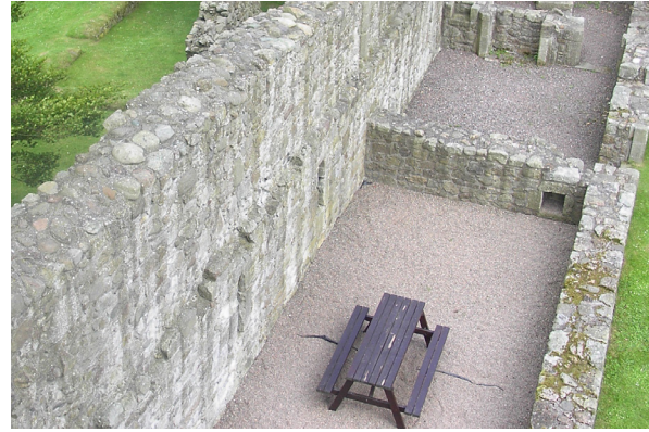
Fig. 2.7: Loch Leven Castle, Kinross-shire. The consolidated wallheads do not preserve the original fractured masonry exactly as found, while focused rainwater run off results in unsightly surface staining. Note the natural colonisation by mosses of the lower walls, which do not have the domed profile of the higher wall consolidation
