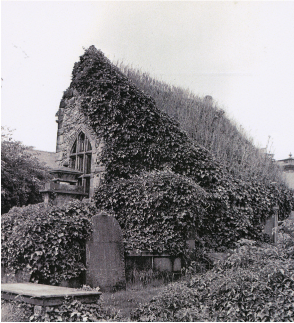
Fig. 6.3: St. Mary's Church, Banff, prior to intervention.
