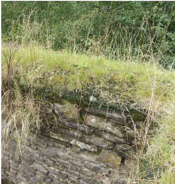
Fig. 2.15: Doune Castle Mill, Stirlingshire (CS15). The clay and turf cap fails to prevent moisture penetration into the wallhead.
