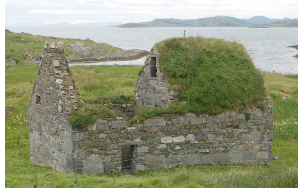
Fig. 2.13: St. Cormac's Chapel, Eilean Mor, Argyll (CS1). The natural vegetation acts as a living thatch. The complex matrix of foliage disperses rainwater runoff, which is largely cast clear of the wall.
