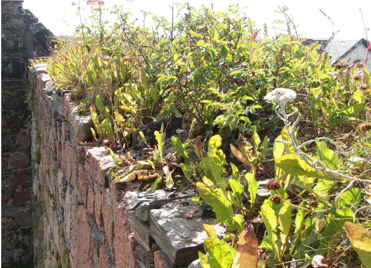
Fig. 3.38: The Nunnery, Iona, Argyll (CS28). Removal of natural caps has allowed colonisation by roses and dandelions, whose penetrating roots will damage the masonry.
