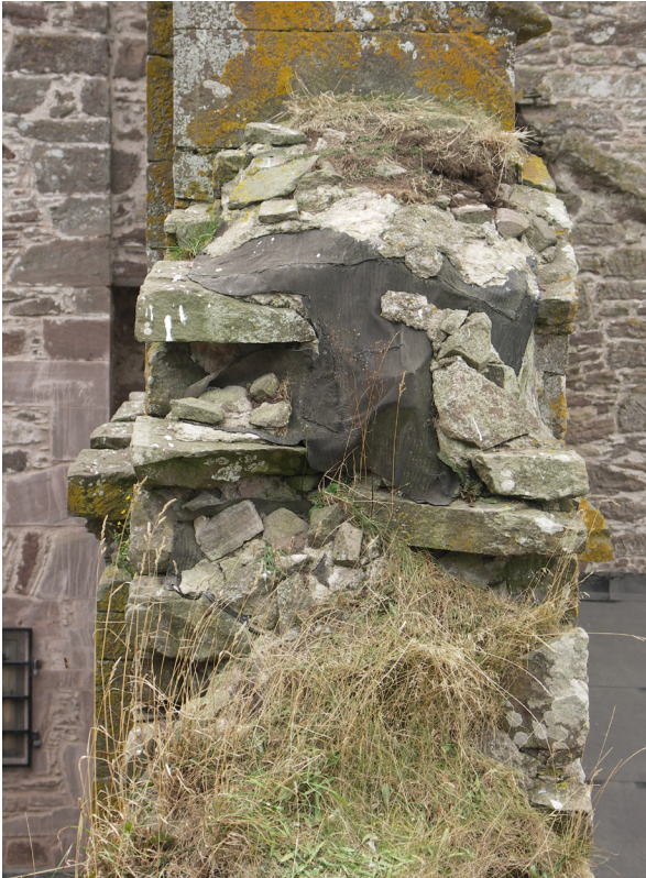
Fig. 3.61: Melgund Castle, Angus. Soft cappings fail over shallow masonry on bitumen-coated lead dpc's.
