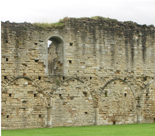
Fig. 2.12: Kirkham Priory, Yorkshire. In tests, soft cappings have reduced rainwater runoff, lowering moisture levels on the upper face of the masonry wall. As a result, the dark stains of damp and associated microflora on the upper wall face have begun to fade.
