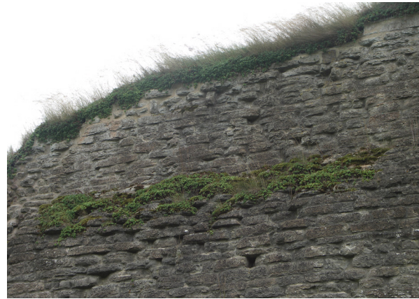
Fig. 3.44: Alvatsra Monastery, Sweden. Pieces of sedum have dropped from the main capping to colonise ledges below, naturally spreading to protect vulnerable masonry surfaces.
