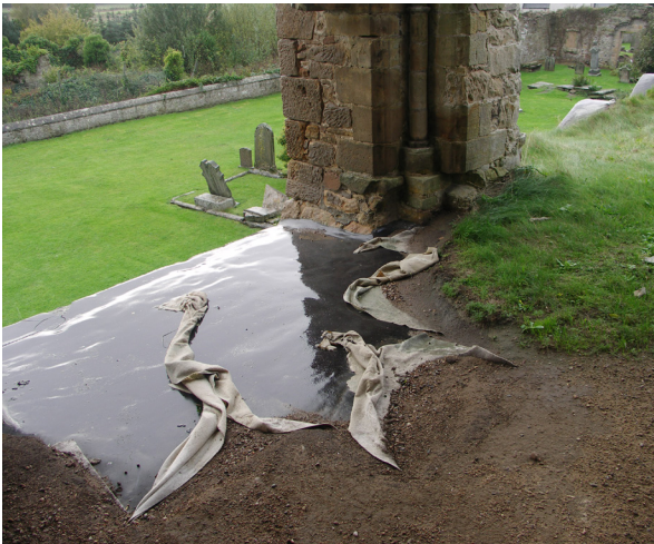
Fig. 3.64: Kinloss Abbey, Moray (CS24). Vandal damage to soft cappings.
