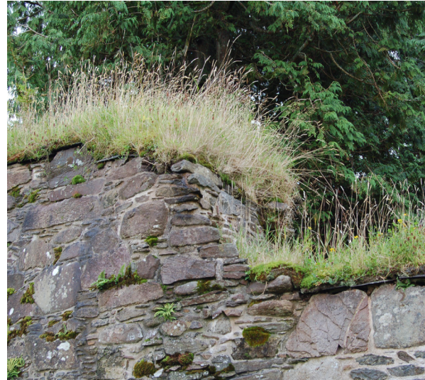
Fig. 3.60: Saddell Abbey, Argyll. The slate dpc has contributed to unstable edge conditions and visually detracts from the original masonry wallhead.
