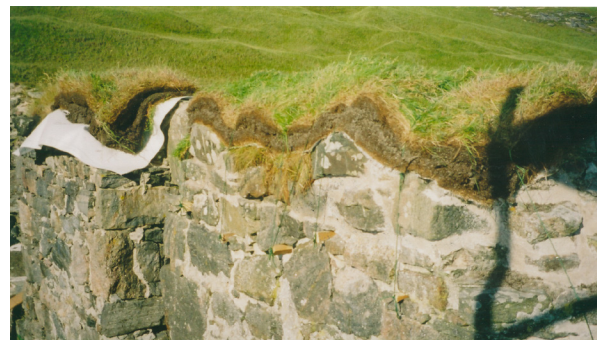
Fig. 3.19: Pabbaigh, Western Isles (CS33). The soft cappings, two layers of turf, root to root, are worked into the sockets left by decayed timber rafters. A permeable geotextile membrane, used as a defining layer, can be seen being installed on the left.
