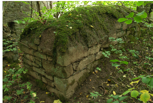
Fig. 3.4: Doune Castle Mill, Stirlingshire. A shaded cap is unable to sustain vegetation other than moss, with the clay saturated and sliding off steep sections.
