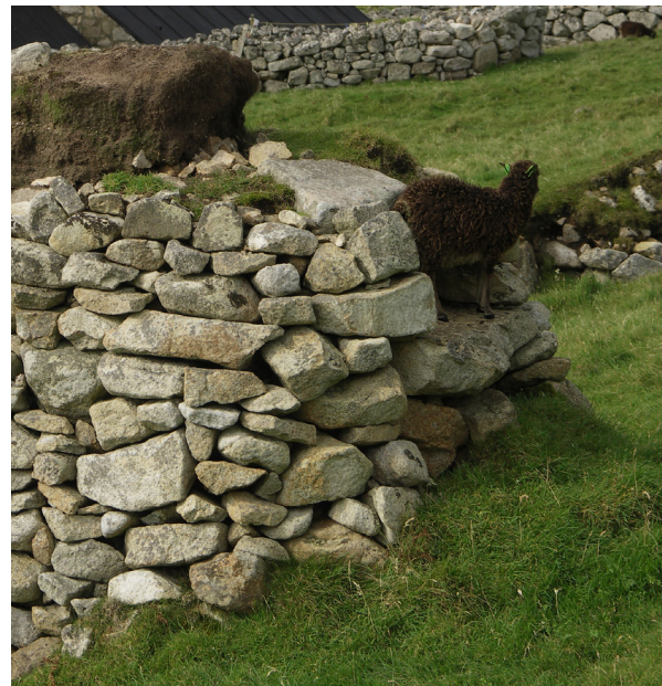
Fig. 2.19: Cleit 23, St. Kilda (CS7). Progressive decay of the soft capping may have been initiated by damage from the feet of sheep climbing on to graze.
