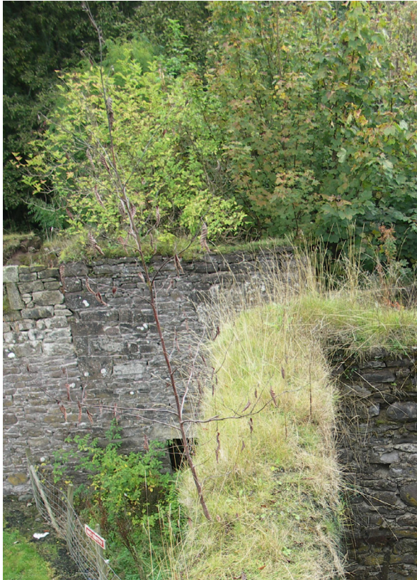
Fig. 2.22: Doune Castle Mill, Stirlingshire (CS15). This isolated tree sapling would probably die naturally, but its removal would be prudent.
