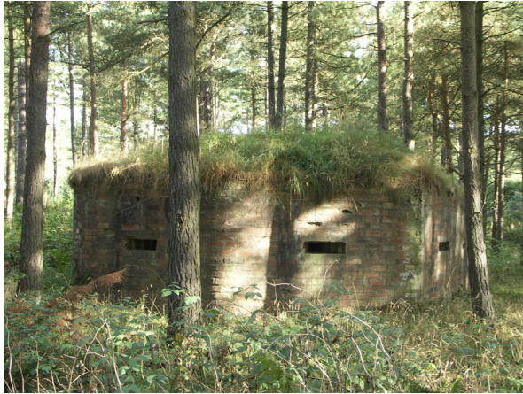
Fig. 3.5: WW2 Pillbox, Fife (CS12). The woodland shade reduces wind exposure and solar radiation and increases relative humidity.
