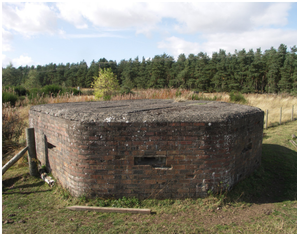
Fig. 3.6: WW2 Pillbox, Fife. High solar exposure, along with wind exposure and density of the substrate, has contributed to complete loss of the capping.
