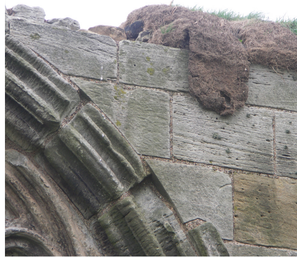
Fig. 3.57: Whitby Abbey, Yorkshire. The doubled-under edge turf has failed to root into the soil bed, leaving it vulnerable to wind lift.
