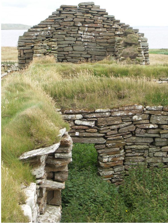
Fig. 2.20: Eynhallow Monastery, Orkney (CS18). Soft cappings here act as a weak ring beam, restraining movement in vulnerable wallhead masonry.
