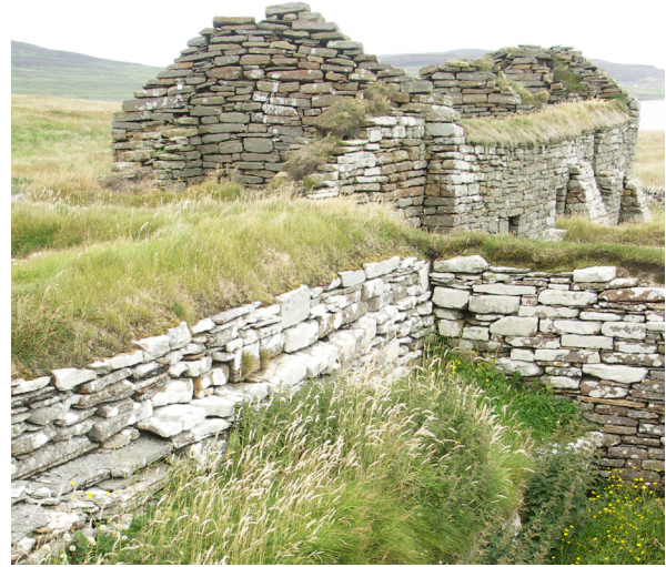
Fig. 2.36: Eynhallow Monastery, Orkney (CS18). The wallhead vegetation is conservation soft capping from several periods, dating back probably to c.1920.
