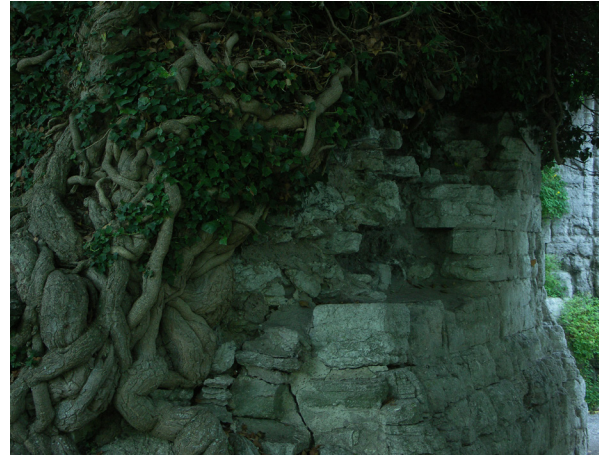
Fig. 8.5: St. Olof's Church, Visby. The ivy stems grip the masonry, causing local damage.
