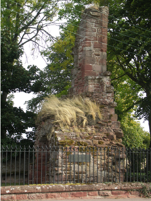
Fig. 3.8: Coupar Angus Abbey, Angus. The west facing side is exposed to much more solar radiation than the rest of the capping, resulting in local dieback.
