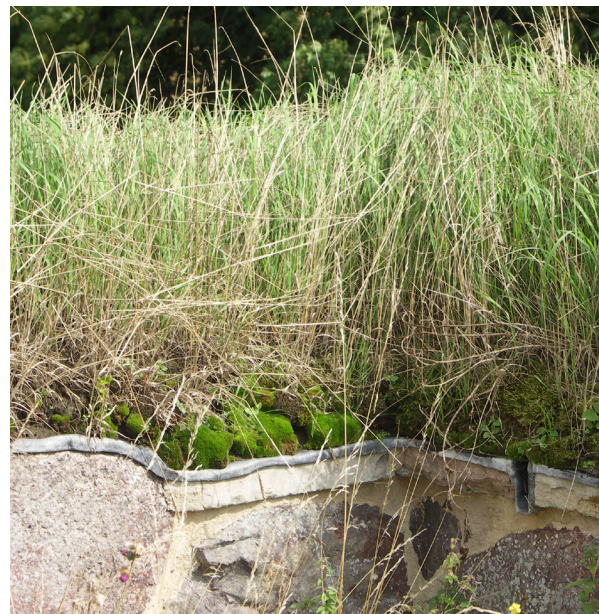
Fig. 1.5: Alvastra Monastery, Sweden. The vegetation grows in lead containers on the wallhead.
