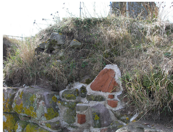
Fig. 6.2: Cessford Castle, Roxburghshire (CS2). Masonry repairs were only required at the edges.
