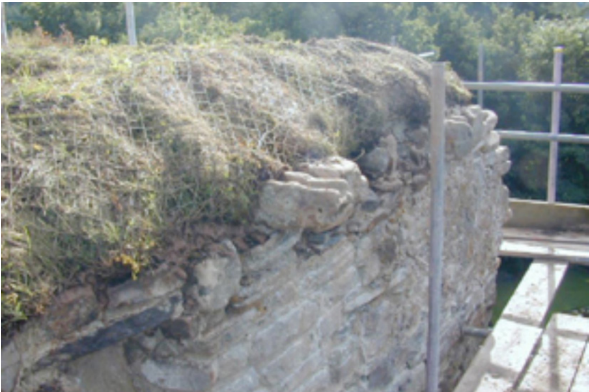
Fig. 5.7: Drumin Castle, Moray. Plants removed from the walls before the repairs were reinstated, with biodegradable mesh as a temporary fixing.
