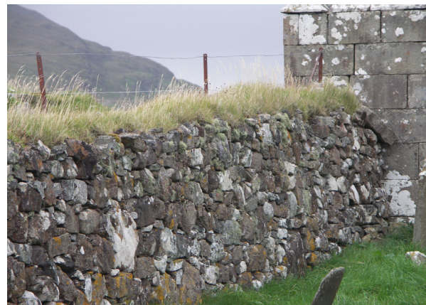
Fig. 4.6: A domed turf capping, with wire fencing as stock proofing, Roghadal Church, Harris (CS37).
