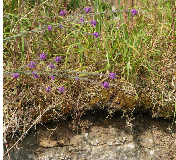
Fig. 2.16: Hugh Miller's Cottage, Cromarty, Ross-shire (CS20). The thick mossy capping has a high capacity to absorb rainfall, while its projection of up to 50mm beyond the wall face effectively casts runoff clear.
