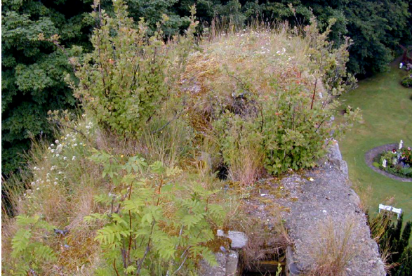
Fig. 2.8: Drumlin Castle, Moray. The defective hard capping has developed frequent cracks, allowing uncontrolled natural colonisation by species with damaging woody roots. A well designed soft capping could control this relationship.
