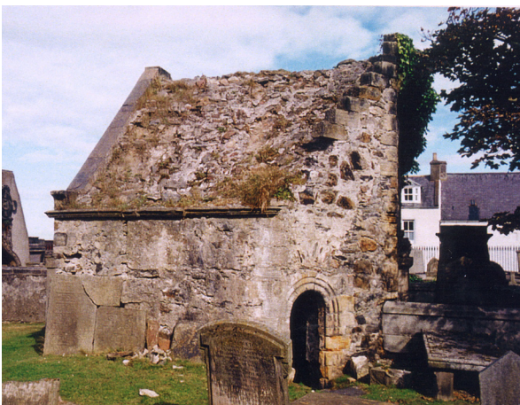
Fig. 6.4: St. Mary's Church, Banff, after removal of vegetation: fabric decay accelerated.
