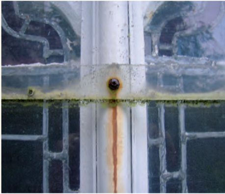
Fig. 10: This secondary glazing has become very unsightly due to corrosion from high moisture levels.
