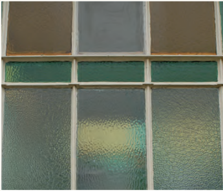
Fig. 6: Window made up of differently-aged panes, attempting to match the original pattern (likely to be the green panes at the upper middle).
