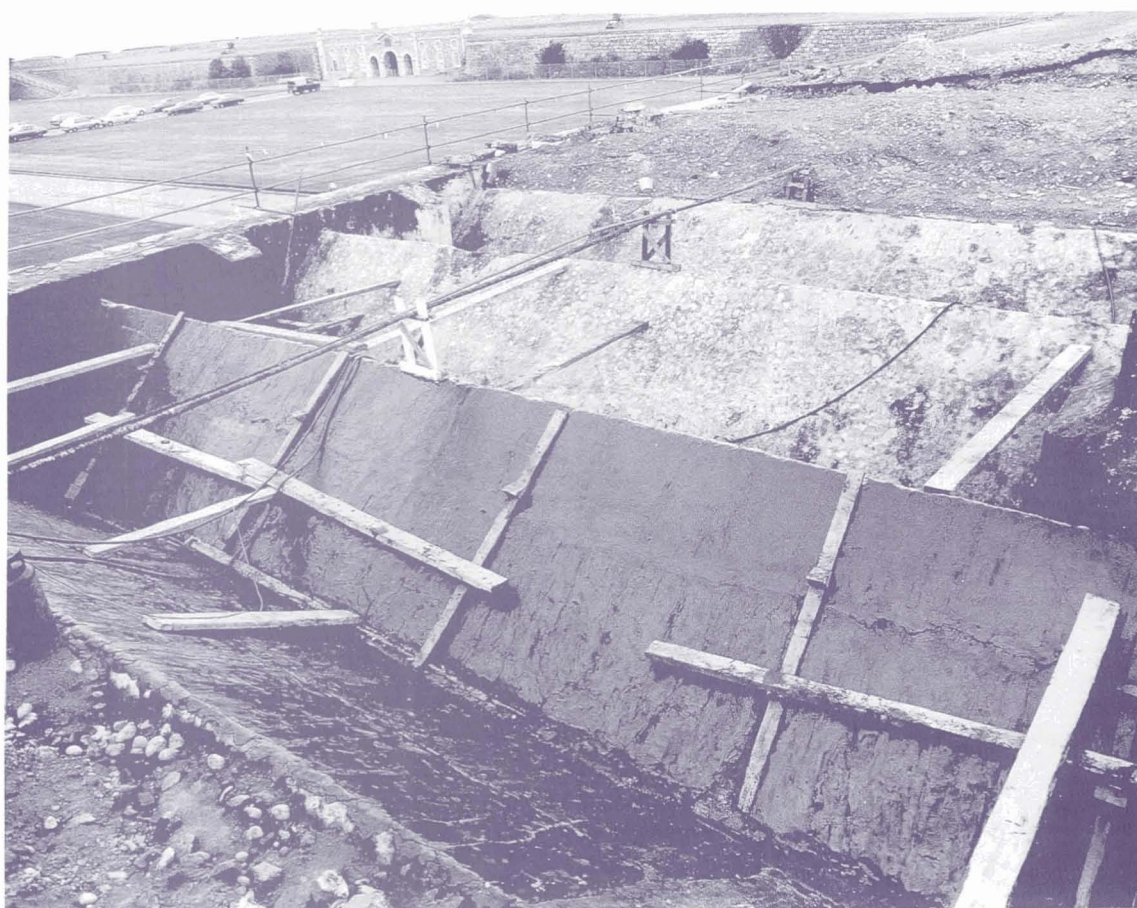
Exposed casemates in south flank wall, showing puddled clay being replaced with asphalt.
