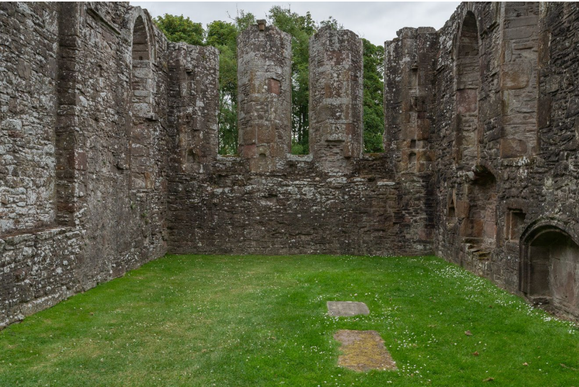
Figure 7: View of the west end of the nave showing the 3 windows unblocked © Historic Environment Scotland
