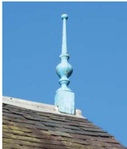
A timber finial in need of maintenance
