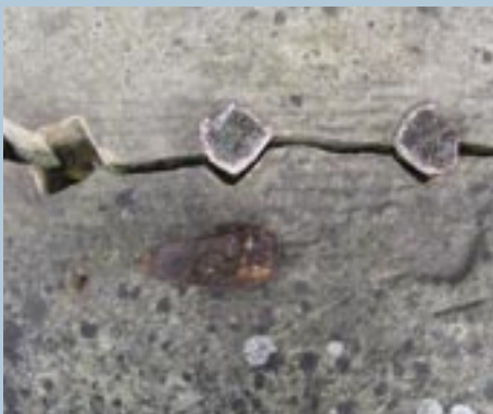
Image : Damage to masonry copes from wrought iron 'corrosion jacking' railing stubs © D S Mitchell
