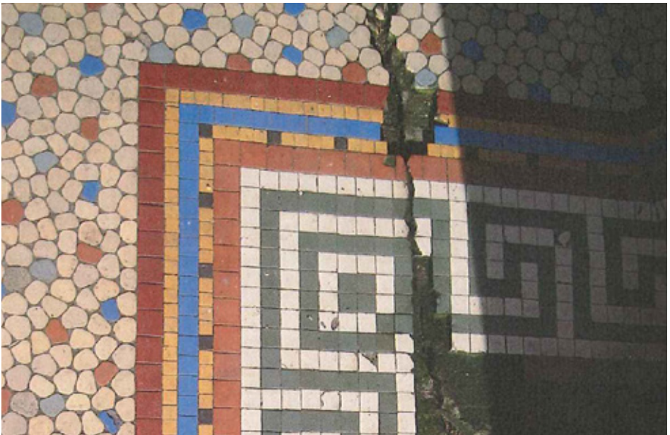
Fig. 7 Progressive loss of floor following dislodging of pieces.
