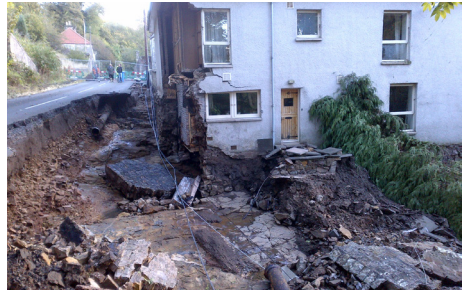
Fig. 4 Fast flowing or deep water can cause structural damage (© Paul Hendy).
