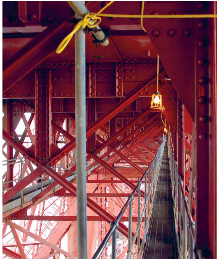
Detail of the access walkway and structural steel work beneath the permanent way in the south viaduct of the Forth Bridge, July 2011. (© Crown Copyright, reproduced courtesy of Historic Scotland. www.historic-scotland.gov.uk Miles Oglethorpe)
