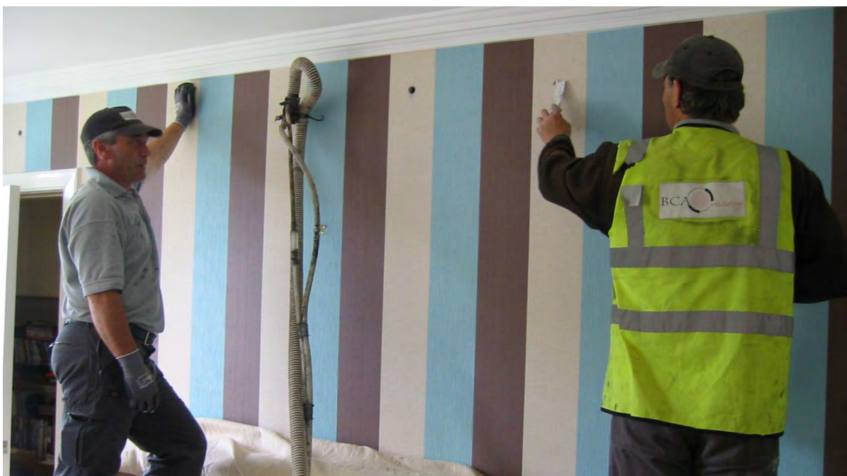
Figure 7. Filling the holes following the injection of the bonded bead. Note the bead delivery nozzle, middle left.
