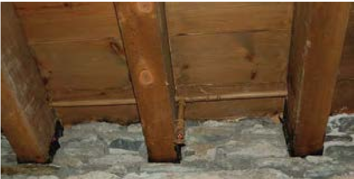
Illus 78 Sprinkler and detection heads and exposed pipework have been painted to blend in with the timber ceiling
