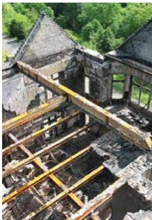
Illus 62 Large complexes of redundant institutional buildings, like this former hospital, present particular security problems. Following a wilful fire raising-related fire, although the masonry external walls remain largely undamaged, the complete loss of the roof structure left the fabric open to accelerated decay
