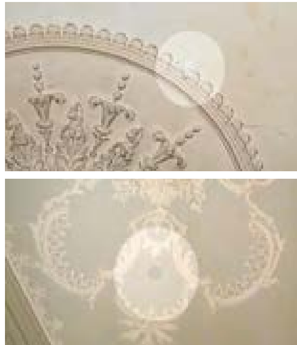
Illus 33 Two examples of discretely situated sprinkler heads in heritage properties (upper image reproduced with kind permission of the National Trust for Scotland)
