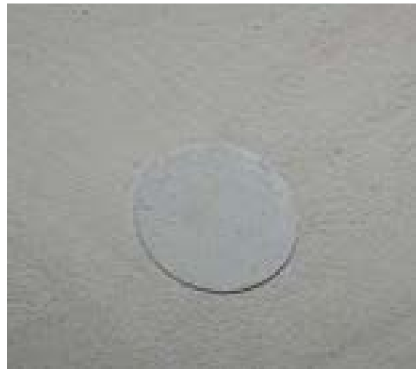
Illus 115 A limewash finish on a concealed sprinkler plate, Corgarff Castle
