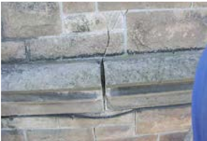
Illus 92 Bulging and cracked external masonry caused by expansion of internal metal beam
