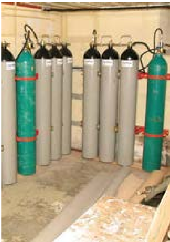
Illus 36 Water and gas filled cylinders for a water mist suppression system in a basement area © Stewart Kidd
