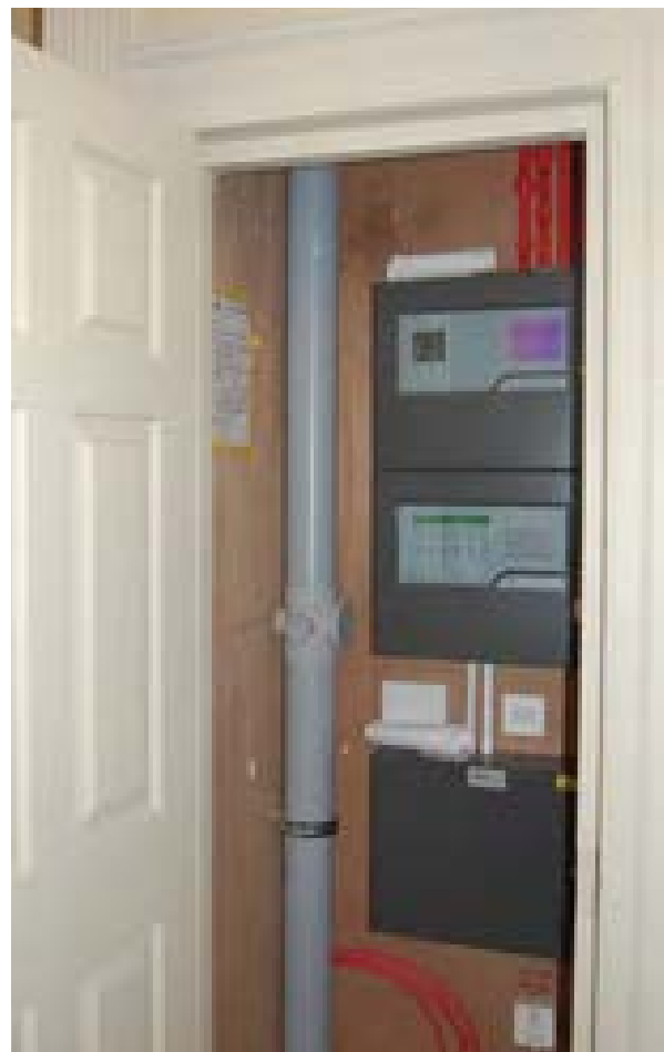
Illus 85 Sampling unit for the aspirating smoke detection system is hidden away in a hall cupboard
