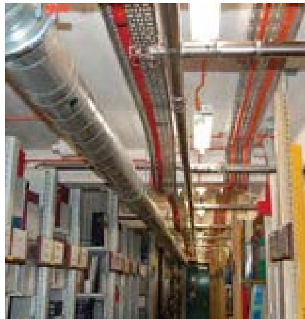
Illus 73 Sprinkler pipes running through the book storage areas (due to the low ceilings, note the protective cages over the sprinkler heads)
