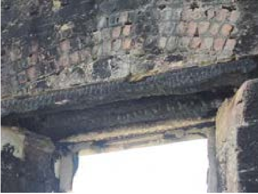
Illus 93 Fire damaged timber safe lintels with masonry arch over
