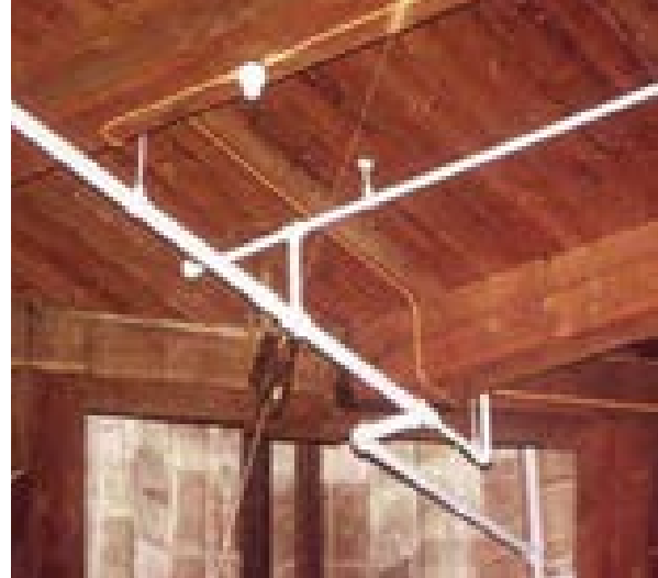
Illus 98 In this out of view attic space, the pipework has been suspended from the ceiling timbers, so minimising impact on the fabric
