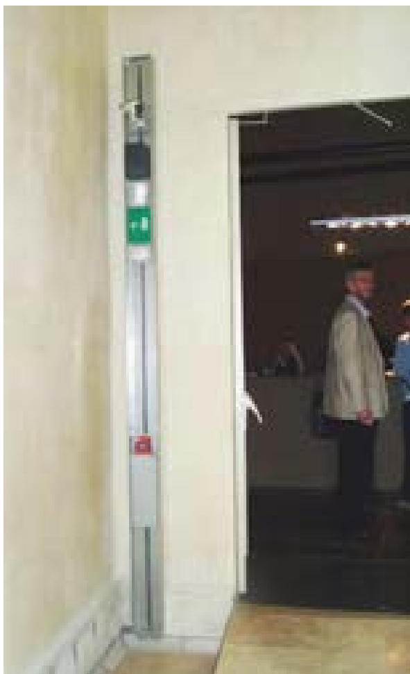
Illus 41 This totem pole is a novel solution – incorporating an exit sign and emergency lighting in addition to video surveillance, break call glass point and audio alerter © Inval Maxwell
