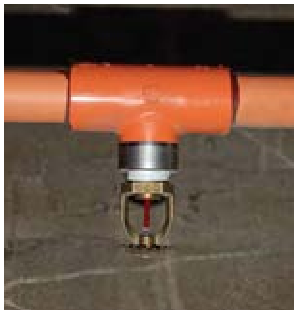
Illus 30 Chlorinated PVC plastic pipework, a possible alternative to metal pipework
