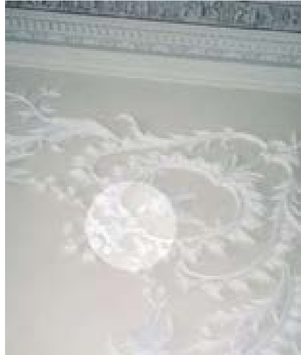
Illus 67 Concealed sprinkler head in the ornate plasterwork in the vestibule ceiling (circle beside the bird's beak) © Ingvál Maxwell
