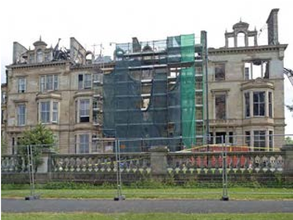
Illus 2 This Category A listed terrace in Glasgow was severely damaged by fire during sub-division into luxury flats
