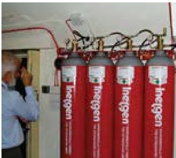
Illus 37 A gas suppression system with high pressure gas filled cylinders © Stewart Kidd
