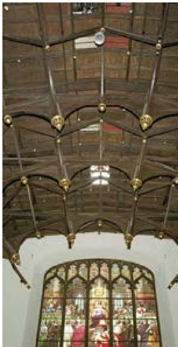
Illus 26 Parliament House in Edinburgh installed sprinklers, with pipework painted black to blend in with the elaborate ceiling © Crown Copyright: RCAHMS. Licensor www.rcahms.gov.uk
