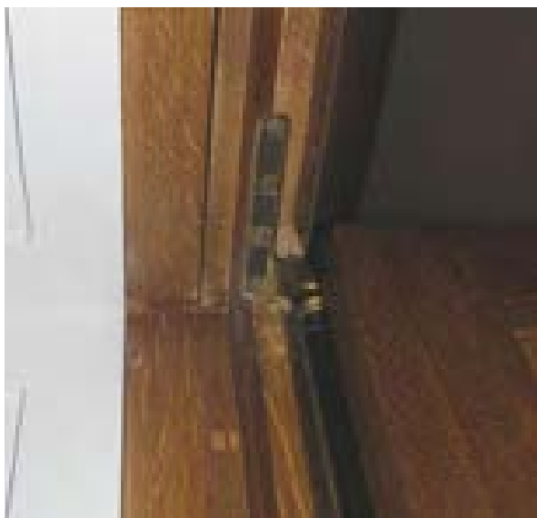
Illus 13 Intumescent products are increasingly available in a range of colours. The timber laminate intumescent strips (the dark band that goes round the door hinge) seen here match the surrounding timber
