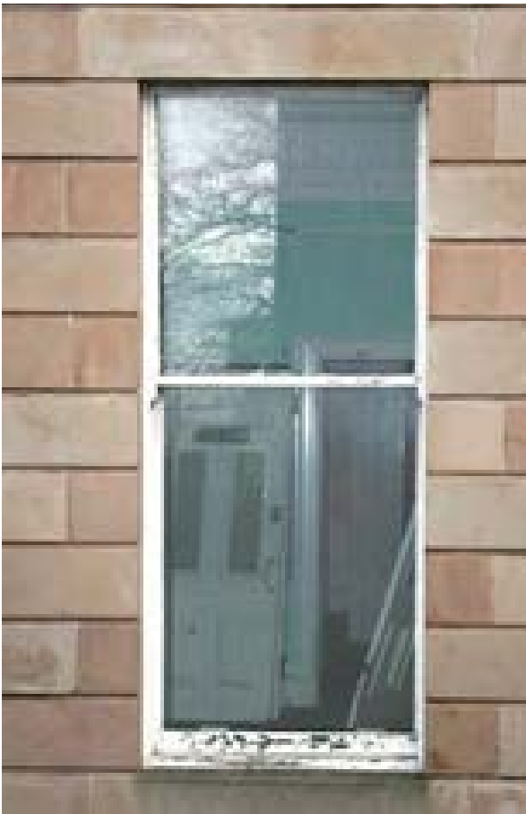
Illus 4 Part of this listed terrace was badly affected by fire during refurbishment work and the spread of the fire was facilitated by the earlier removal of the doors
