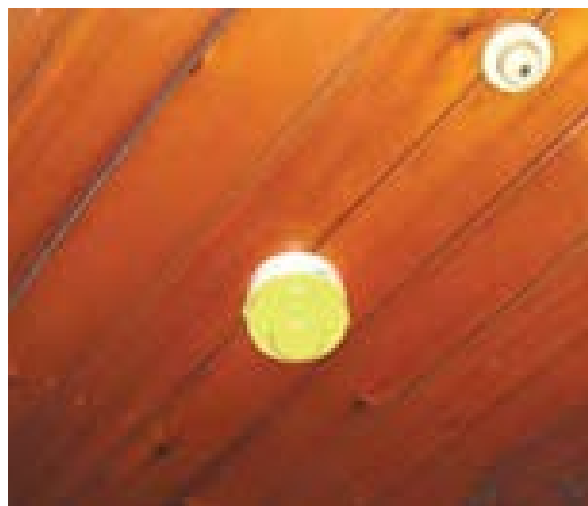
Illus 5 If detector heads are covered during works, or systems switched off, compensatory measures must be implemented during work hours. Temporary covers should be removed at the end of the working day © Stewart Kidd
