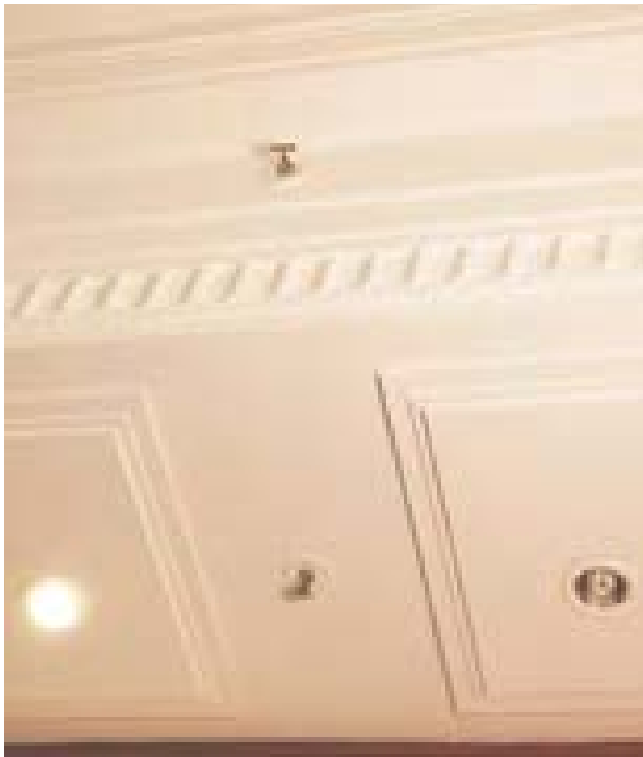
Illus 32 In any given installation, there may be a number of different types of sprinkler head installed, as here in one of the reading rooms at the National Library of Scotland
