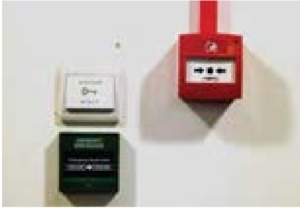
Illus 19 This is an example of bad design where the break glass call point and electric door release are too closely located
