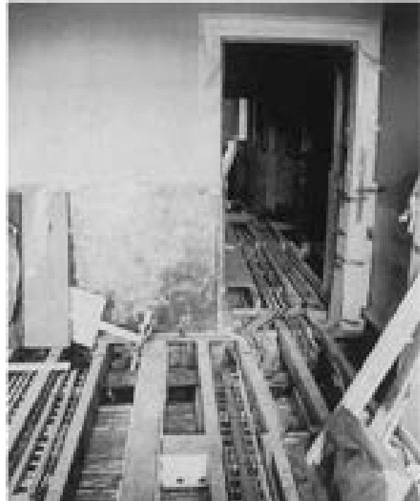
Illus 100 The timber floor has been lifted to allow the integration of horizontal service ways
