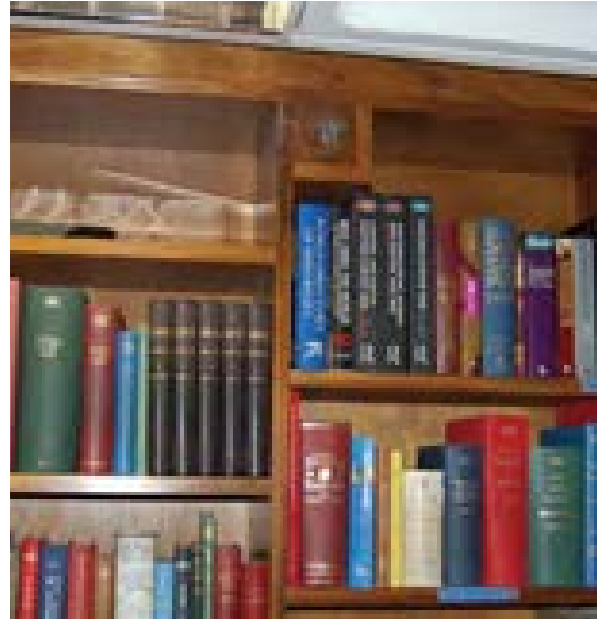
Illus 69 Sprinkler head discreetly integrated into bookshelves in one of the public reference rooms (located towards the top of the bookcase to the centre)
