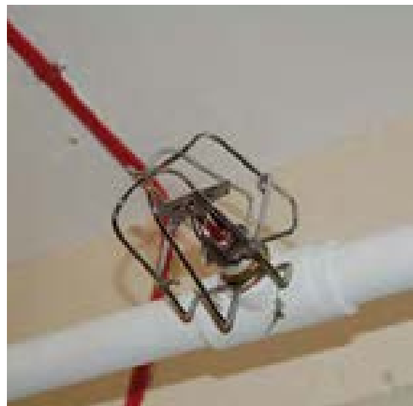
Illus 116 Protective grill placed over sprinkler heads in the low-ceiling book storage areas in the National Library of Scotland
