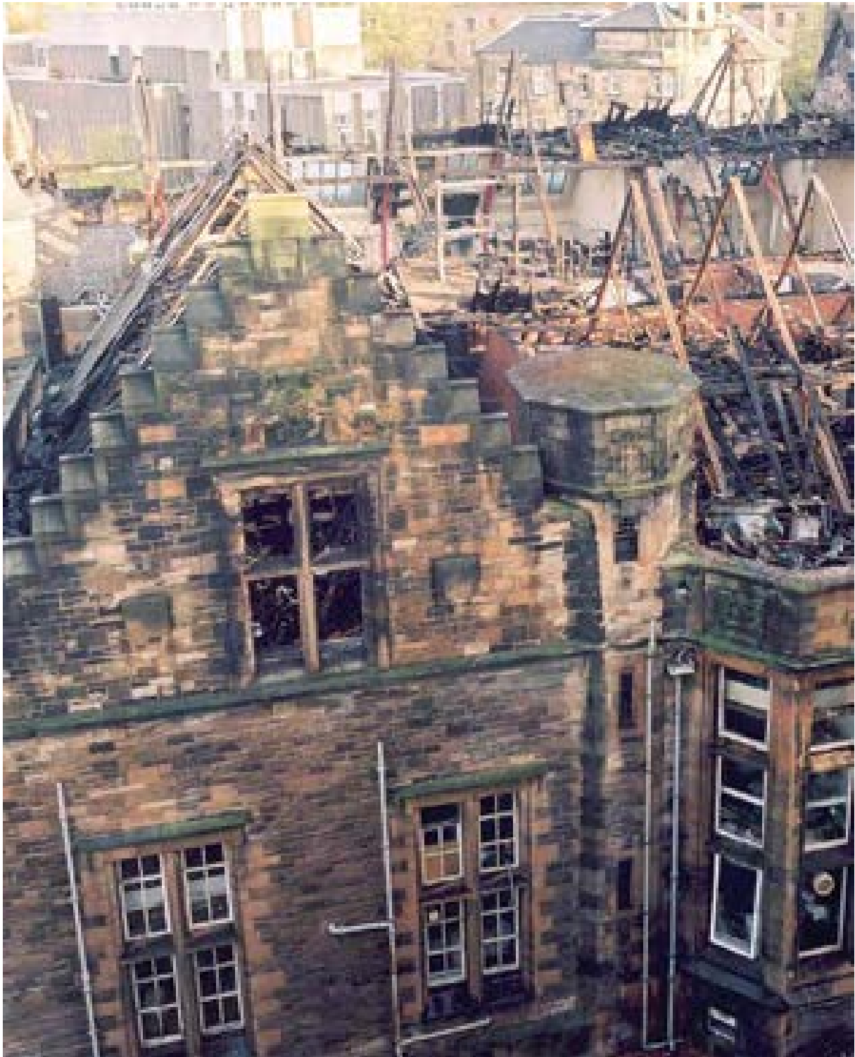
Illus 7 The Bower building, University of Glasgow. Severe fire damage to the roof and interior of this category A listed teaching and laboratory building © Crown Copyright: RCAHMS. Licensor www.rcahms.gov.uk
