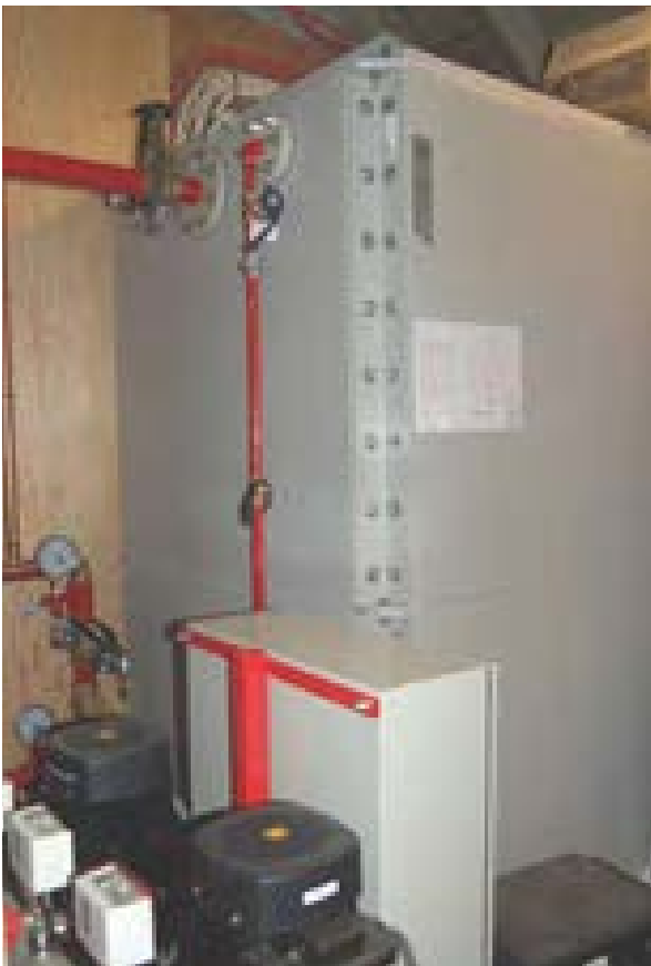
Illus 76 Water tank and pumps – the tank was assembled in situ
