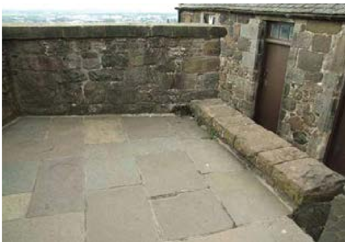
Illus 9 A thermographic survey at Stirling Castle kitchen block unearths a redundant chimney flue at parapet level
