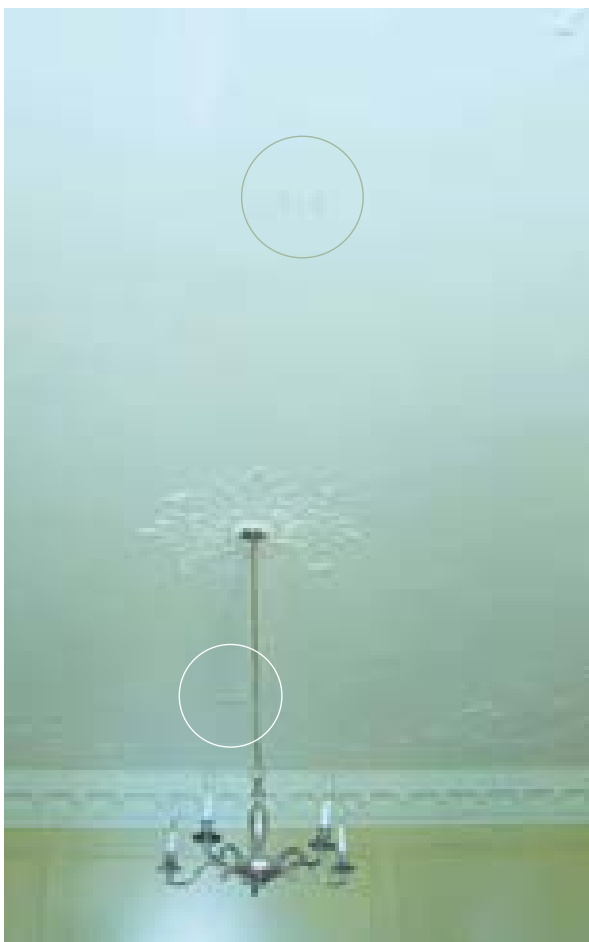
Illus 83 The highlighted areas show that concealed sprinkler heads do not detract from the delicate ceiling plasterwork
