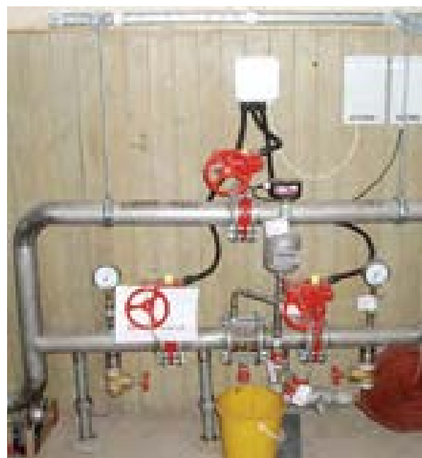
Illus 29 An example of a main stop valve for a sprinkler system, located out of sight in a basement area
