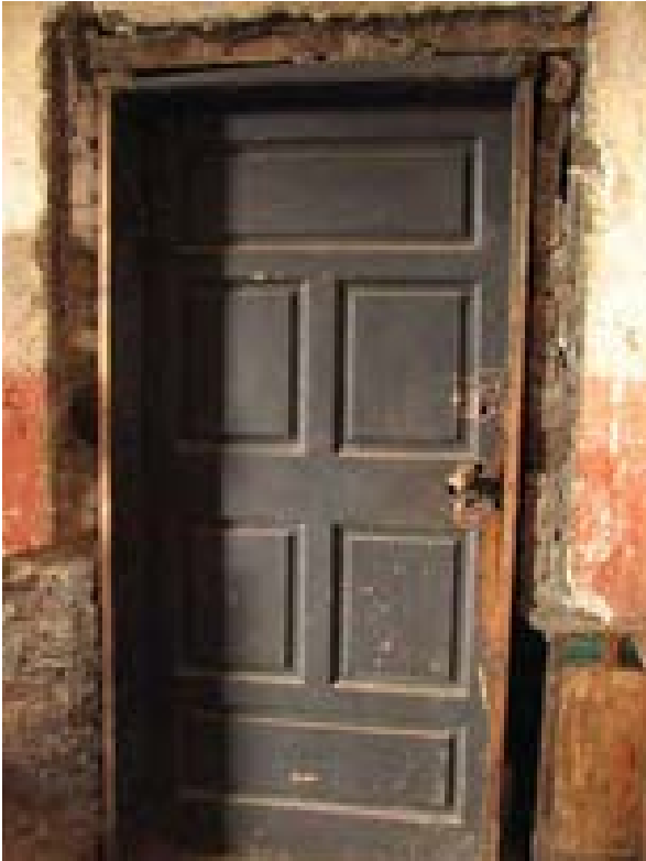
Illus 12 This image from a property undergoing refurbishment clearly shows the sizable gaps that can exist between a door frame and the supporting wall
