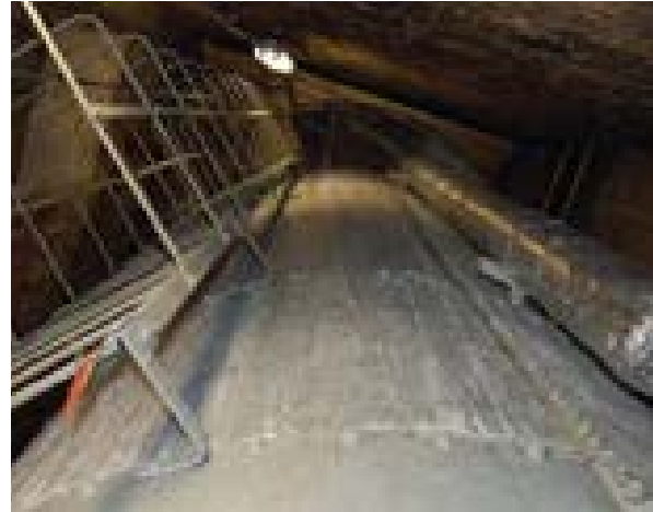
Illus 27 To satisfy the required volume of water for the sprinklers in the National Library of Scotland, two purpose built water tanks were constructed and housed in the historic vaults below the street
