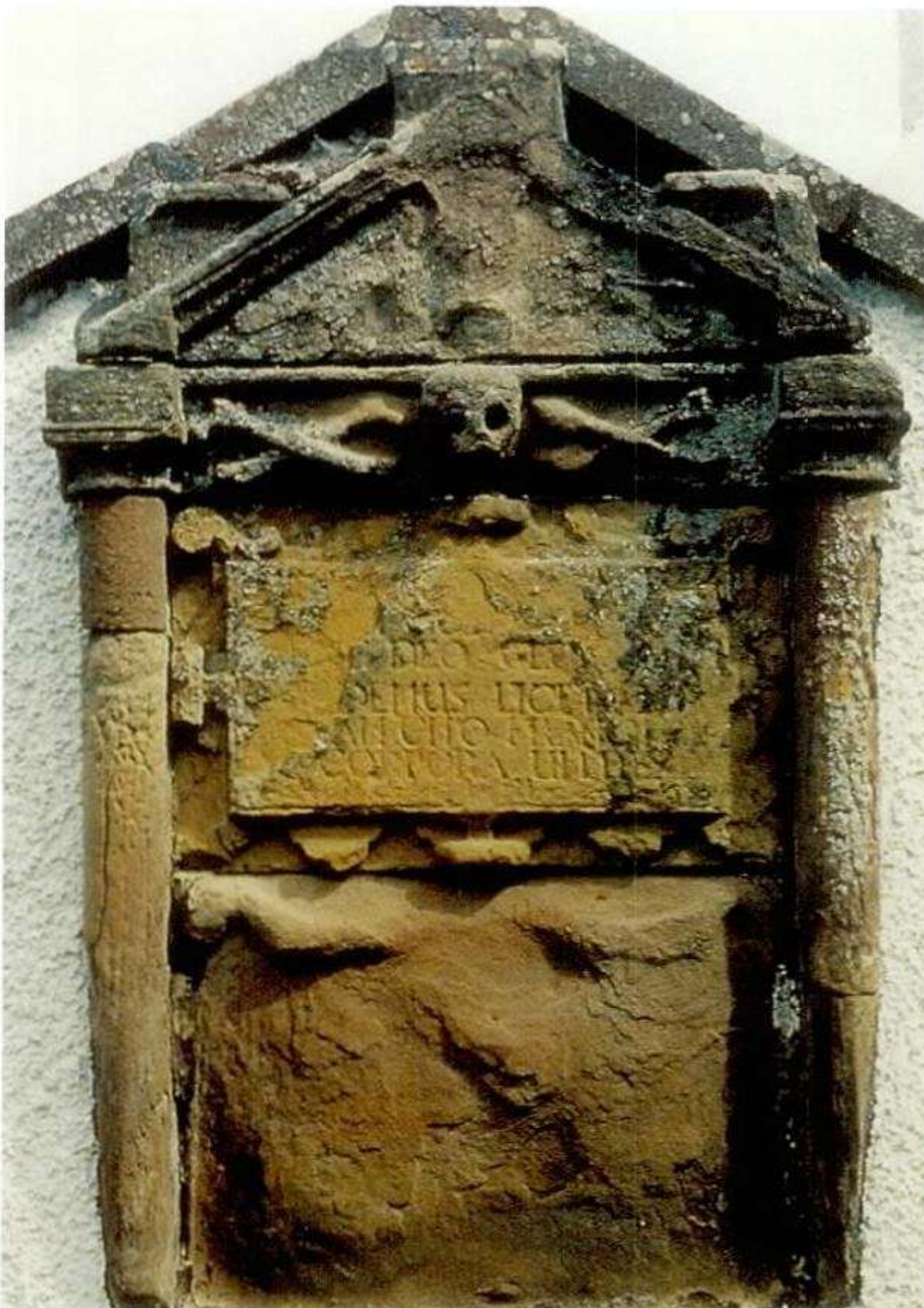
Illus 2 Sandstone wall monument at Cromarty East Church that is now in an advanced state of decay
