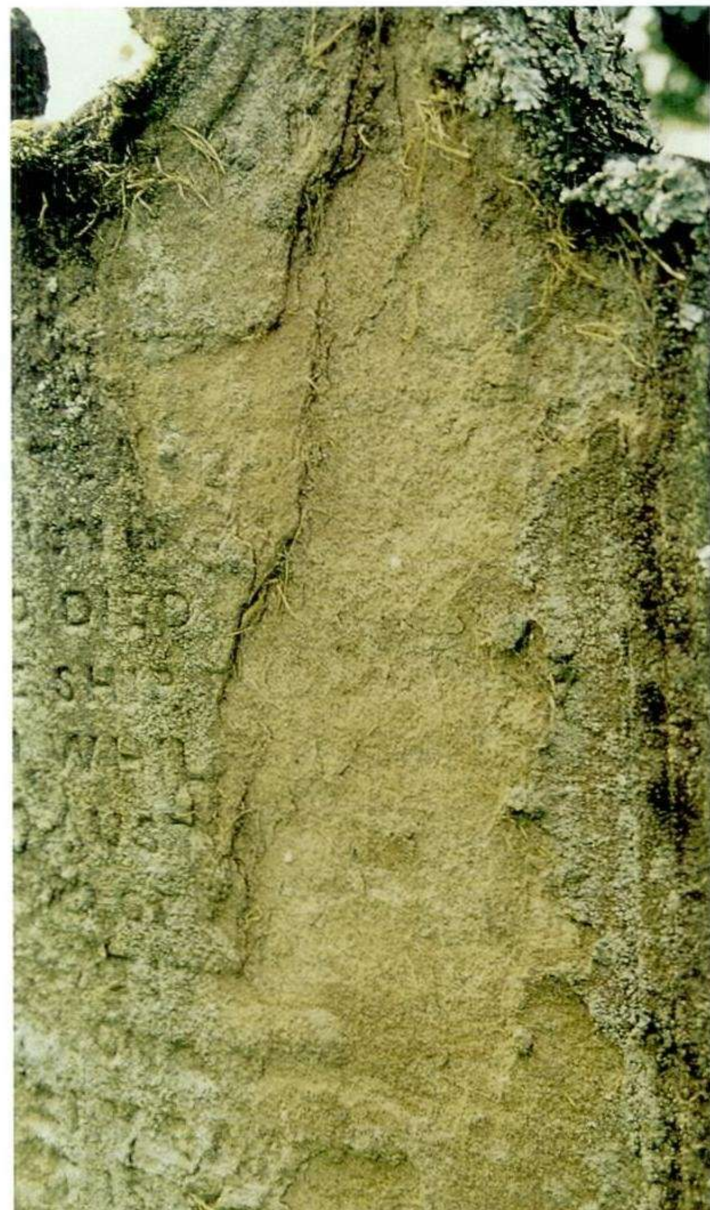
Illus 4 Moss roots contributing to the delamination of a sandstone headstone
