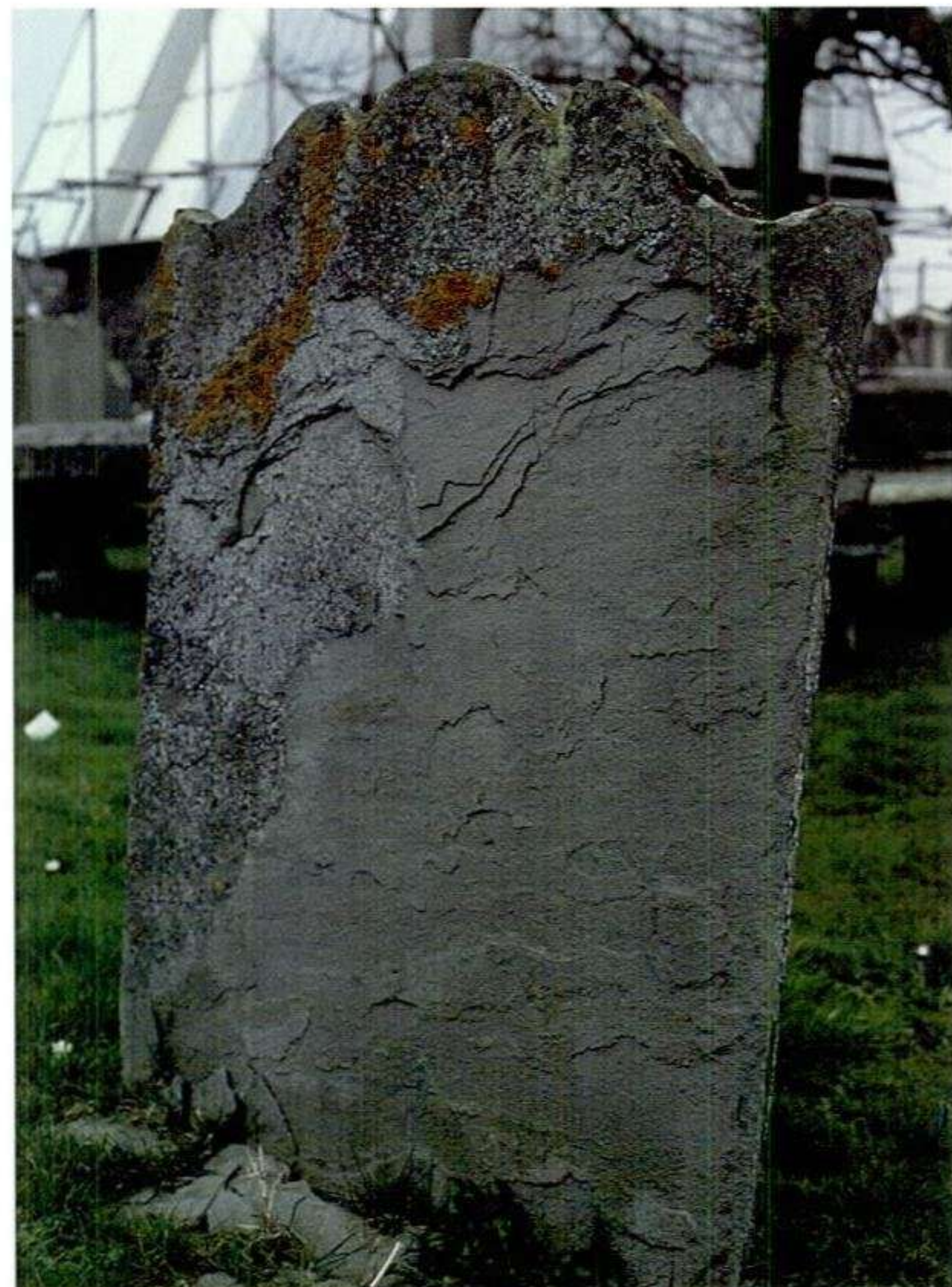
Illus 2 The inscription on this headstone has been completely lost as a result of delamination of the stone
