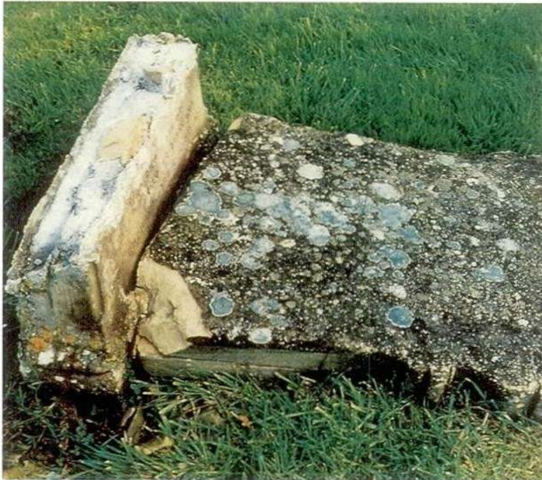
Illus 5 A failed cement mortar repair has increased the damage to this headstone
