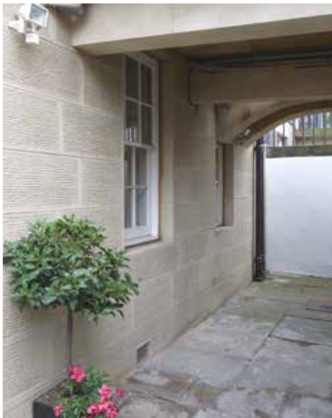
Fig. 13 The extensive use of restoration mortars for an entire building façade is not recommended.
