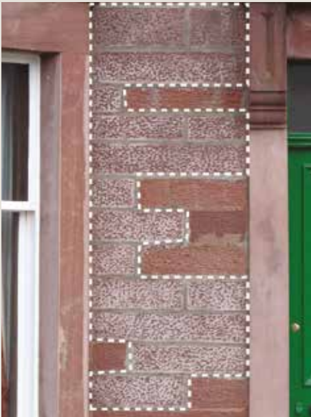
Fig. 11 Overworking the repair surface (highlighted by dashed lines) results in a light, patchy appearance.
