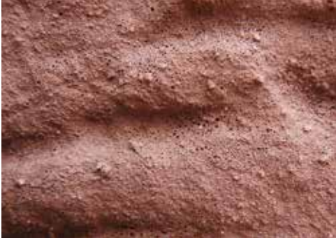
Fig. 5 Over mixing or addition of excess water can create a 'foamy' texture in restoration mortars.
