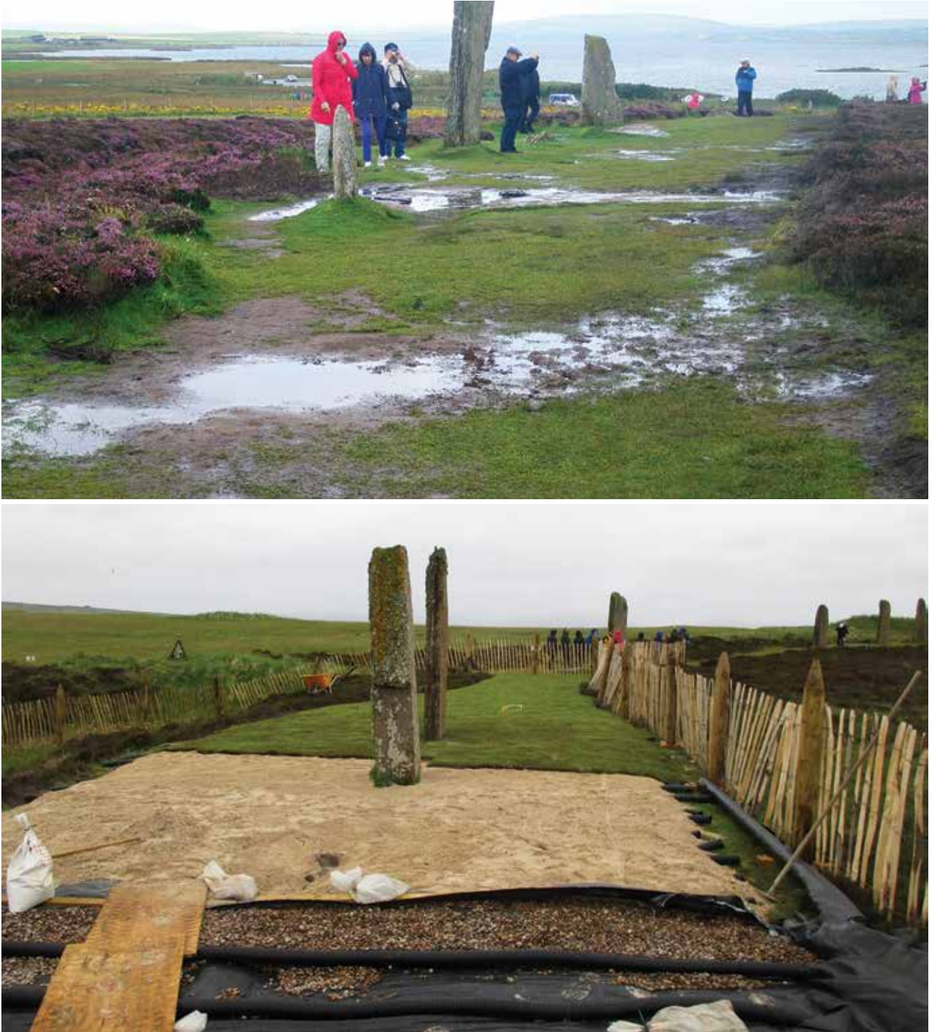
Figure 2.9 Examples of management pressures and conservation actions at HONO sites: Damage to footpath at Ring of Brodgar resulting from higher visitor numbers and increased rainfall levels (top); Installation of engineered surfaces to improve footpath resilience (bottom).
