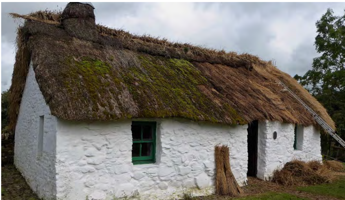
Figure 5. Cruck Cottage in 2017 prior to rethatching. The moderate decay of the thatch was likely being exacerbated by vegetation growth. Image courtesy Cruck Cottage Heritage Association.
