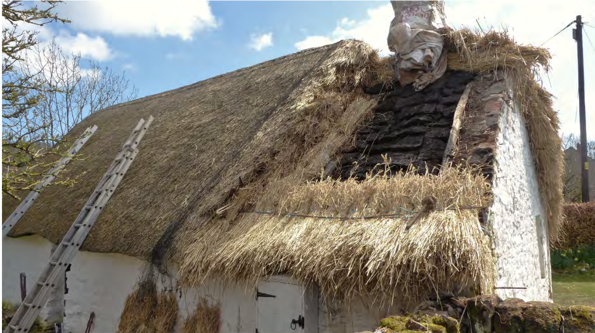
Figure 13. Layers of the 2018 thatch repair. Turves have been laid like tiles, and the bottom row of thatch bundles has been fixed down with steel rod sways, stitched through the underlay with wire. Image courtesy Cruck Cottage Heritage Association.
