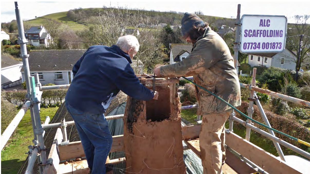
Figure 11. Clay daubing being laid over the repaired timber frame. Image courtesy Cruck Cottage Heritage Association.
