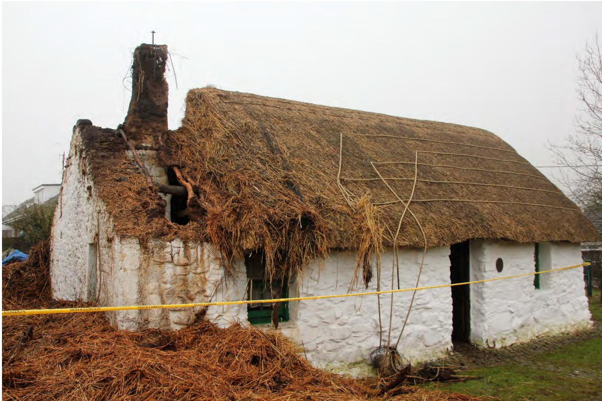
Figure 10. The damage from the 2018 fire. A great deal of thatch was rendered unusable and the wooden framework of the chimney was compromised, but the roof frame and historic crucks were essentially undamaged. Image courtesy Cruck Cottage Heritage Association.
