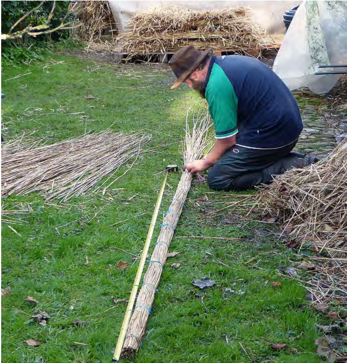
Figure 8. Long straw 'dollies' were added underneath the thatch at the ridge to raise the apex.
