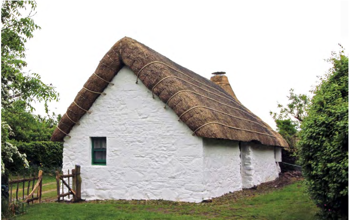
Figure 9. The east gable following the 2017 rethatch, showing the rolled overhang and rope fasteners. The 'eyebrow' profile over the back door is also visible. Image courtesy Cruck Cottage Heritage Association.
