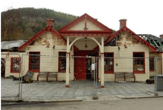
Fire Damage at Ballater Railway Station
