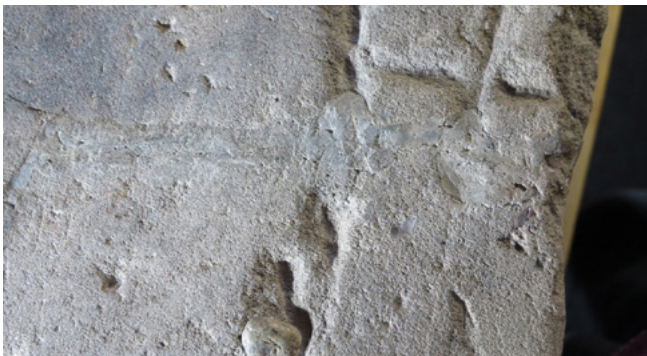
Fig 16. Close-up of the area with visible fibrous material within the cementitious repair (2023).
