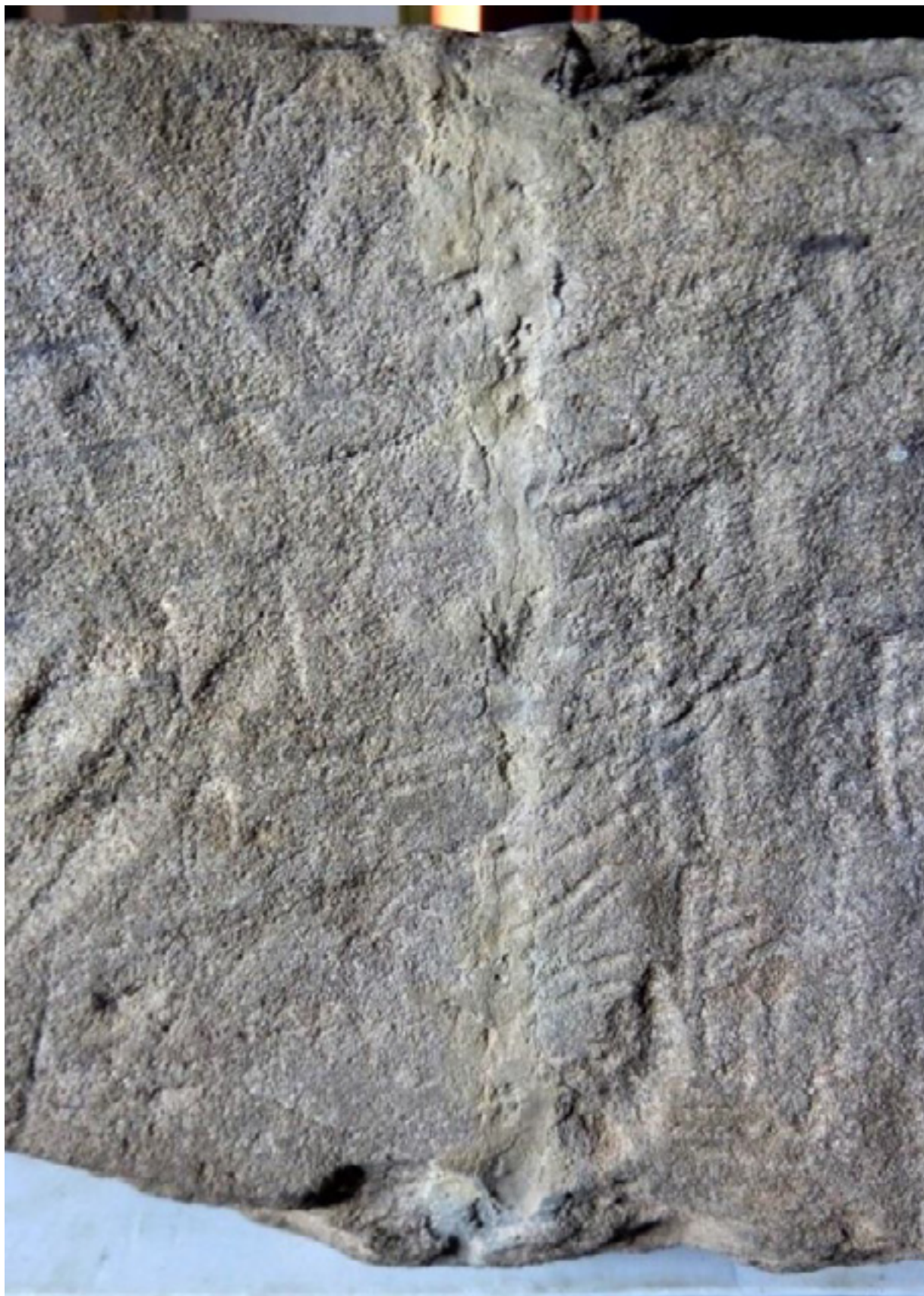
Fig 23. Condition of the joint over the repair (2016).
