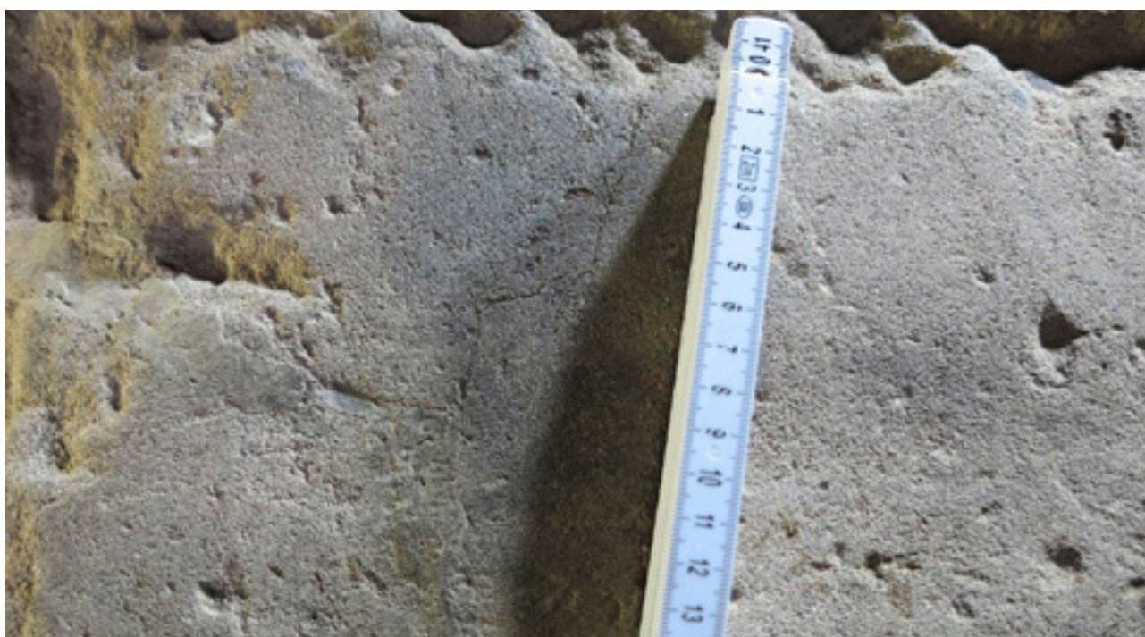
Fig 14. Close-up of a hairline fissure (2023).
