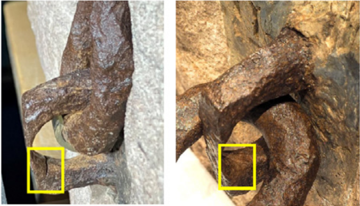
Fig 55. The cracked staple before (left) and after (right) application of the fill.
