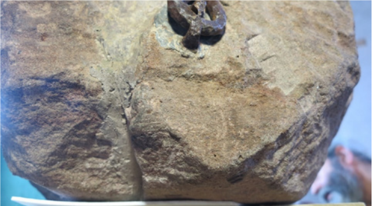
Fig 53. The same area shown in Fig 52 after injection and filling with acrylic resin mortar repairs.
