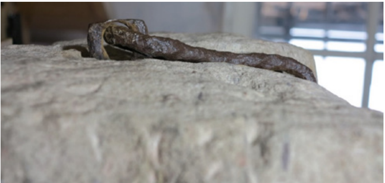
Fig 51. Close-up of the dexter face showing the fragility of the ironwork and its vulnerability to mechanical damage (2023).
