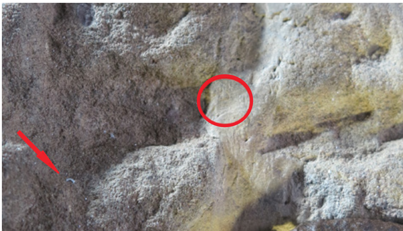
Fig 15. The circled area (top) shows a repair joint with visible fibrous material incorporated into mortar (2023). The area indicated by an arrow (left) shows visible white flecks of a silicone-like substance deposited on the stone surface.
