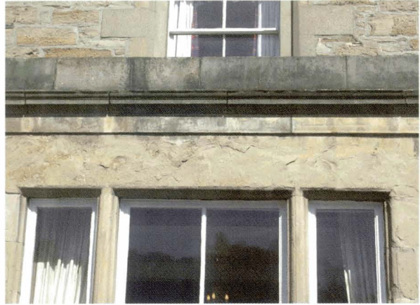
j) Multiple scaling: Surface scaling of lintel. No immediate structural problem.
