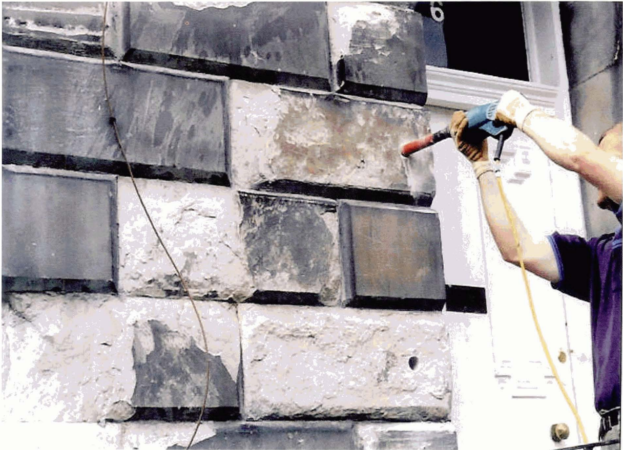
Fig 14 Diamond core drilling to extract small-diameter plug of stone from damaged masonry (Photo: BGS©NERC)
