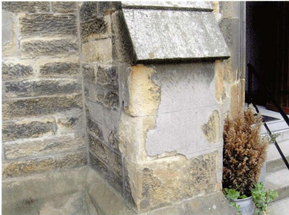
h) Cement mortar patch; in this case the stone decay is minimal behind the patch.
