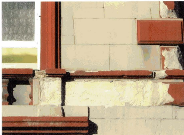
c) Loss of stone surface. Primary cause is difficult to determine but the facade has been cement plastered and painted resulting in entrapped moisture. Maintenance will be required on this facade to remove the cement plaster within the next twenty years. Classification: Immediate replacement of decayed stone and maintenance of plastered areas within twenty years
