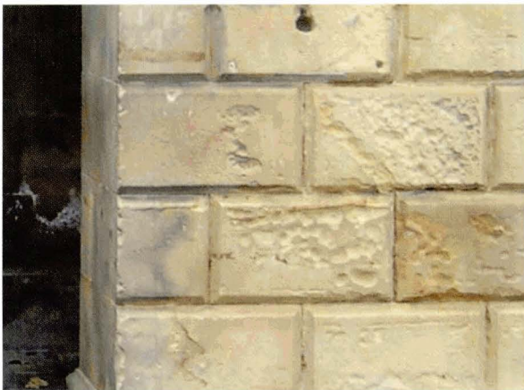
i) Differential decay. Natural weathering of stone on 200 year old facade.
