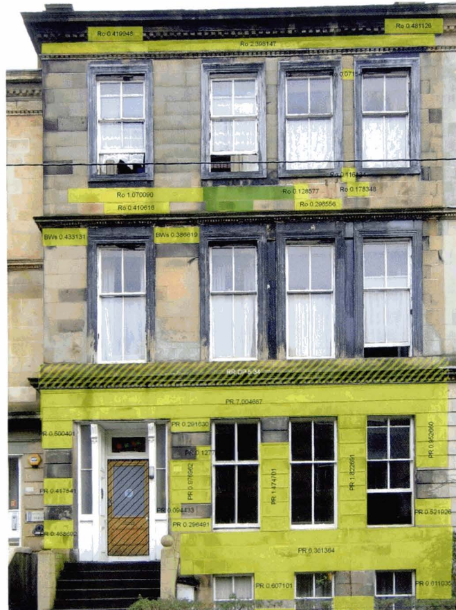
Figure 2. Examples of the results of facade surveys with stone decay identified by a colour coding system (Photos: BGS©NERC)
