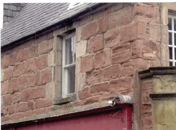
l) Squared rubble (clay-rich sandstone) has suffered long-term granulation, possibly aggravated by salt action due to coastal location. While a lot of surface has been lost the stone remains structurally sound.
