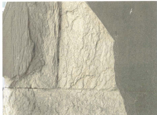
e) Flaking: Pre-existing decay accelerated by a covering of cement mortar plastic repair. Classification: Immediate replacement
