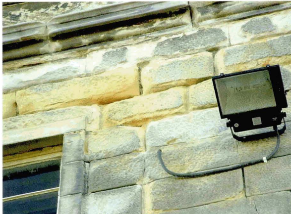
b) Crust plus granulation: Edge erosion: similar action to illustration a) and decay is accelerated by loss of pointing in both the drip moulding, and in the stonework generally, and/or use of hard mortar. Classification: Immediate replacement
