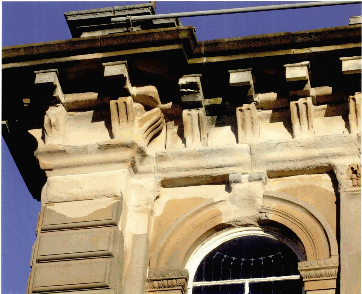
Figure 6. An extreme example of sandstone decay promoted by chemical stone cleaning. Falling masonry is now a risk on this building (Photo: D Urquhart)
