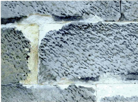
a) Surface crust formed (tooling on surface is still intact) but the loss of sandstone cement from the grains below the surface has led to granular disaggregation in the surface zone for more than 20 mm depth. Classification: Immediate replacement
