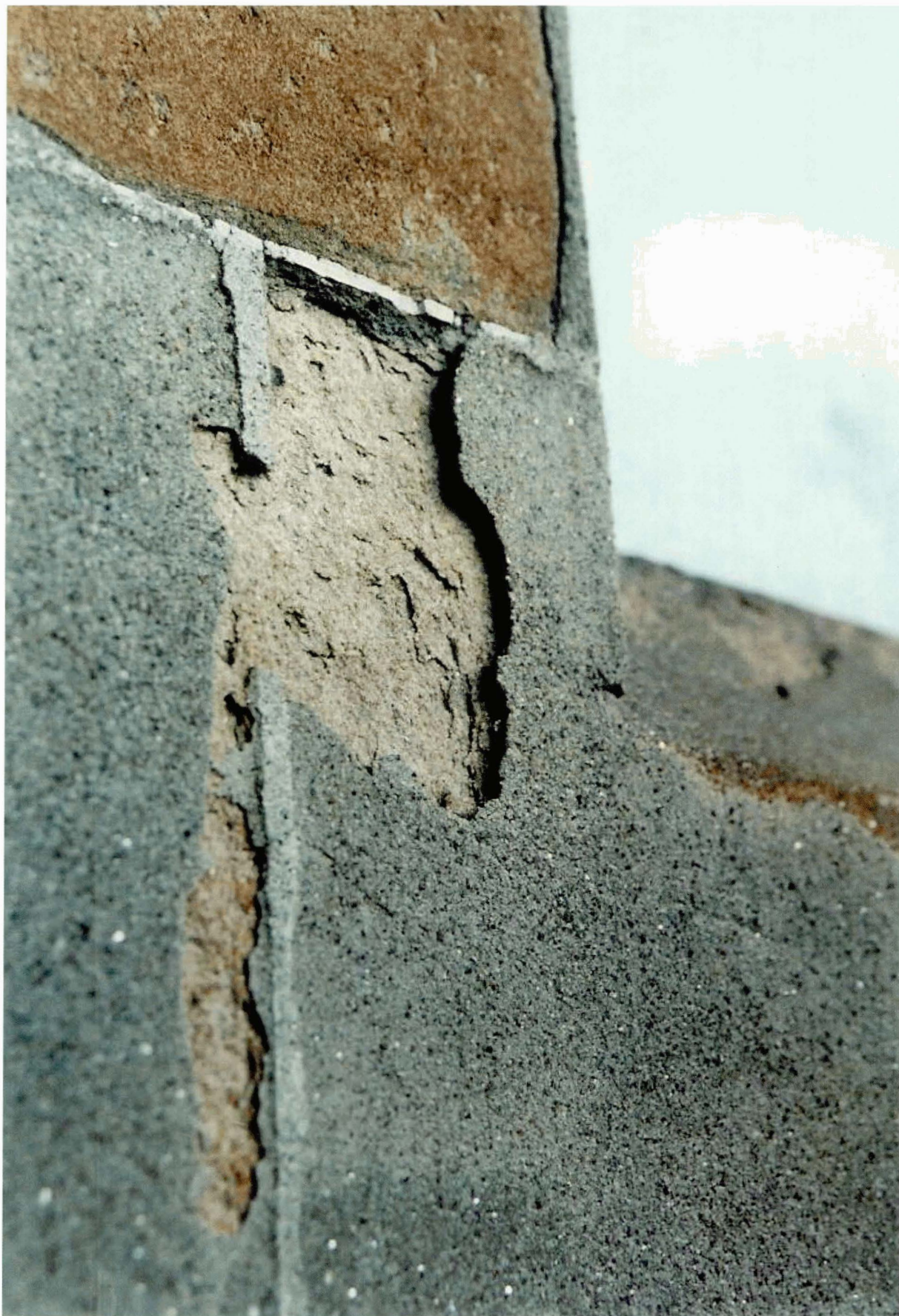
Figure 7. Typical example of plastic repair causing damage to the underlying sandstone (Photo: D Urquhart)
