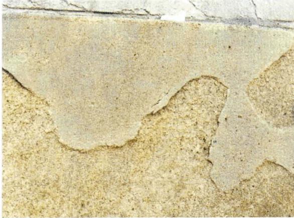
g) Contour scaling on ashlar – large sheets several millimetres in thickness.
