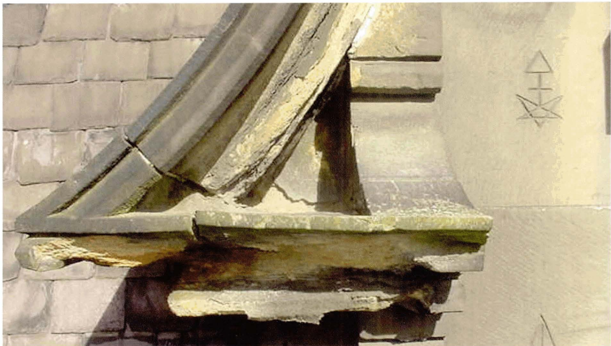
Figure 3. Decayed cornice presenting a risk of falling masonry (Photo: Edinburgh City Council)
