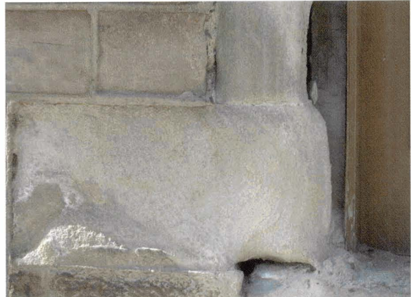
d) Granulation: Serious loss of binding cement in the blonde sandstone. Possibly associated with salt action and hard pointing. Classification: Immediate replacement
