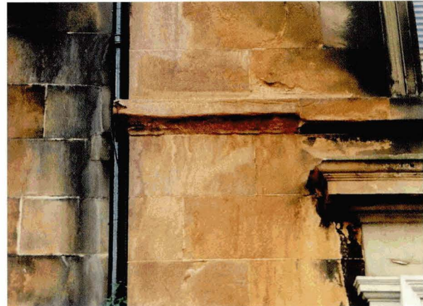
f) Partial loss of stone from drip moulding leading to surface runs of rainwater but some function still retained. Classification: Replacement within twenty years
