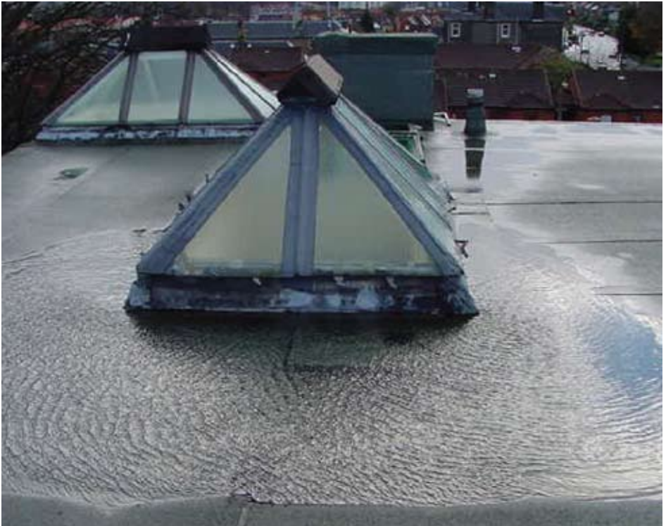
Pooling water around a roof light will lead to major deterioration of both the roof light and the flat roof
