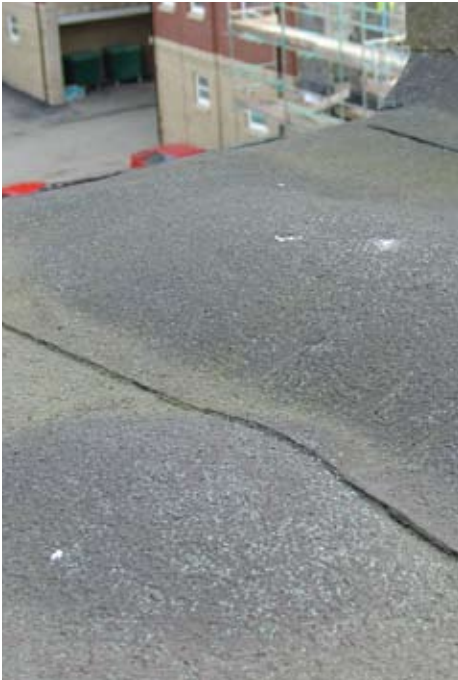
Blistering of roof felt
