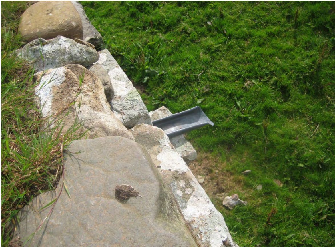
Figure 8. The new lead spout inserted in the existing stone opening to take water off the roof.
