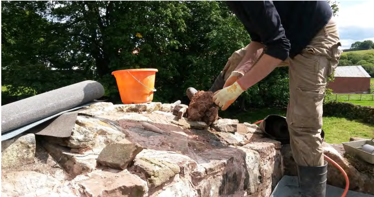
Figure 6. Re-bedding the masonry of the tower wall heads prior to the application of the soft capping.
