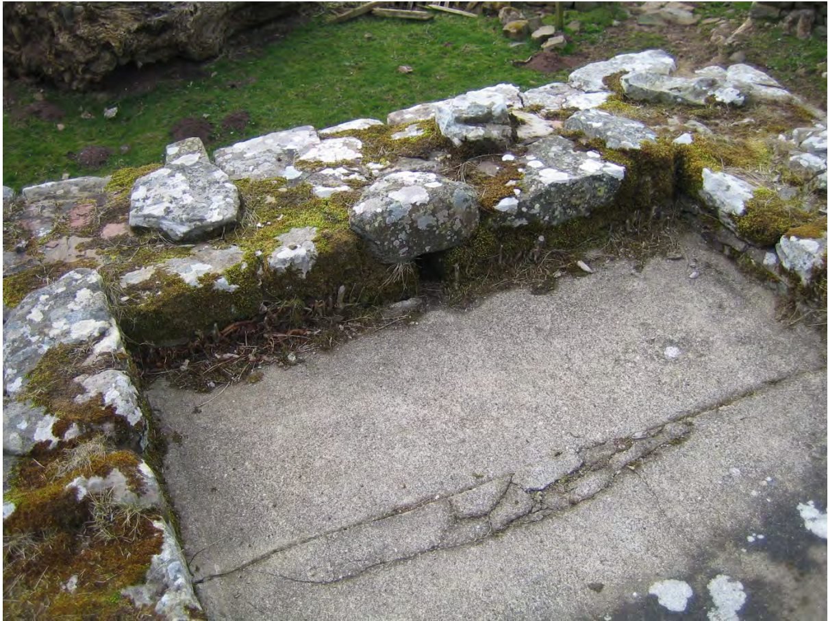
Figure 5. The roof of the tower following cleaning. The sapling stumps and the cracked concrete roof can be seen.
