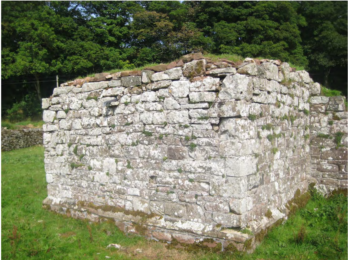
Figure 9. The tower viewed from the south west. The turf and grass of the soft capping is just visible. The grey cement pointing from earlier works is very evident on the lower courses.
