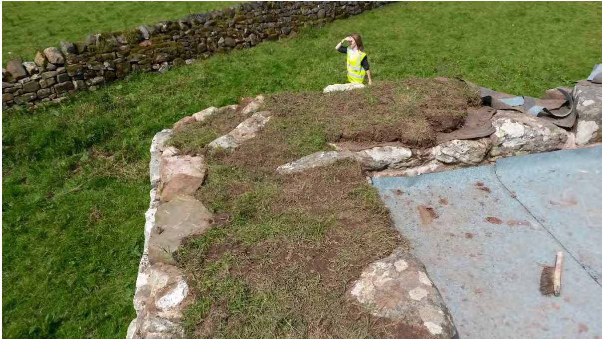
Figure 7. The new turf forming the soft capping on the tower wallheads during laying. Due to the exposed nature of the site from the southwest, the turf was edged with masonry. The application of the new mineral felt covering to the flat concrete roof is underway, seen to the right.
