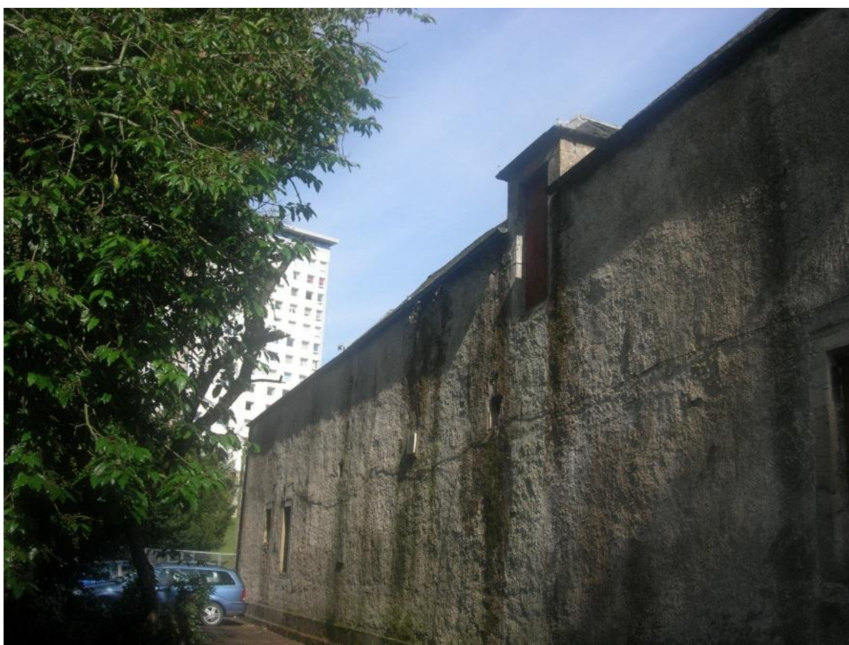
Fig. 8. Shrubs and trees were cut back to prevent physical damage and allow free air movement
