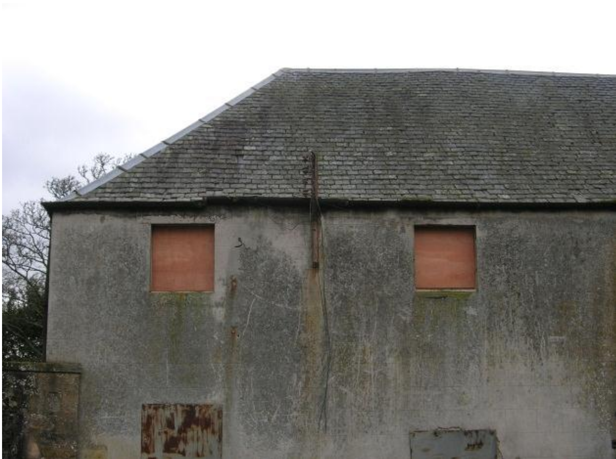
Fig. 9. Windows were boarded up to prevent re-infestation by birds and other unauthorised access
