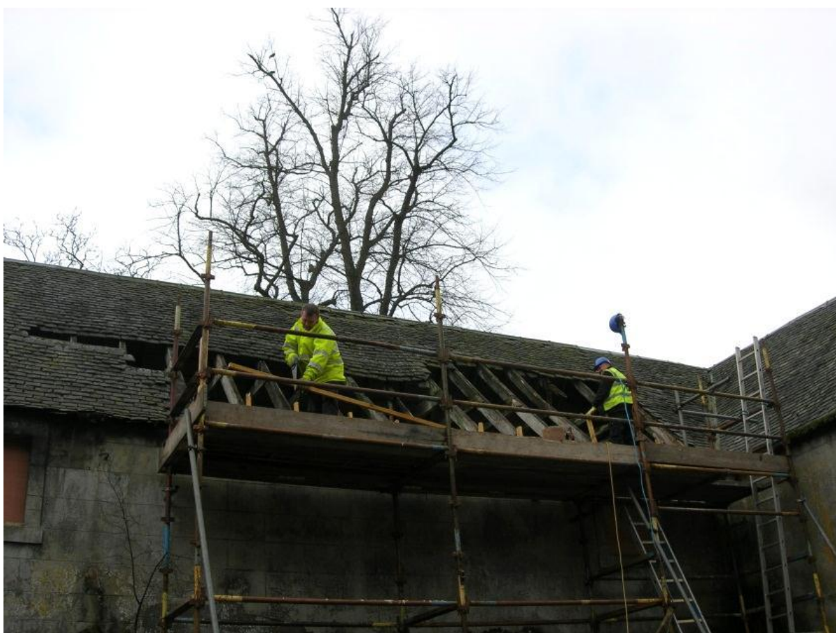
Fig. 5. The decayed section of roof being removed, in total twelve trusses required to be replaced during the interim repair measures
