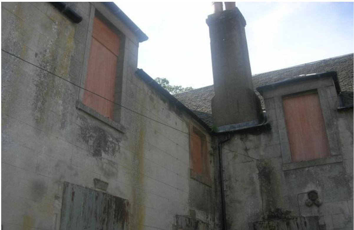
Fig. 4. Where the existing castwork was missing, new temporary plastic gutters were fitted to the courtyard elevations
