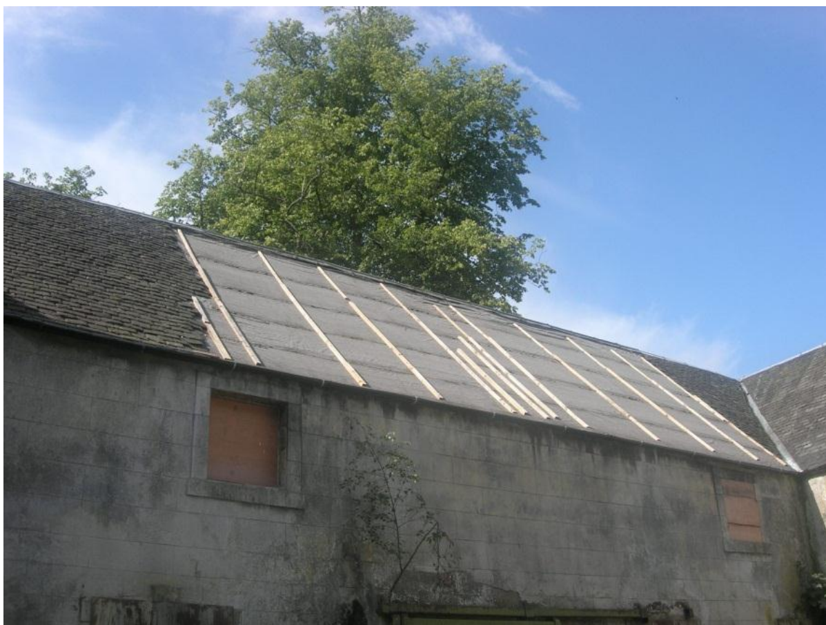
Fig. 7. The finished roof repair, showing the temporary felt covering and the battens
