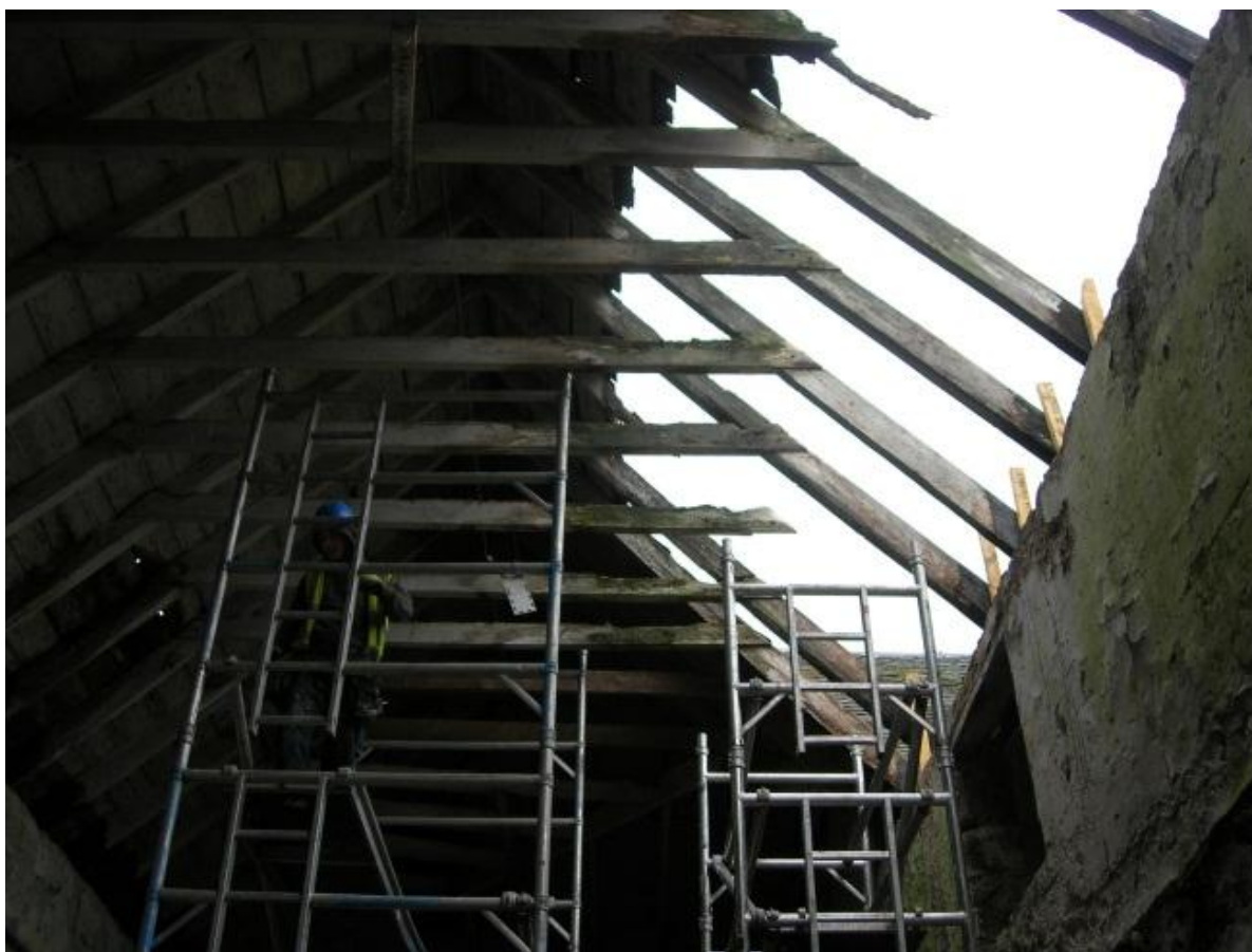
Fig. 2. Access to the damaged section of roof was via both an internal and external scaffold
