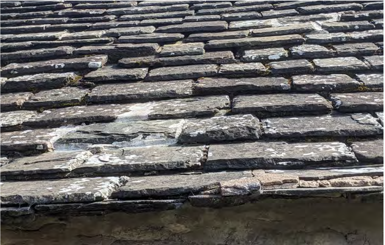
Figure 35: An example of surface pointing of flagstone slates. While this can secure a broken slate, pointing under the tail will trap water within the roof and stone, promoting moss growth and frost damage. © Sara Carruthers.
