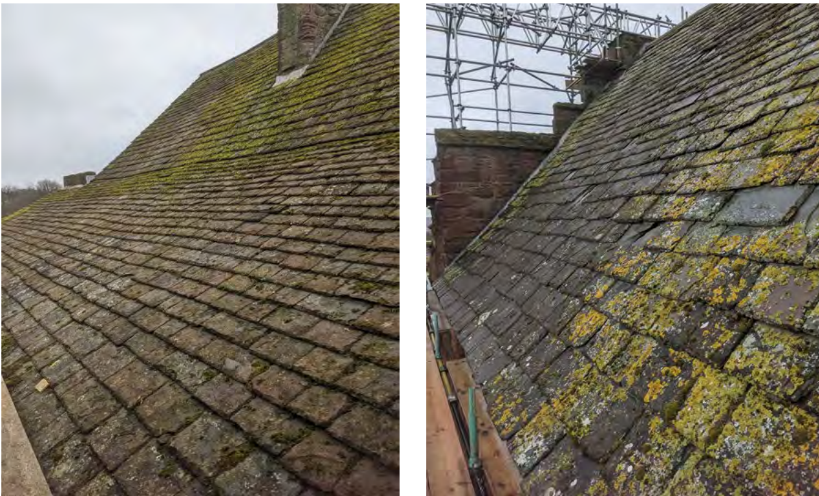
Figure 51a and b: The roof of the Abbot's House showing the north elevation (a) and south elevation, facing the sea (b). The south elevation is in poorer condition, with broken and delaminating flagstone. © Sara Carruthers.
