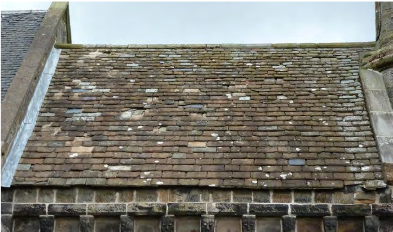
Figure 44: The south roof of the chancel at St Athernase, before repair. © Douglas Binnie.
