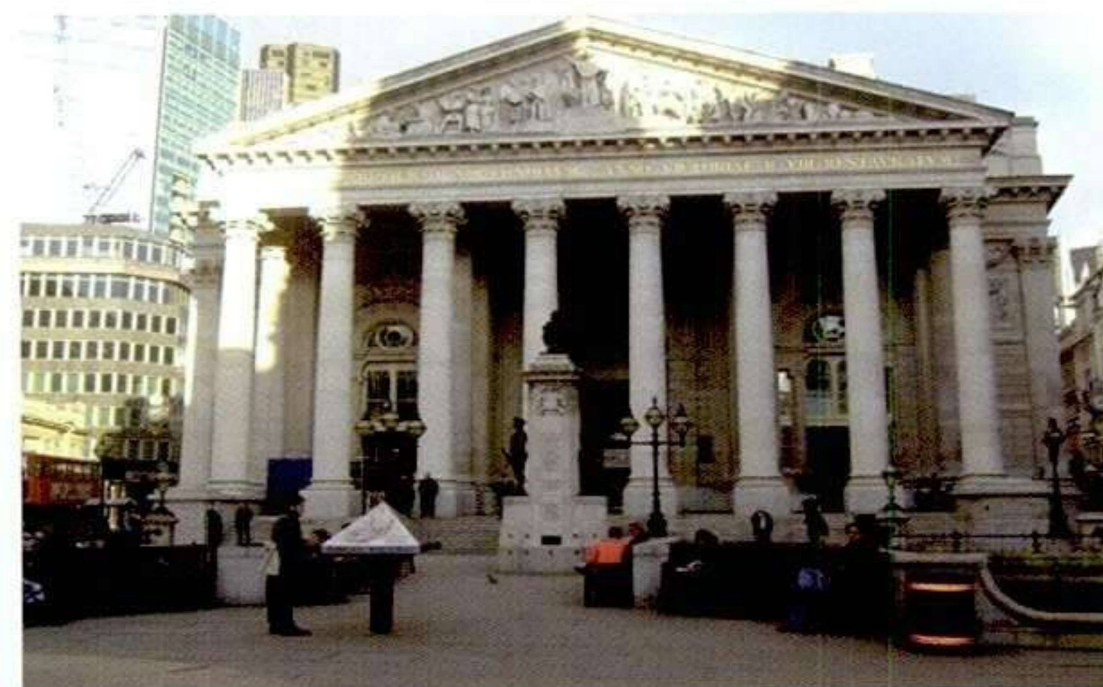
The Royal Exchange at the end of 2007, after cleaning with a combination of low volume water, steam, latex poultice and clay poultice. The stonework still holds evidence of previous abrasive cleaning.
