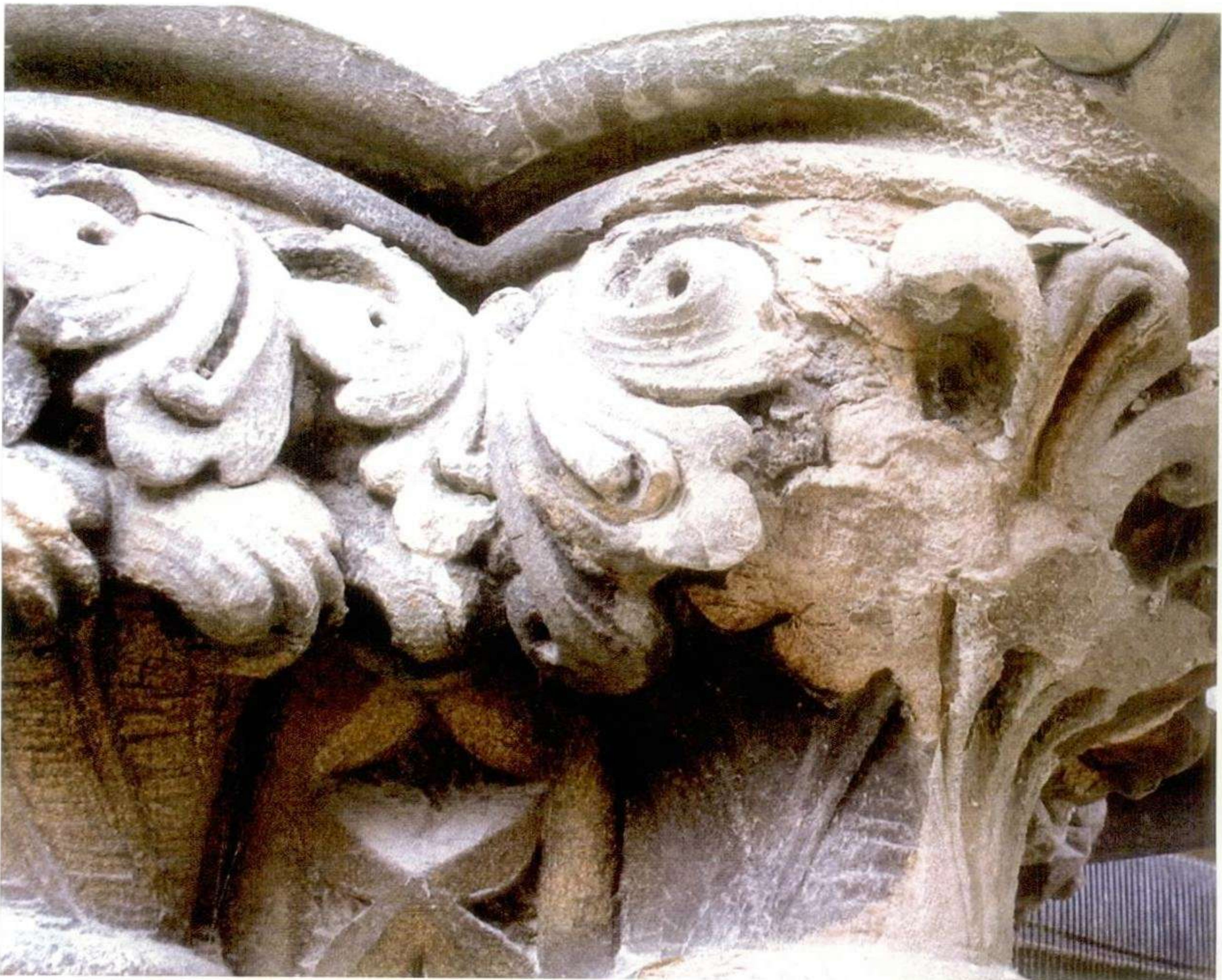
Stone erosion of a moulded capital.
