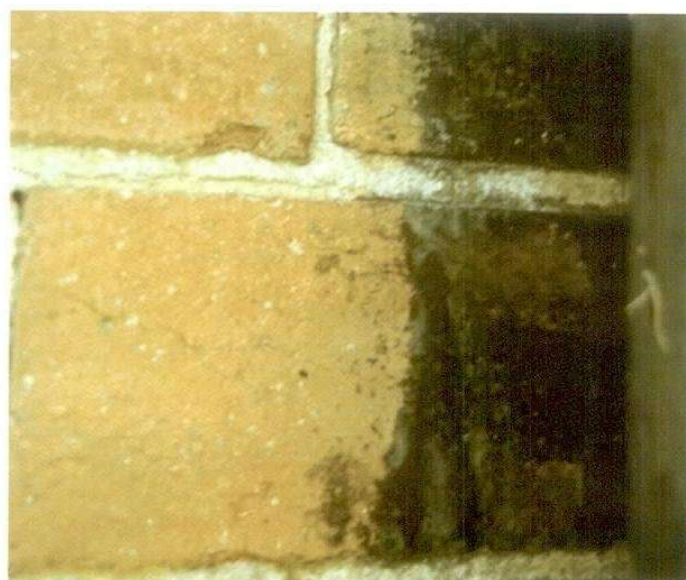
There are many types of brick in historic façades. The properties of each must be identified for the selection of an appropriate cleaning regime. The common bricks seen here are highly porous, brittle, easily damaged by impact or abrasion and variable within each brick and from brick to brick.
