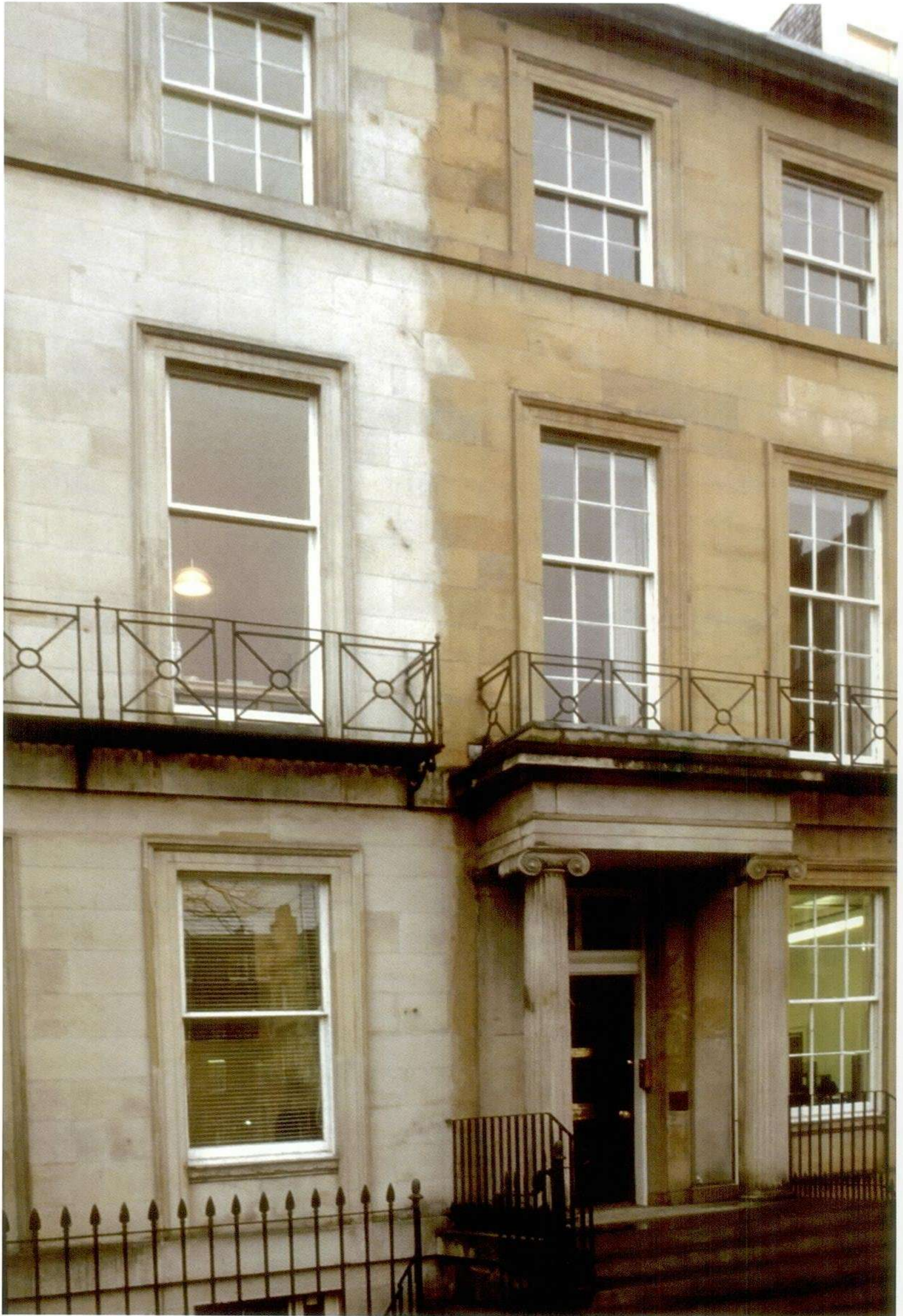
Rutland Square, Edinburgh, is an often quoted example of bad cleaning which has caused permanent damage to many of the Square's stone façades. It could so easily have been a different story.
