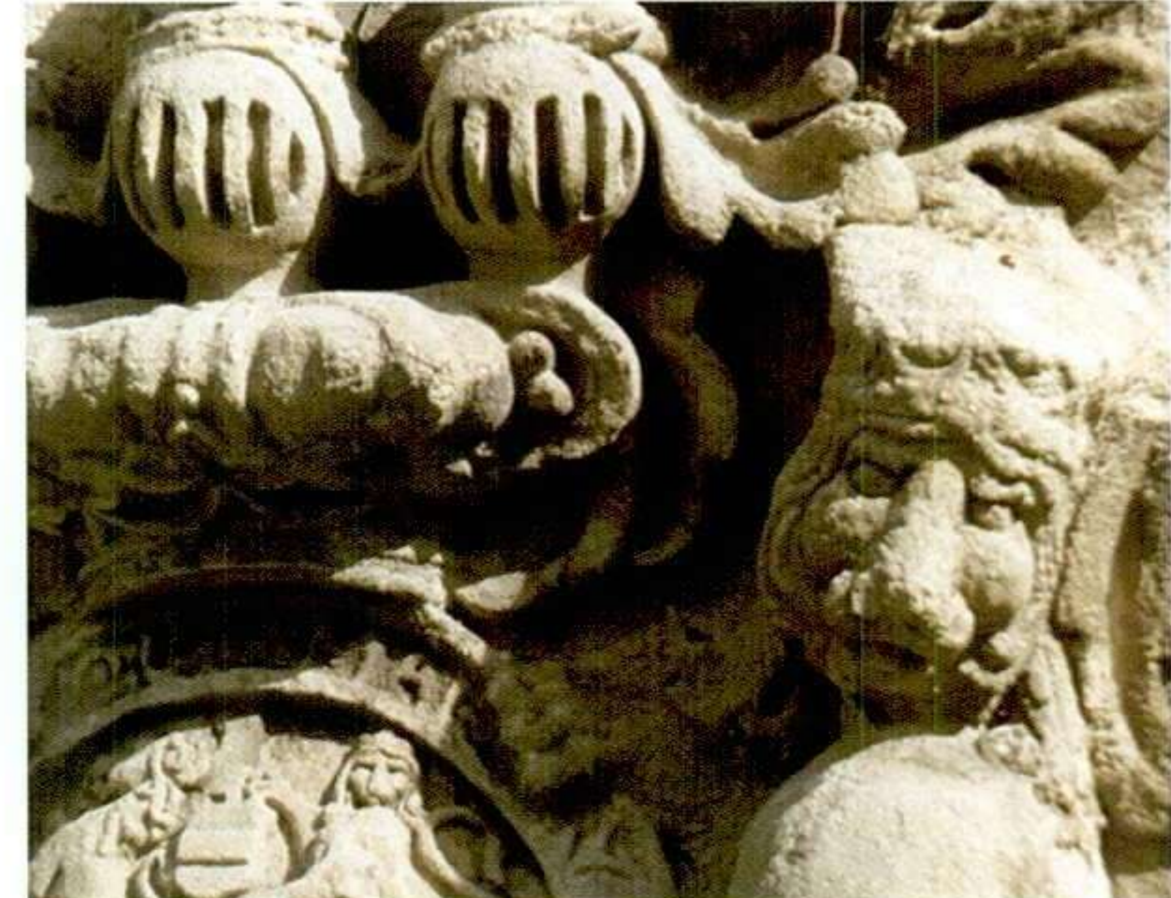
Pressure water has damaged the carved surfaces of this limestone, operating more as an abrasive clean than as a water clean. The irregularities of hardness within the stone have added further to the roughening of the surfaces.
