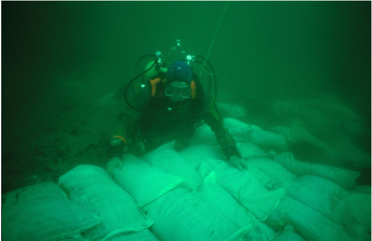
Figure 5: Laying sand-bags on the seabed to help protect and stabilise the site of a 17 th -century historic shipwreck in the Sound of Mull. When this wreck was discovered by divers, structure and artefacts had become exposed and were at risk of being lost. After a rescue excavation was completed, the hull structure has been covered in sand-bags to encourage natural processes to help re-stabilise the site and prevent further exposure of ship structure. 000-000-110-634-R – © Colin J M Martin. Licensor www.scran.ac.uk
