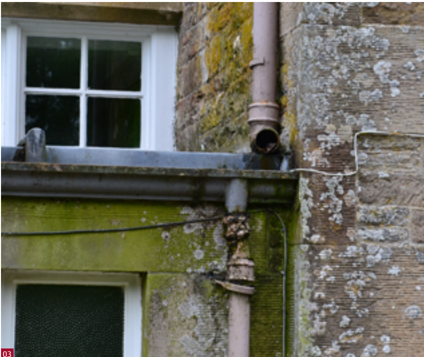
Fig. 3 Complex roof drainage is vulnerable to overloading and blockages.
