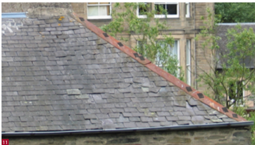
Fig. 11 This roof has been poorly maintained and is progressively failing.
