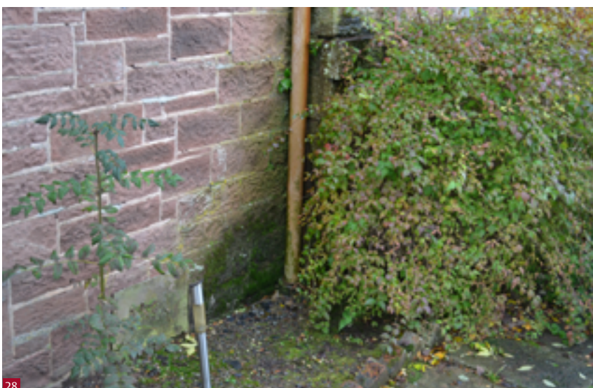
Fig. 28 A closed downpipe with a blockage; the water is backing up and overflowing causing saturation of the adjacent masonry, which is now showing green.
