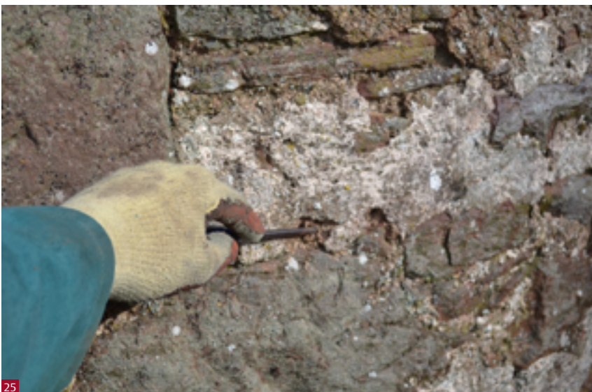
Fig. 25 The lime mortar on this wall is now weak and friable and the wall needs re-pointing.
