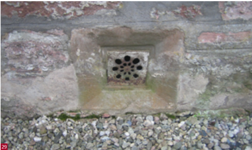
Fig. 29 The correct ground level relative to a vent grille. The green colouration on the vent stone indicates how far the ground level had previously been raised.
