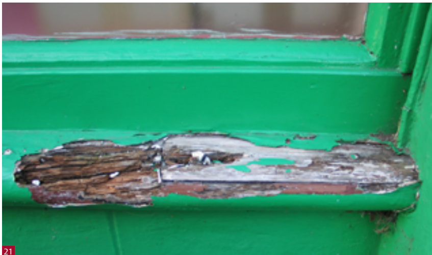
Fig. 21 A decayed timber window cill.
