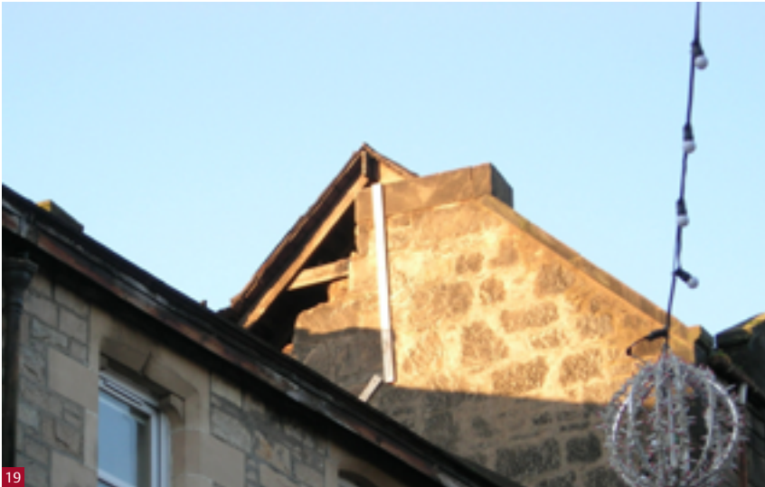
Fig. 19 The aftermath of a storm – the masonry from this chimney stack is now on the pavement below.
