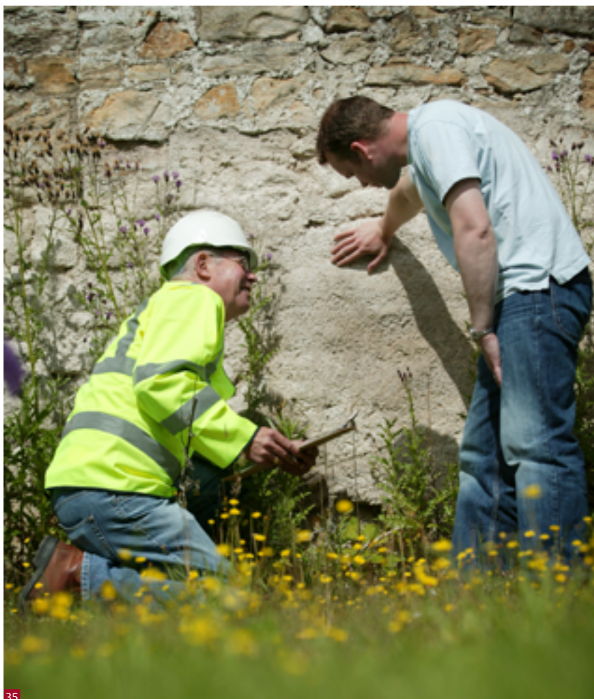
Fig. 35 Discuss the repairs on site with the contractor; samples may be needed.
