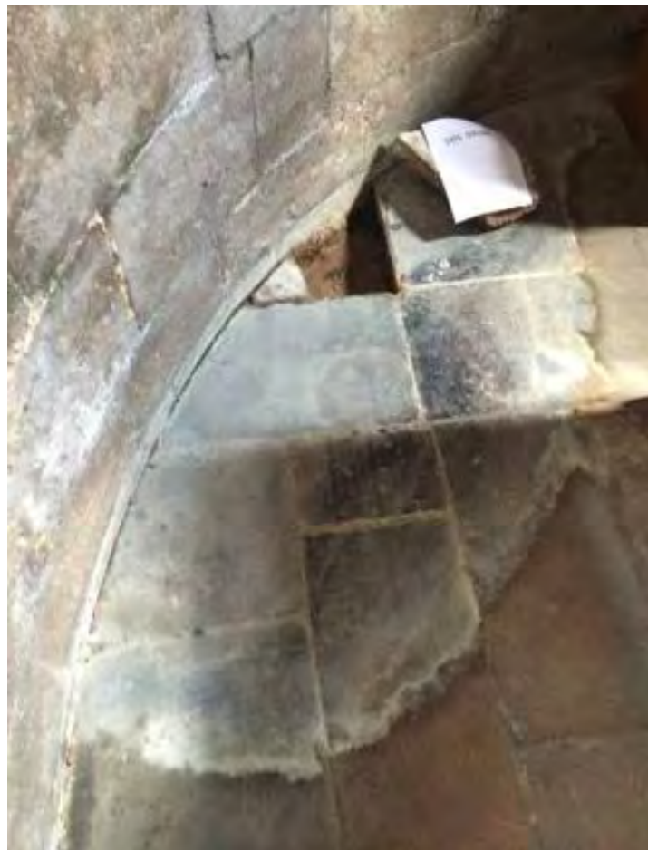
Figure 6. Damp and staining on the floor of the apse.
