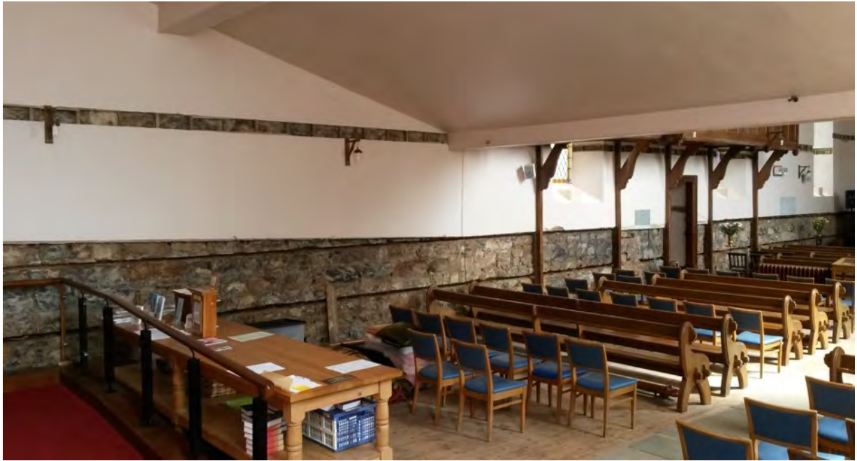
Figure 5. The north side of the nave, showing the areas of stonework exposed by removal of the decayed panelling.
