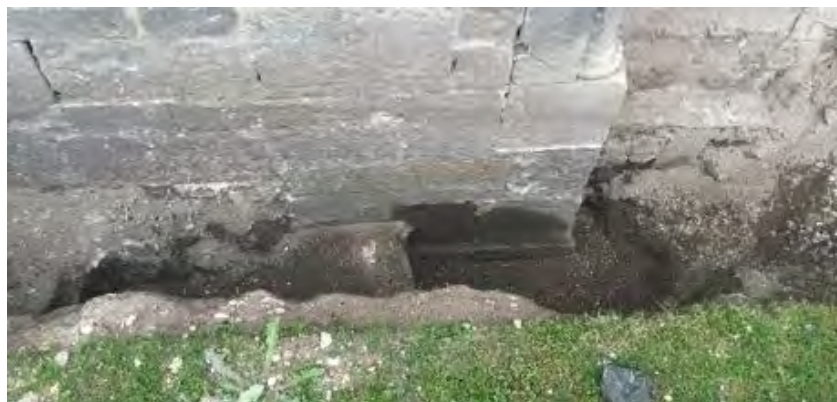
Figure 12. The base of the nave wall, now some 300mm below the present ground level.
