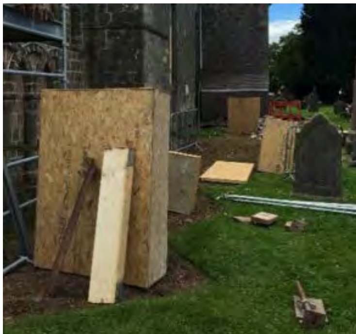
Figure 13. Timber enclosures in place to protect memorials from damage.
