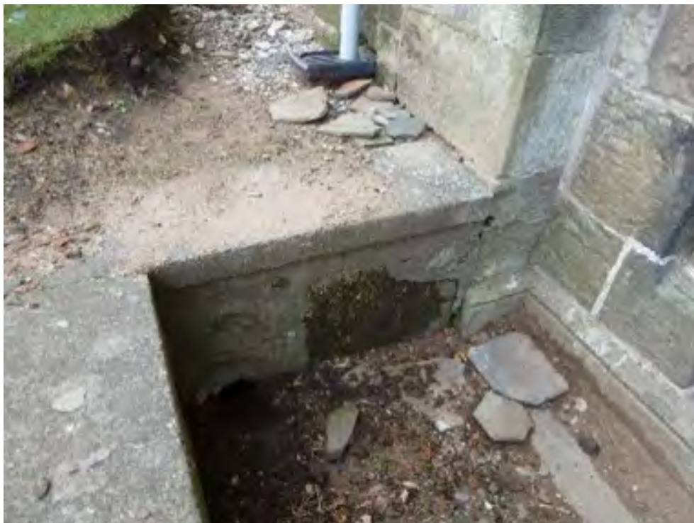
Figure 7. The outlet point (the base of the downpipe) for water from the nave roof was effectively directing water into the lowered area around the choir and the apse.
