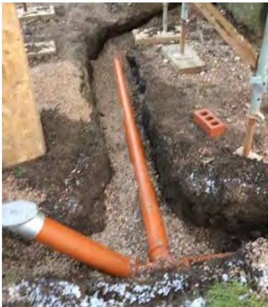
Figure 21. New drain route, note the rodding eye on the left for cleaning.
