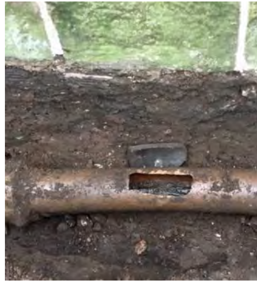
Figure 11. Fireclay drain adjacent to the nave wall, showing previous efforts to clear blockages.
