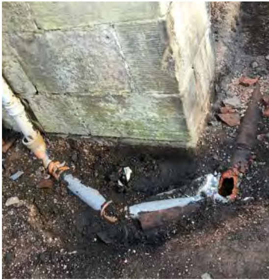
Figure 10. Long turns with no rodding facility resulted in blockages.
