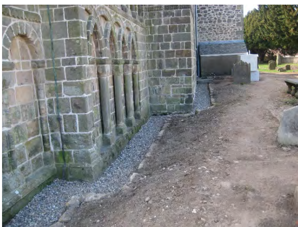
Figure 27. The finished gravel and edging on the north side of the church.
