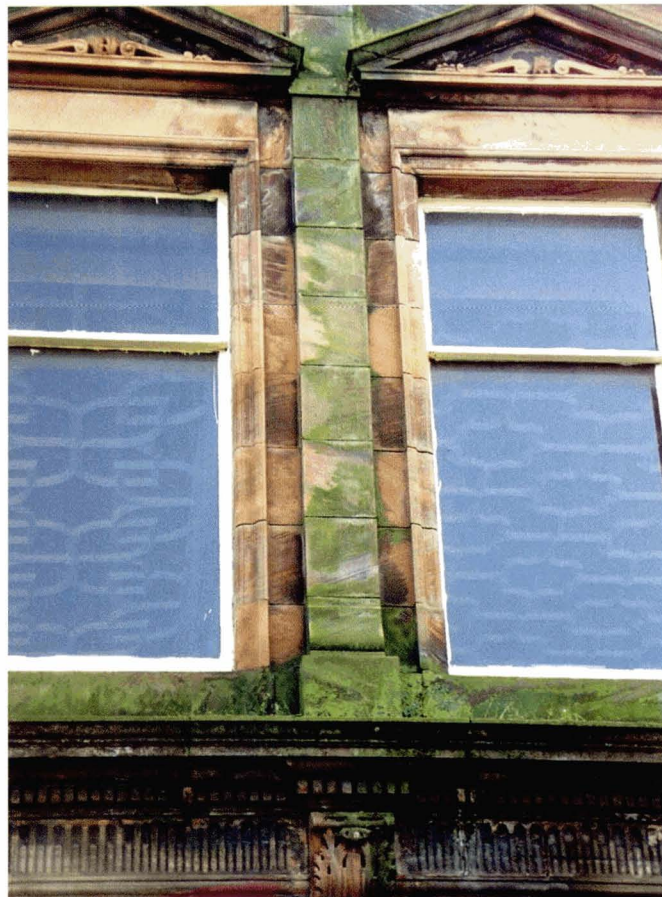
Plate 10 Colonisation by algae at run-off zone between ends of hoodmould at window lintels.
