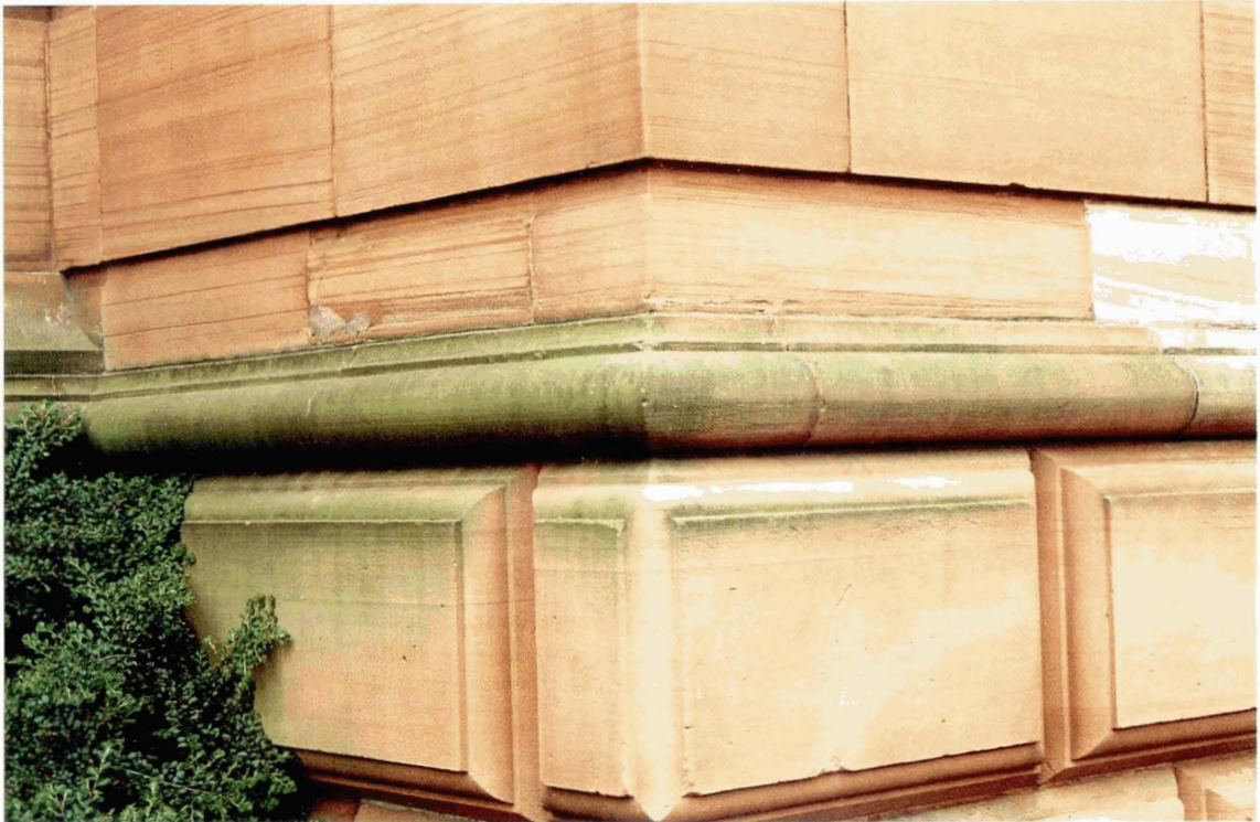
Plate 5 Corner between north west and south west elevations. Note increased incidence of algal growth on north west facing wall.
