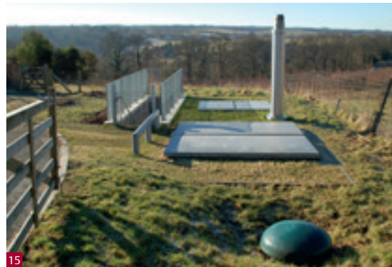
Fig. 14 Insulated accumulator tank for the biomass boiler system at Rosslyn Chapel (Category A-listed).
