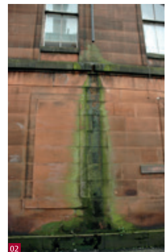
Fig. 2 Damp masonry, and the associated soiling and biological growth, can be prevented with proper maintenance, which will improve thermal comfort.
