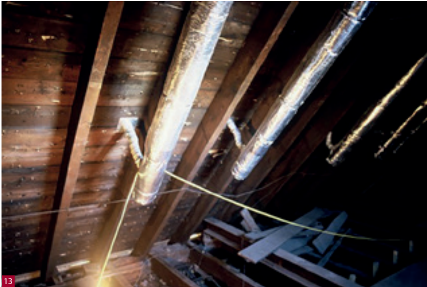
Fig. 13 Passive solar energy system which collects heated air from below the slate roof (© Richard Atkins, Chartered Architect).
