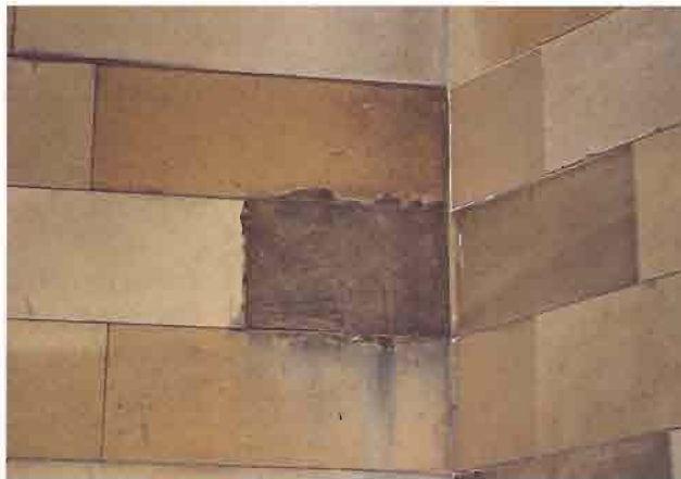
This plastic repair was coloured to match the soiled stone. When the building was cleaned, the colour no longer matched. The pigment used to achieve a soiled appearance is now running off onto underlying stone
