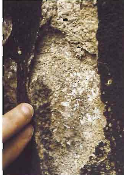
Case hardening of sandstone – a hardened crust develops over a weakened interior. The stone may appear sound until the crust is breached, but when the weakened interior is exposed there will be rapid decay
