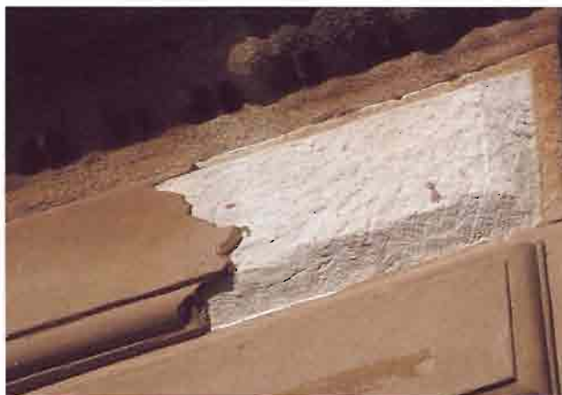
The life span of a plastic repair is short compared to that of a stone façade
