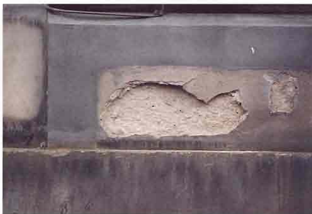
Moisture trapped by a plastic repair of low permeability can induce decay in the adjacent stone
