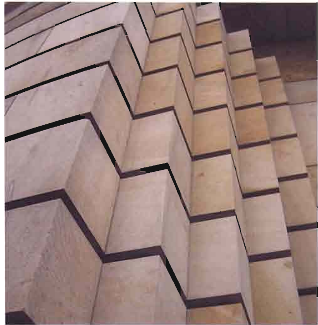
The Clashach rainscreen cladding to the Museum of Scotland by Benson + Forsyth Architects was precision cut to form a perfect curve when fixed to the circular entrance tower.
