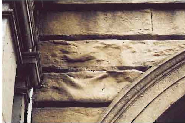
This thin layer of plastic repair has failed to bond with the underlying stone, forming the 'slumped' surface
