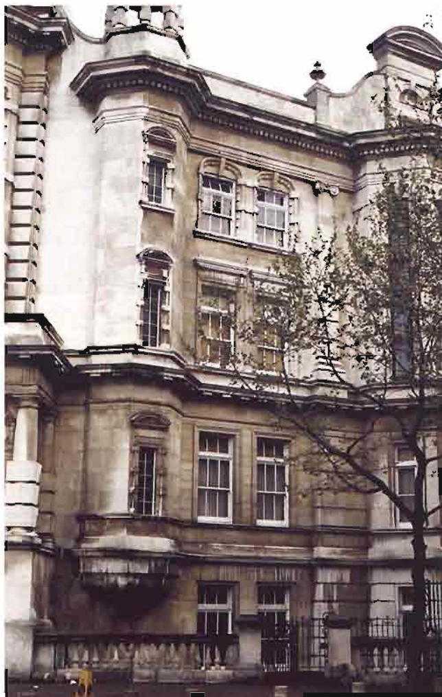
Figure 1. Typical soiling on a limestone façade. Rainwashed areas on limestone buildings remain clean due to the slight solubility of the minerals in the stone.
