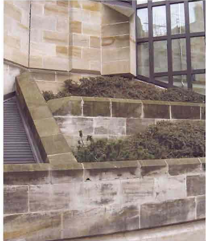
The complex design of the exterior stonework to the National Library of Scotland on Edinburgh's Causewayside manifests many of the technical issues highlighted here and in the following section.
