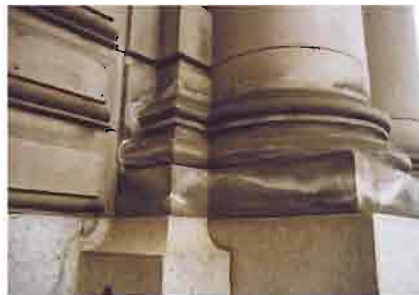
Salt concentrated in sandstone above impermeable granite. The salts are derived from residues of cleaning chemicals which reacted with pollutants in the stone. Salts of this type can cause rapid stone decay
