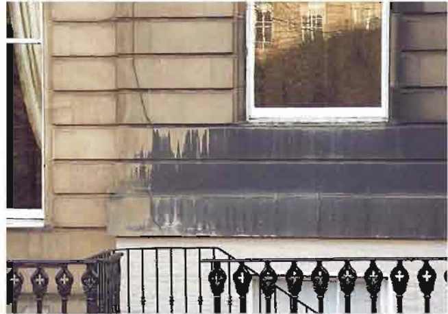
The stone around this window has been deliberately stained, probably at the time of construction, to achieve the 'expected' soiled appearance. This 'soiling' has since been partially washed off by rainwater
