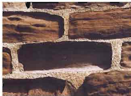
Hard pointing mortar can induce decay of adjacent stone if the mortar is more impermeable than the stone. Moisture movement, and associated decay, occurs within the stone rather than the pointing
