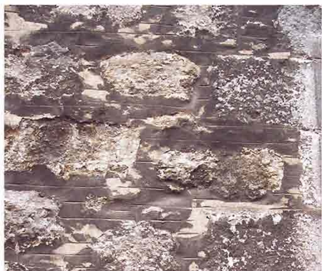
The black gypsum crust on this granite is causing blistering and disintegration of the stone surface.
