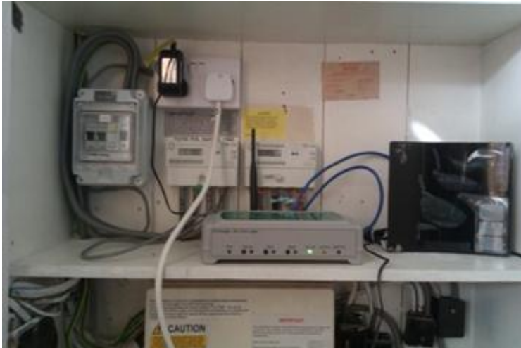
Fig. 5 Monitoring equipment installed at Scotstarvit Tower Cottage. Web logger (with green light) and power meter above.
