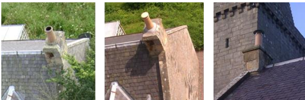
Fig. 28 Change in chimney pot. Left to right: 2011, 2012 capped with an "elephant's foot", 2013 – replaced with a cowl so the hearth or flue can still be used.
