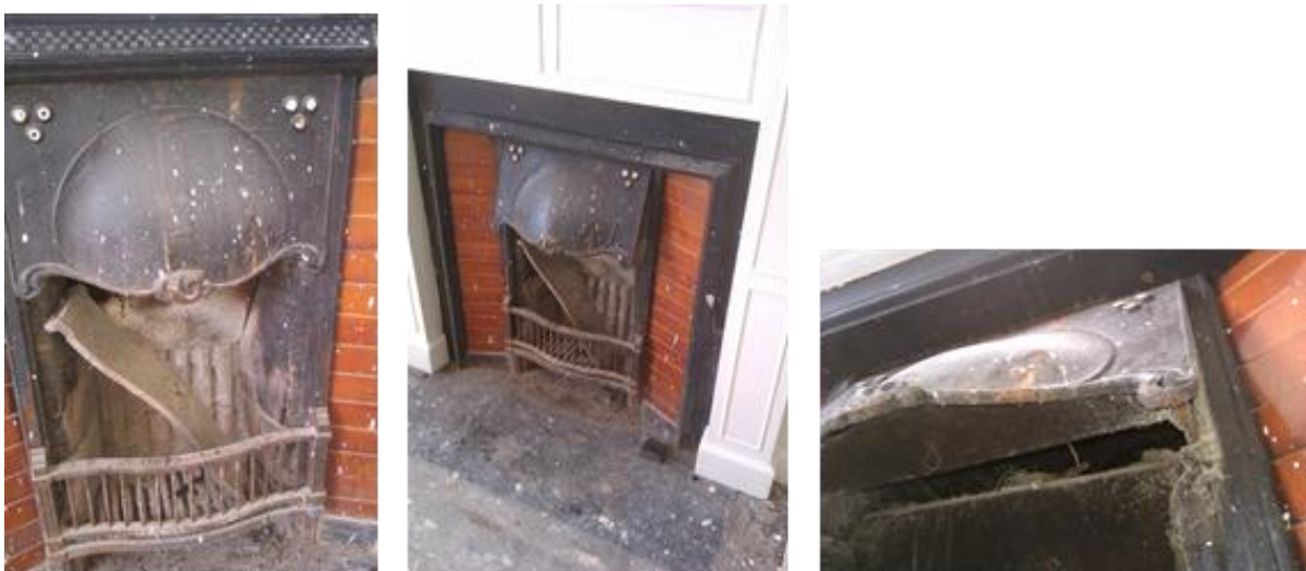
Fig. 26 Living room fireplace shown with damper closed (top left), open and suitable for use (top right and bottom).
