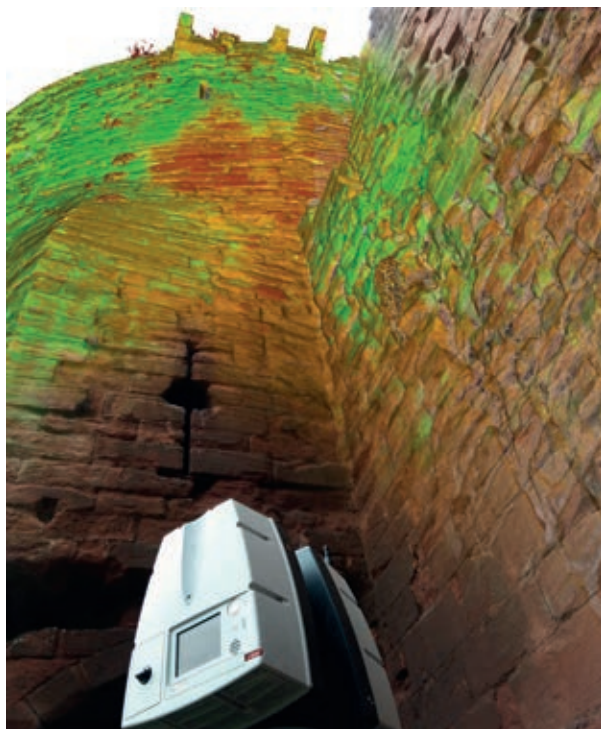
Below: Point cloud image blend from Bothwell Castle with one of the laser scanners
