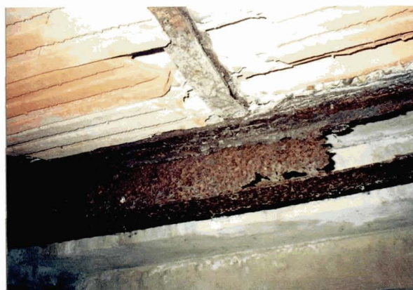
Illustration 249 Beam web loss due to corrosion A patent block floor over a neglected basement, supported (just) by a severely corroded wrought iron or steel beam. (Picture: Joe Marsh)
