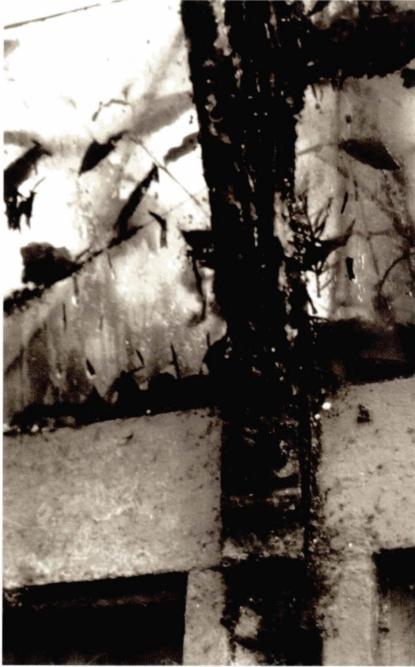
Illustration 265 Skelmorlie Castle, Largs: garden conservatory (c.1860) Severe corrosion at the lower bearing of a wrought iron rib. Note that the supporting cast iron member remains in good condition (Picture: T. Swailes)
