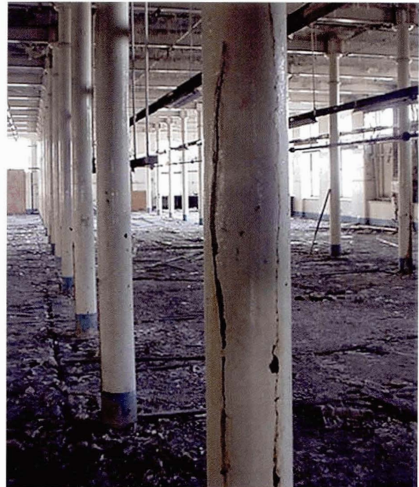
Illustration 188 Domestic Finishing Mill, Anchor Mills, Paisley (1889) Cast iron columns split by ice. Several columns became filled with water due to a defective flat roof. The water in the columns froze over winter in the semi-derelict building, which was largely open to the elements. (Picture: Buro Happold)
