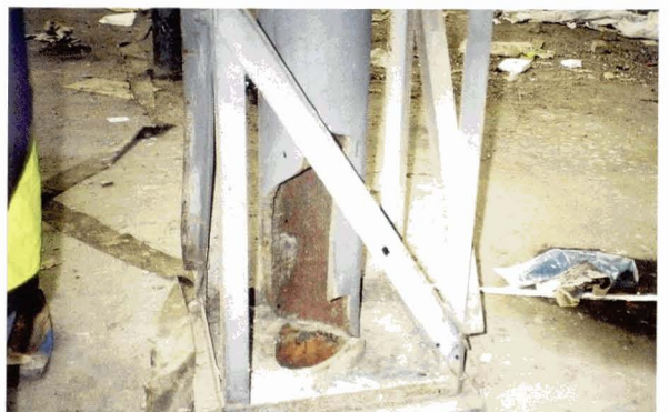
Illustration 186 Former Rail Store, Gidea Park, Essex (above) Internal view (below) Detail A 'historic repair', with a replacement column of light angle truss construction providing vertical support to an overhead crane rail support beam. The badly damaged hollow circular cast iron column was left in place, still supporting the roof (Picture: Morrison Construction)
