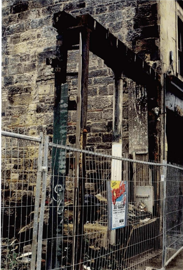
Illustration 183 Glasgow Green (probably c.1850) Shop front framing during demolition (Picture: T. Swailes)
