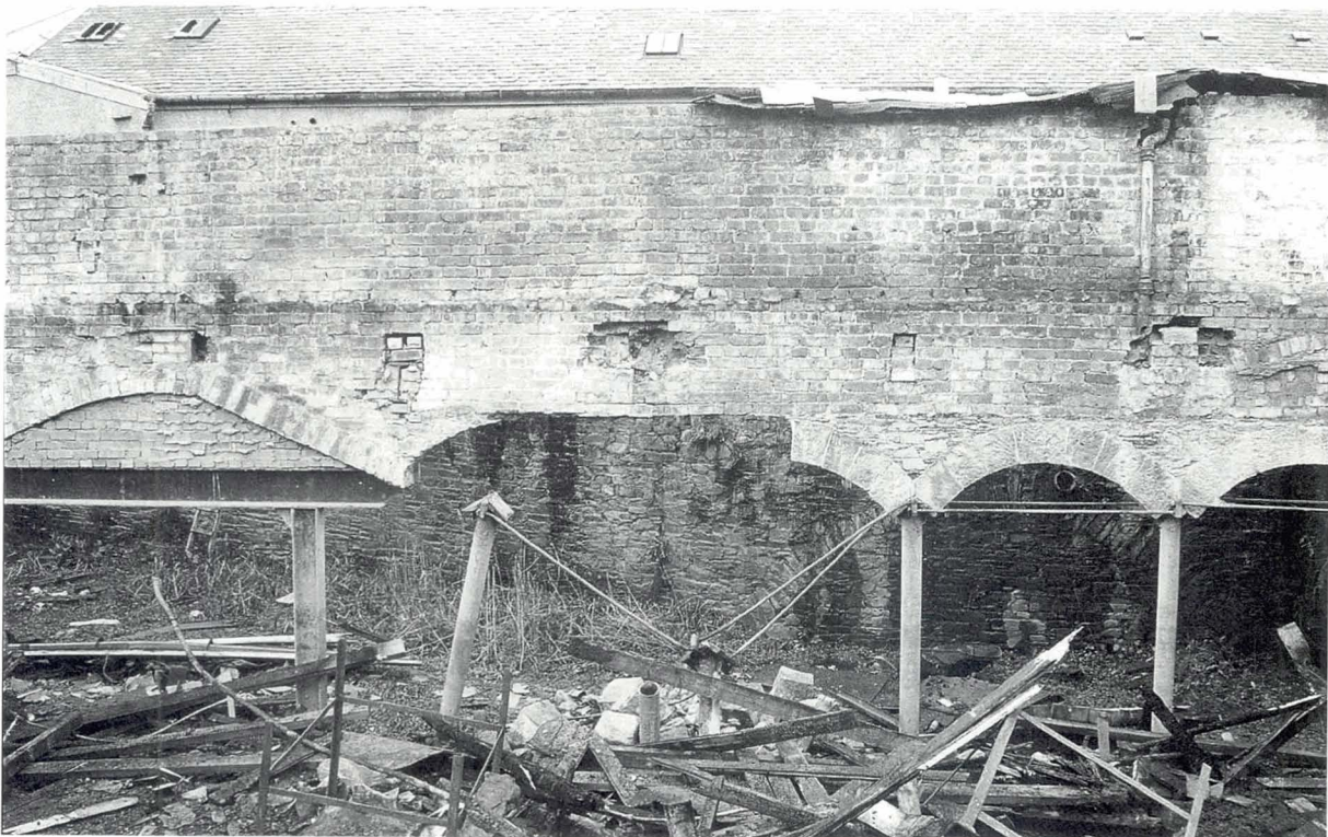
Illustration 227 Weensland Mill, Hawick (1850) After partial demolition of the remains of the burnt out mill, a masonry wall bridges over two fallen supporting columns (Picture: T. Swales)
