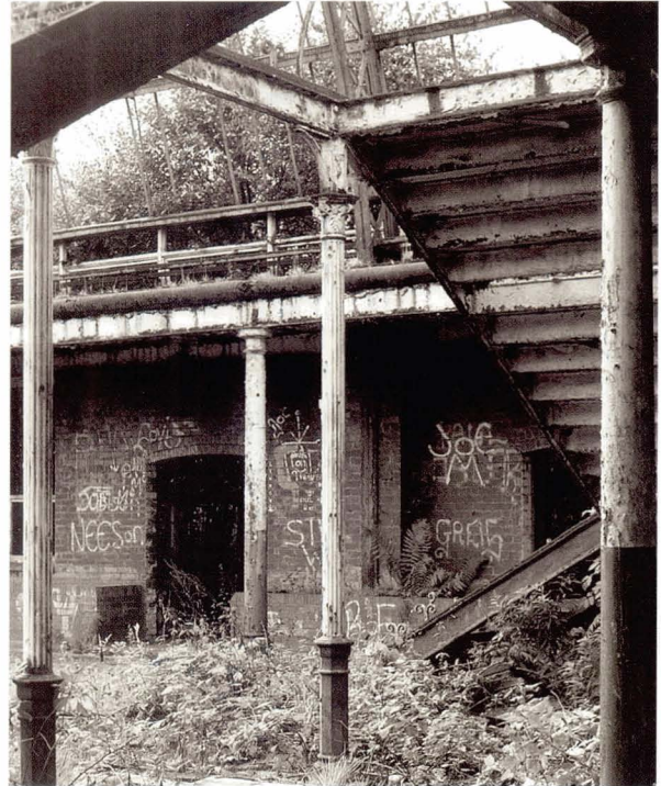
Illustration 104 Springburn Park Winter Gardens (1899). The dilapidated iron-framed interior in 2001. The filler joists to the gallery floors are likely to be steel (Picture: T. Swailes)
