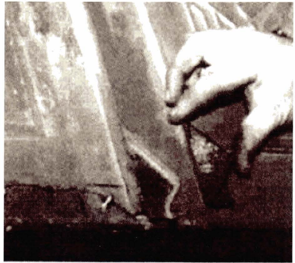
An unusual conservation project: a gentleman's toilet in central London, made of cast iron panels only 6mm thick. Conservation work included a broken panel which was repaired by bolting to backing plate of galvanised steel 2mm thick bedded on resin and sealed round. If such a thin plate of cast iron had been welded, it would have cracked repeatedly: welding is not recommended for thin sections.
