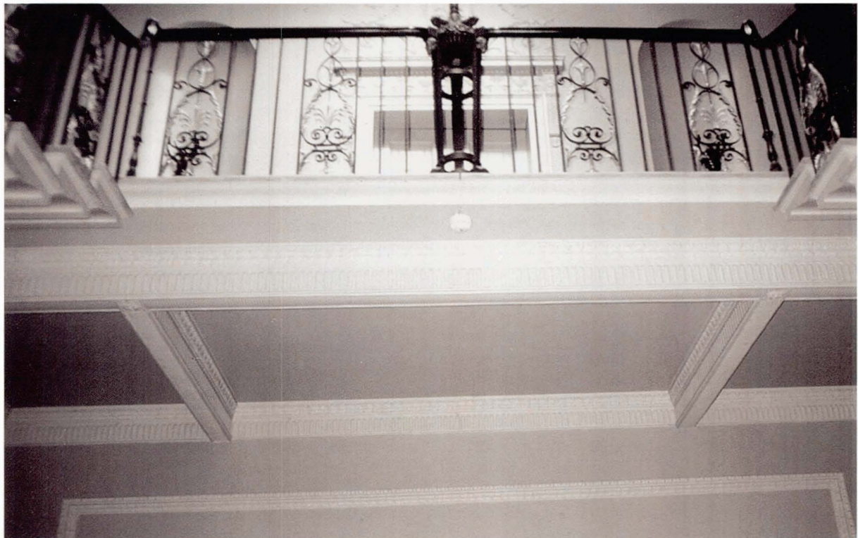
Illustration 82 Heaton Hall, Lancashire (1776) Staircase landing support beam. Examined initially from ground floor level, the slender beam was assumed to be timber with an iron flitch plate. On investigation with a 'cover meter', the beam was found to be (most probably) of solid cast iron, moulded to exactly match the decorative plasterwork. Secondary beams of identical appearance provided a second surprise, being hollow 'dummies', provided purely for aesthetic reasons. (Picture: Joe Marsh, UMIST)
