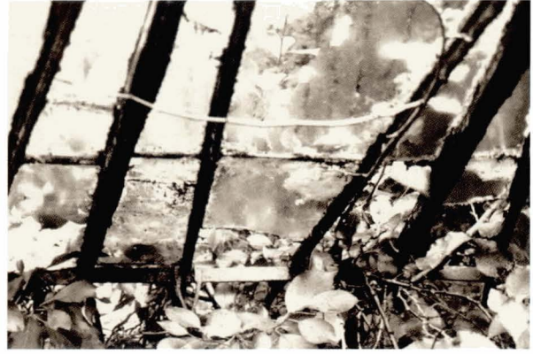
Illustration 266 Skelmorlie Castle, Largs: garden conservatory (c.1860) Curved wrought iron ribs to the roof comprise strip riveted to the sides of rectangular bar, as a bearing for the glazing. With the glazing incomplete, the detail traps water (Picture: T. Swailes)
