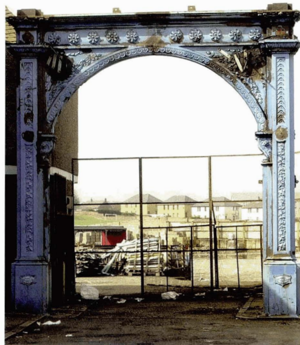
Illustration 110 The Grahamston Gate Unightly makeshift repairs to cracks, prior to conservation work (Picture: Historic Scotland)
