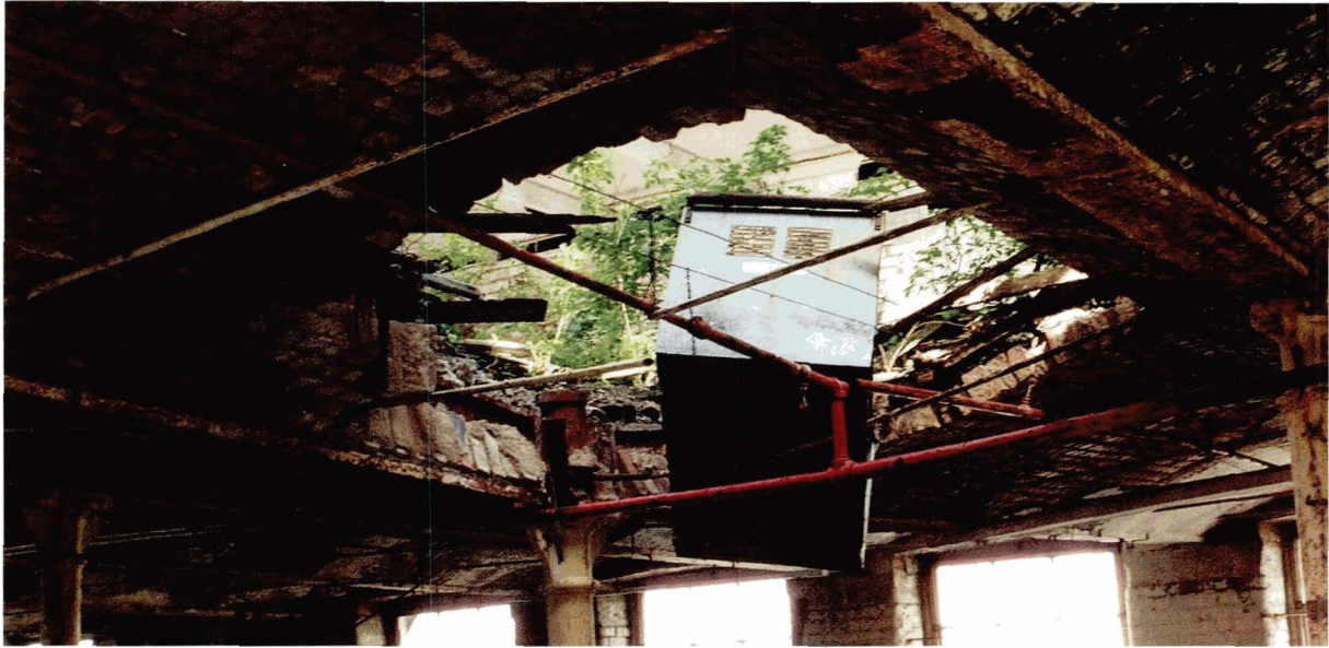
Illustration 137 Gourock Rope Works (1866) Partial floor collapse (Picture: Malcolm Waters, Historic Scotland)
