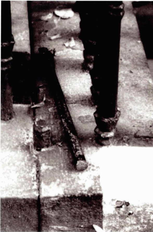
Illustration 262 Broken cast iron railings (Picture: T. Swailes)
