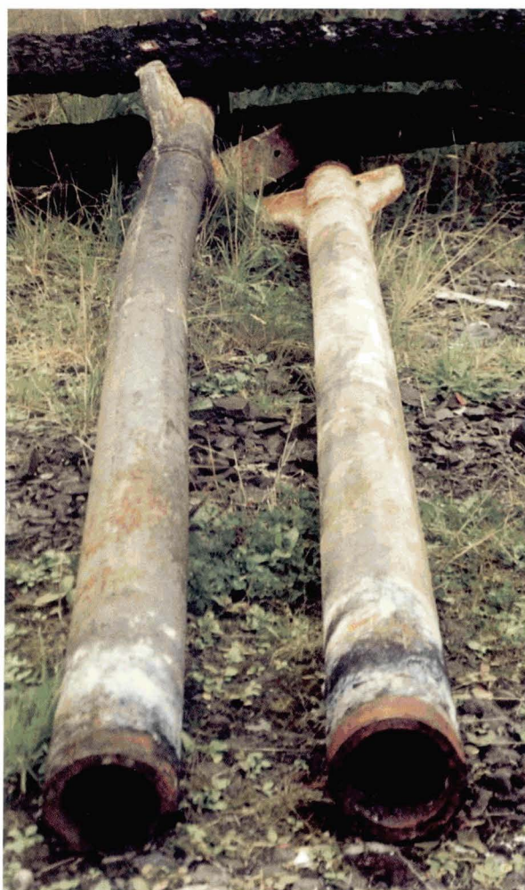
Illustration 242 Stanley Mills. Cast iron column bent in fire (Picture: T. Swailes)
