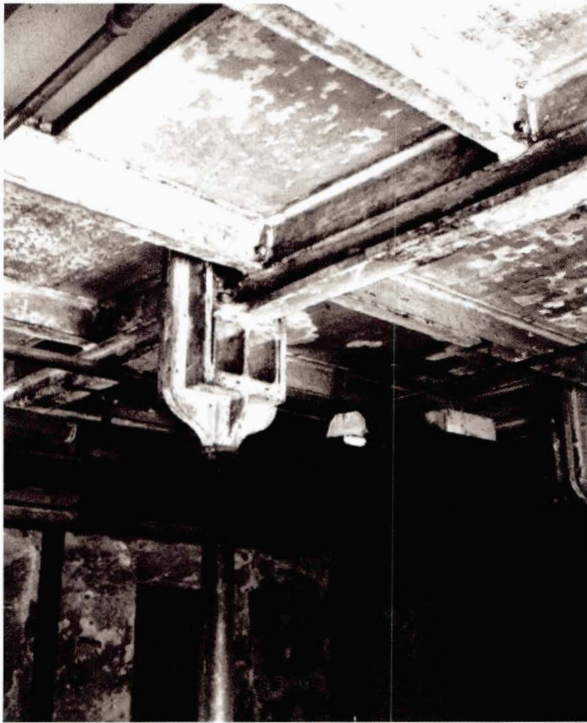
Illustration 38 Grandholm Works, Aberdeen: Old Spinning Mill (1793-4, modified 1820s) Iron framing and stone flag floors (Picture: T. Swailes)
