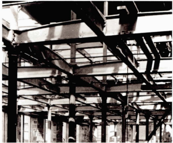
Illustration 39 Mid-Wynd Works, Dundee (1894 and 1903) The iron framing to a power loom factory under construction. The specialist textile engineering firm Robertston & Orchar of Dundee used cast iron beams here in the structural framing at a time when rolled steel beams were being used in other kinds of building. The vibrations due to power looms demanded a very solid floor and weaving sheds were usually of single storey construction with ground bearing floor slabs. In this case a constricted, steeply sloping site made 3 and 4 storey buildings with heavy suspended floors necessary (Picture: Dundee Archive and Record Centre)
