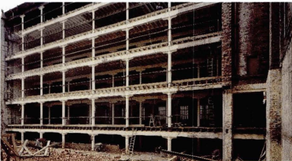
Illustration 40 Robertson's (later Watson's) Bond, Seagate, Dundee (1897, rebuilt after a fire in 1907) The structure exposed by partial demolition of this former deep-plan bonded warehouse during conversion to residential use (Picture: RCAHMS/ The Drawn Evidence)
