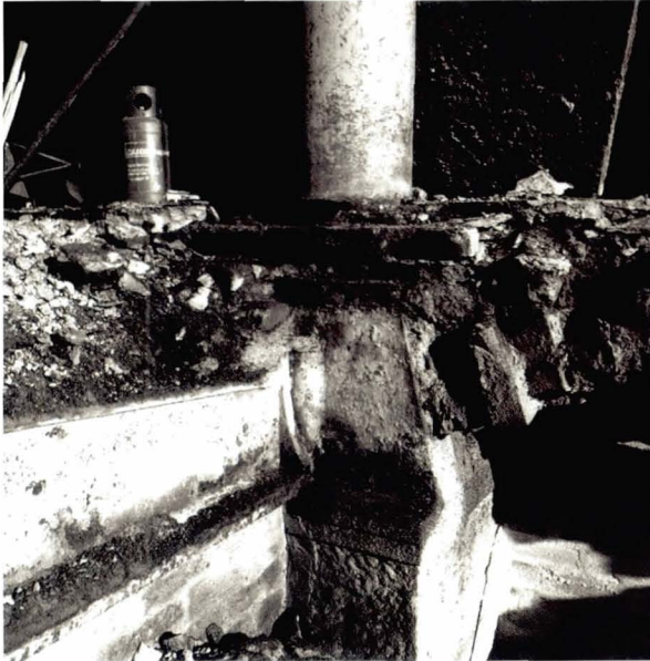
Illustration 202 South Mill, Dundee (1864) A cast iron column on a large cast iron base, also supporting a ground floor beam (Picture: RCAHMS)
