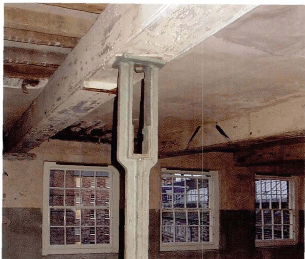
Illustration 28 Bell Mill (or West Mill), Stanley Mills, Perthshire (1786-7) Cast iron storey posts with timber beams continuous over (Picture: Mark Watson, Historic Scotland)
