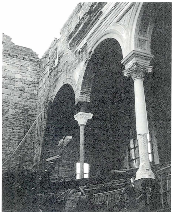
Illustration 136 Langside Hill Church, Glasgow (1896) Cast iron columns beneath lath and plaster. The building is now a restaurant (Picture: Neil Ross, Historic Scotland)
