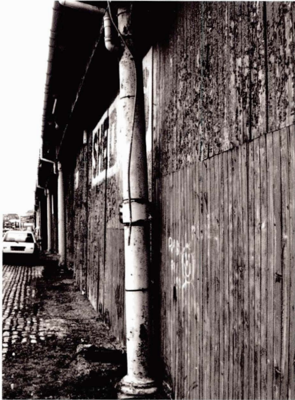
Illustration 187 Dockyard Transit Shed, Victoria Dock, Dundee (1874) Fractured quayside column (Picture: T. Swailes)
