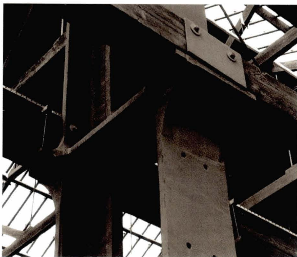
Illustration 210 Linthouse Marine Engine Works, Scottish Maritime Museum, Irvine (1872) Cast iron stanchion detail (Picture: T. Swailes)
