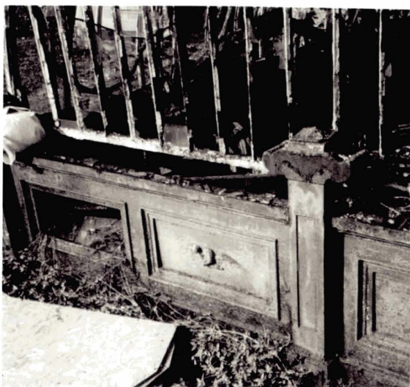
Illustration 215 Fairfield House conservatory, Dalkeith (c.1835) Ironwork detail, prior to restoration (Picture: Heritage Engineering, The Industrial Heritage Company Ltd)
