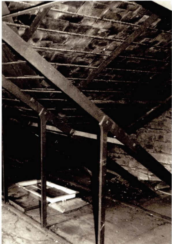
Illustration 37 New Lanark: East end of Mill 3 (c. 1826) The iron-framed attic (Picture: T. Swailes)
