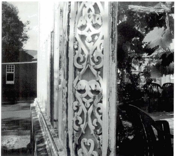
Illustration 268 Kingsknowe Hotel conservatory Damage to cast iron facing panel. Water can penetrate to the rear face of the panel, which is inaccessible for cleaning and painting. Water ingress is also likely to lead to deterioration of the timber elements (Picture: T. Swailes)
