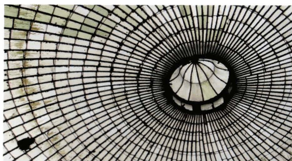
Illustration 144 The Kibble Palace, Glasgow Botanic Gardens (1873) (Picture: Glasgow City Council) The rotational twist of the dome between the inserted clerestory and the lantern is apparent from the curvature of the glazing bars.
