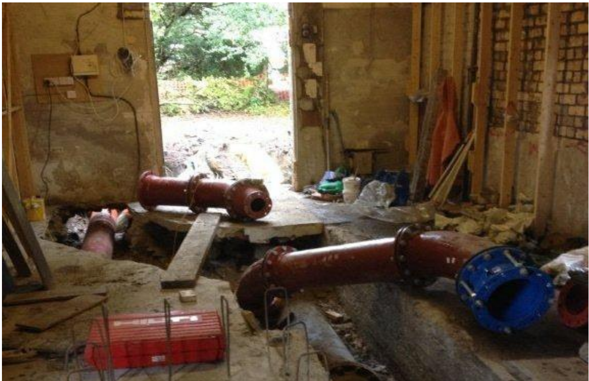
Figure 20: The installation of the new pipework in the turbine house (image Atholl Estates).
