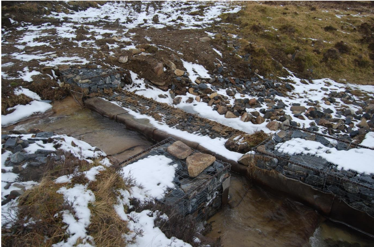
Figure 12: One of the new spillways needed to manage surges in water coming off the hill in periods of high rainfall or snow melt.
