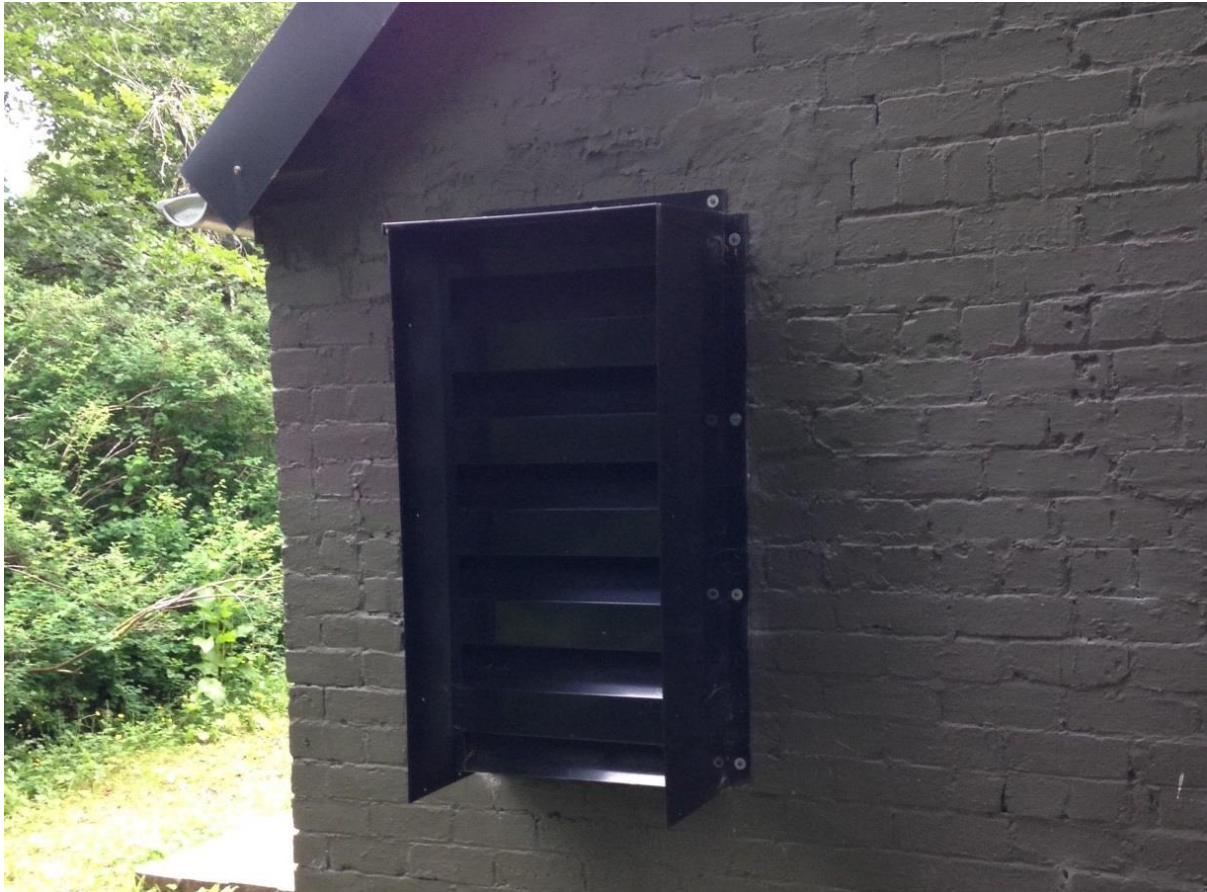
Figure 18: One of the noise mitigation features in the turbine house – a sound proofed ventilation opening.
