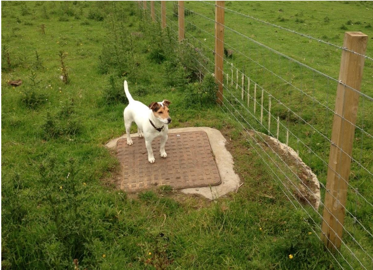
Figure 16: The manhole cover over one of the new chambers for the isolating and air bleeding valves (image Atholl Estates).
