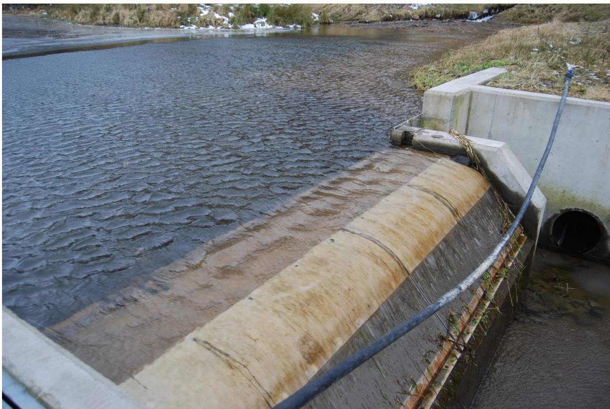
Figure 15: The new cill for the holding pond. Note the filter screen designed to keep debris out of the penstock.
