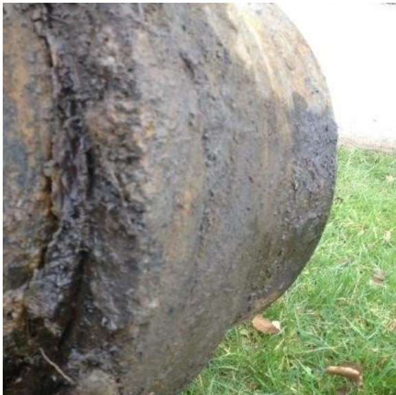
Figure 9: A section of the 1908 steel penstock was removed to allow close inspection and assessment (image Atholl Estates).
