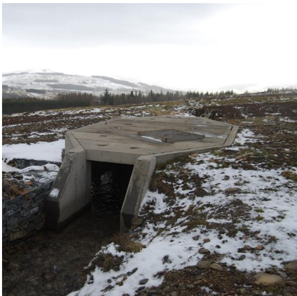
Figure 13: The new concrete silt trap on the hill moor behind the castle.
