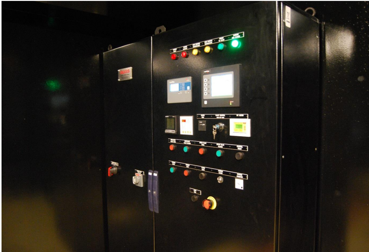
Figure 21: The new control panel and switchboard for the turbine and dynamo.
