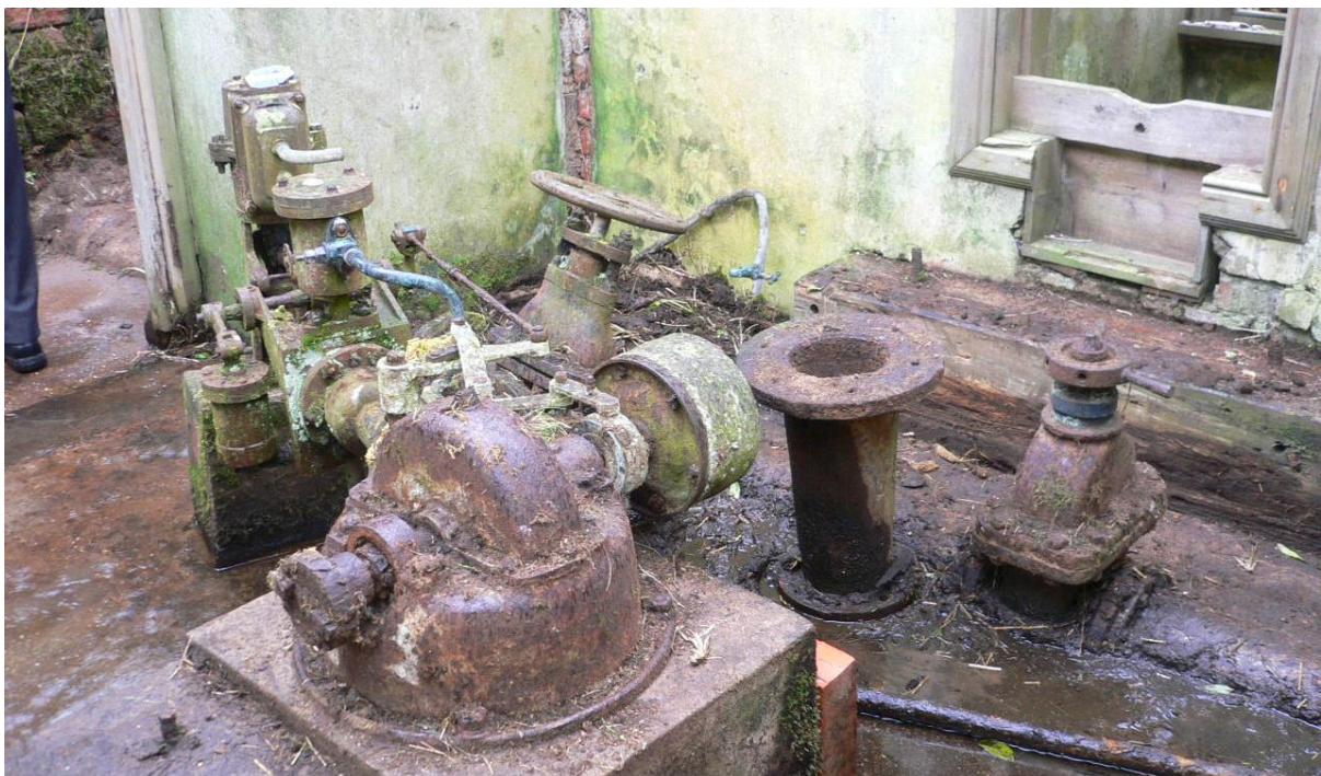
Figure 4: A 1909 Gilkes turbine surviving near a country house in Berwickshire.
