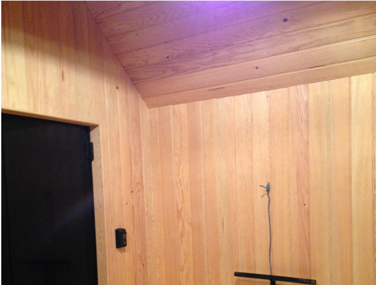
Figure 17: The new entrance lobby of the turbine house finished in local Scots Pine from the Blair Estate.
