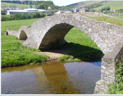
Stow Packhorse Bridge in the Scottish Borders has been retained although it is now redundant.
