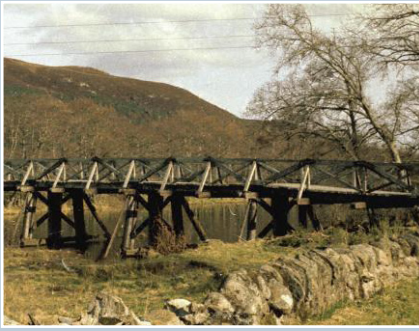
This bridge at Garve, Highland, is one of only four of its type to survive. Built during the late 19th century, the bridge is of timber trestle construction, and consists of eight spans, with six main truss spans. © Crown copyright: RCAHMS. Licensor www.rcahms.gov.uk .
