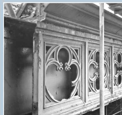
Dalmarnock Bridge, Glasgow, is a series of wrought iron girders behind a gothic cast-iron panel. It was strengthened in 1996 by insertion of new steelwork. The repaired cast-iron parapet is protected from traffic by bollards.
