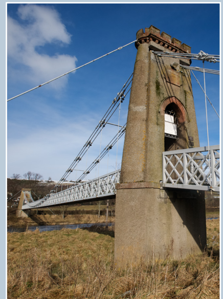
The same bridge at Gattonside after its reconstruction in 1991–2. The parapet of the same bridge is so straight that it now acts as a girder. Chains and connections are much heavier and while some fabric has been retained its character is compromised.
