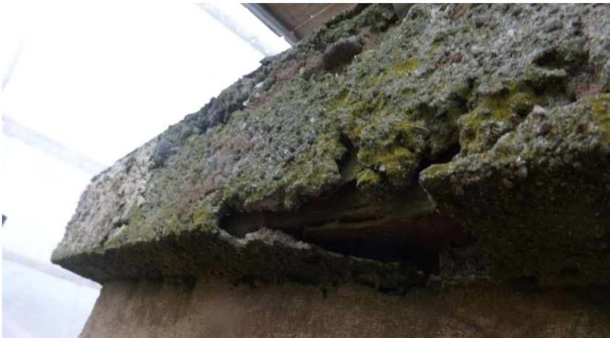
Figure 11: Degraded and defective concrete chimney cope.
