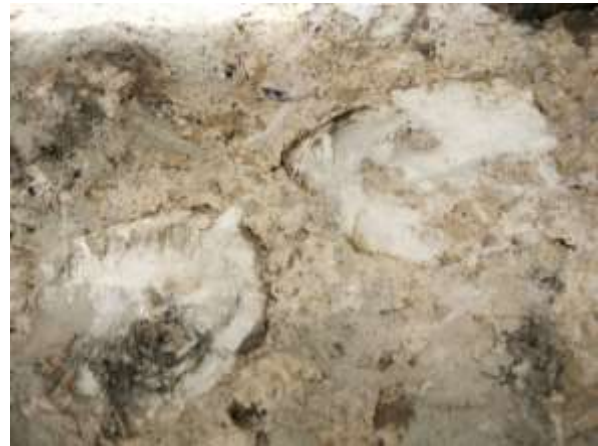
Figure 14: Oyster shell pinnings in the original underlying mortar mix.
