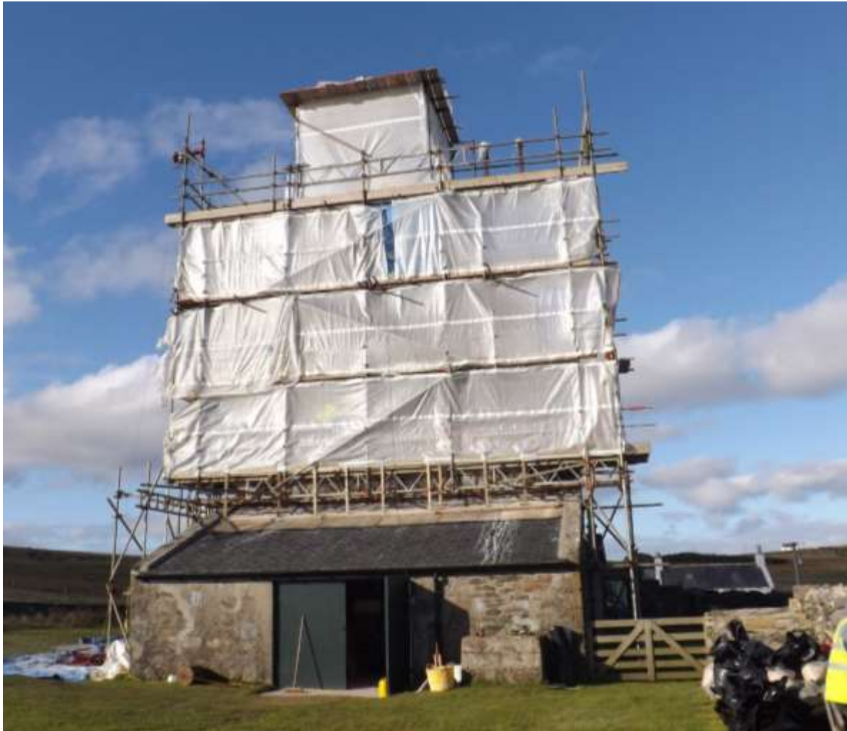
Figure 16: Work on site October 2014. The lime work was protected with plastic sheeting during works to prevent rapid drying.
