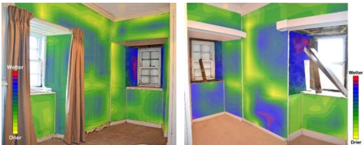
Figures 22 and 23: Pre-intervention moisture patterns within the gable at a depth of 30cm into the wall. The darker areas indicate high levels of damp.
