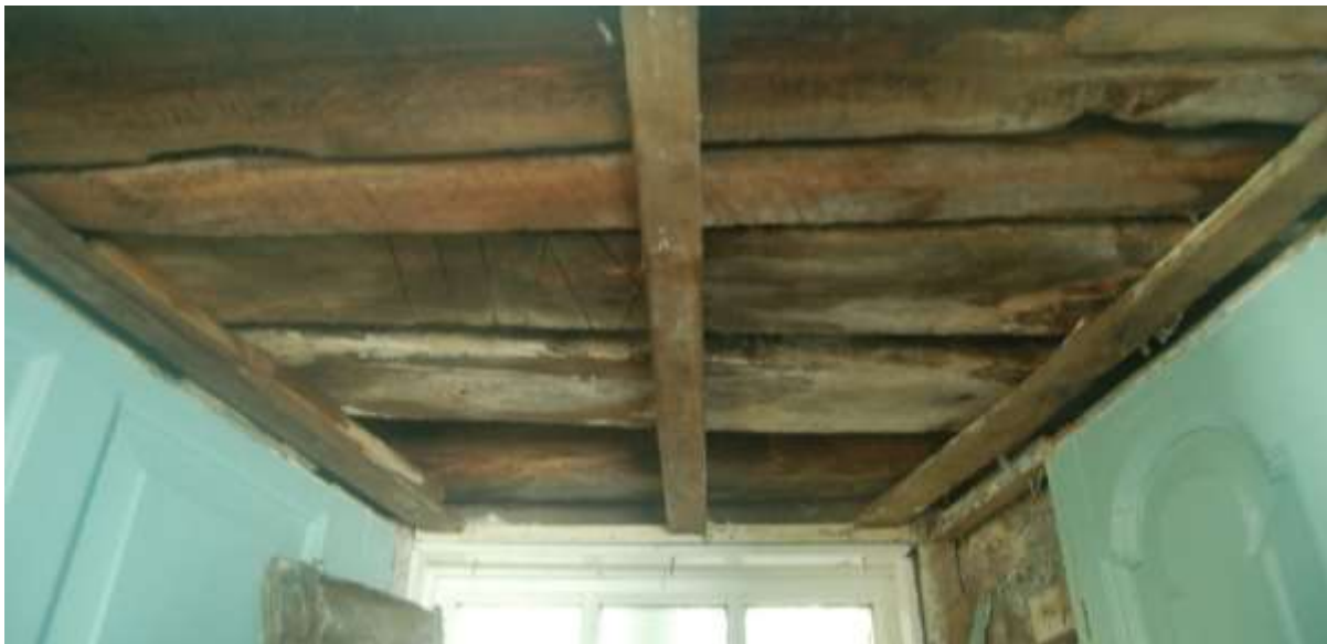
Figure 9: Water damage to window soffits.
