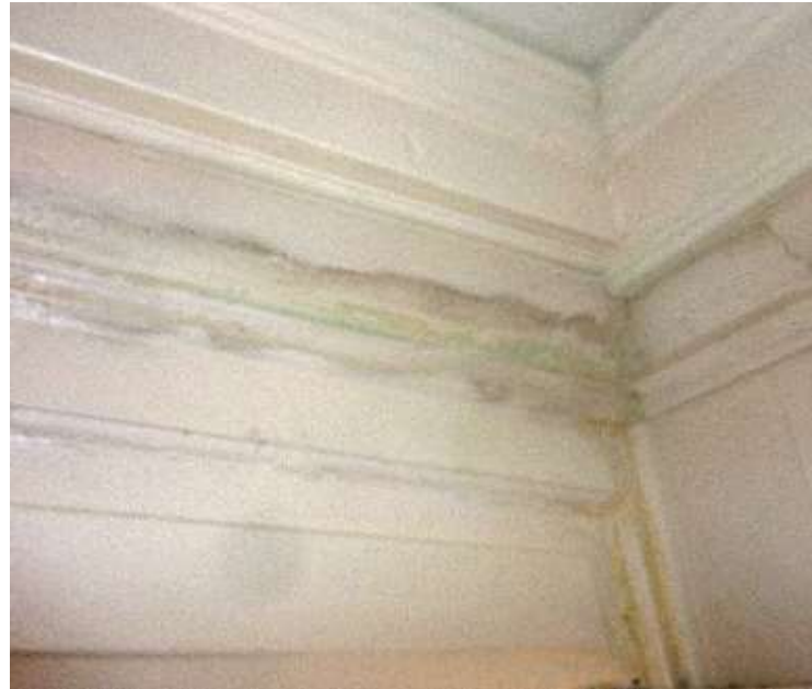
Figure 8: Water damage to panelling and cornice.
