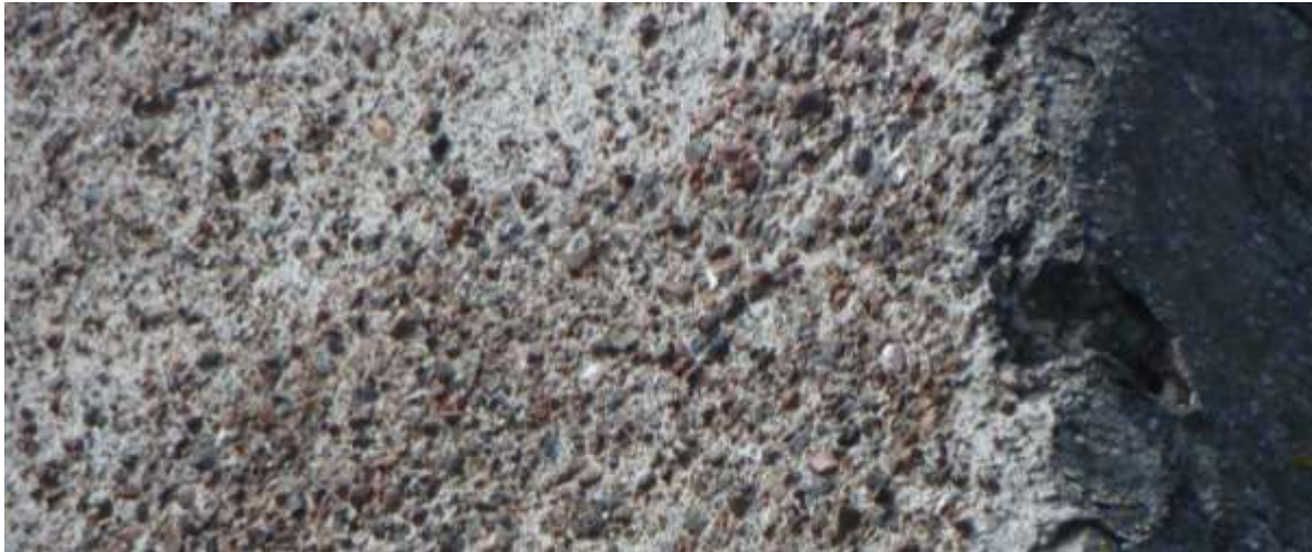
Figure 10: The existing cement-based roughcast was in poor condition.
