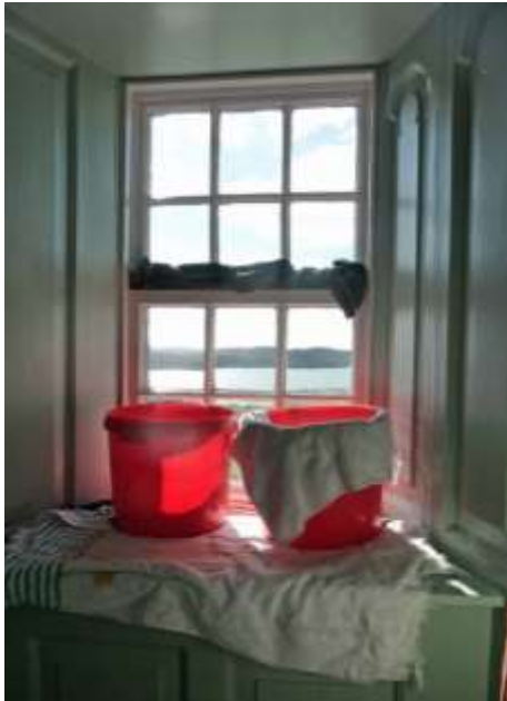
Figure 7: Water penetration around windows during bad weather (Photo: Redman Sutherland Architects).
