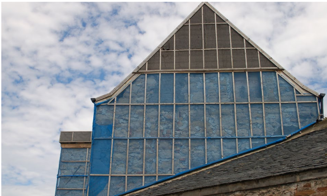
Harlaw Hill House in Prestonpans is a case where a program of non-traditional repairs was undertaken to help avoid the total or substantial demolition of the A-listed building © Courtesy of HES.
