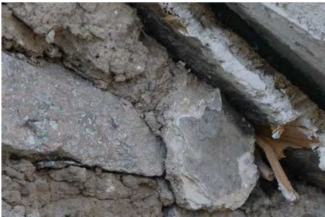
Figure 18: One fragment of original lime harl with limewash was found beneath the cement render.
