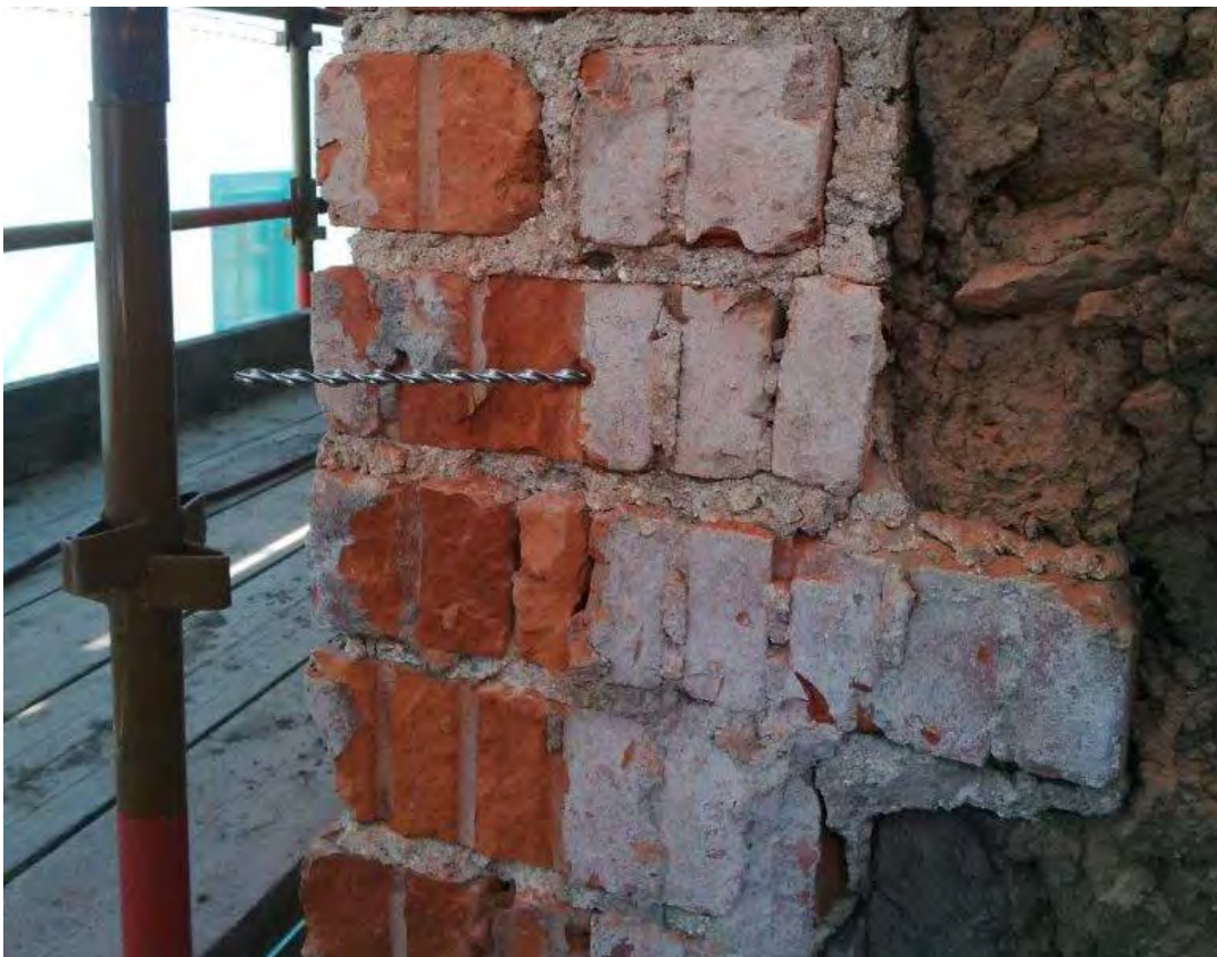
Figure 10: HeliBar being inserted to tie the corner brickwork to the main mudwall.
