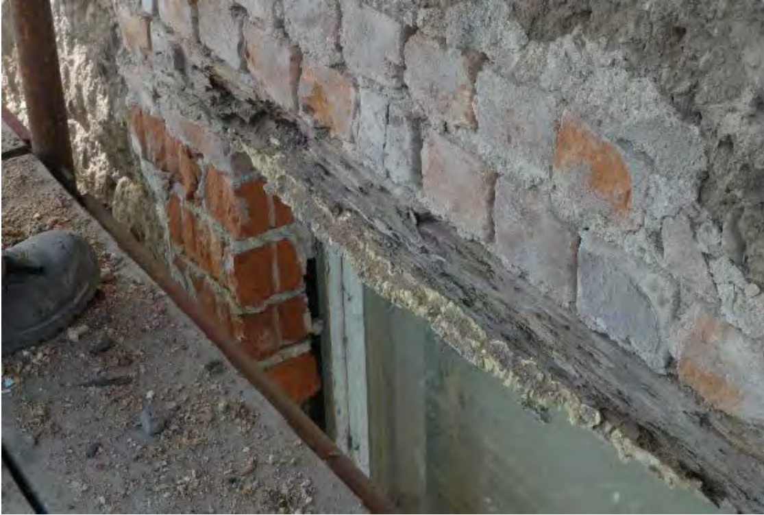
Figure 8: Removing the cement revealed rotten timber lintels supporting brick infill on slender brick facings.
