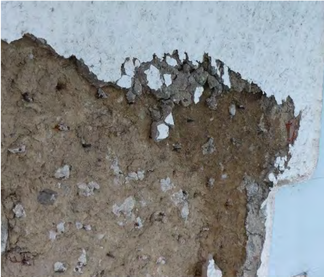
Figure 7: The darker area is damp mudwall, which lightened as it dried.
