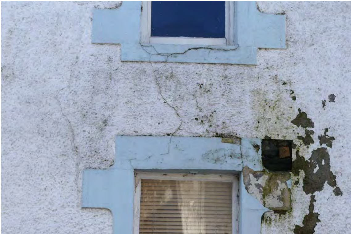
Figure 3: Cracks in the cement render
