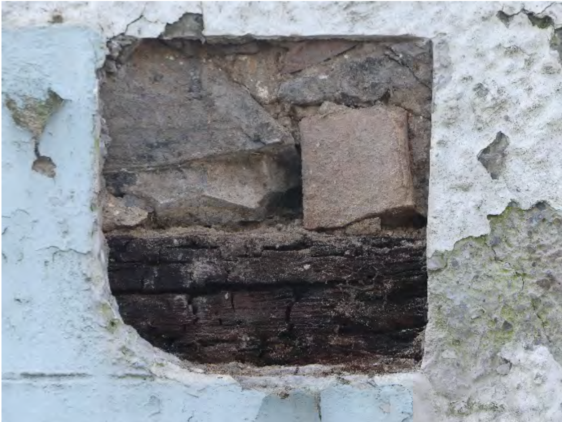
Figure 4: Inspection hole revealing a decayed timber lintel.
