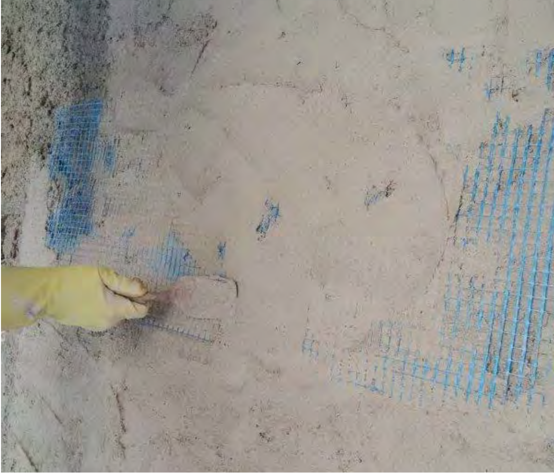
Figure 16: Plastic mesh reinforcement across substrate junctions to prevent cracking of the lime harl.
