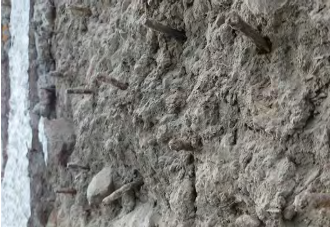
Figure 13: Some of the numerous rusted nails that had to be removed.
