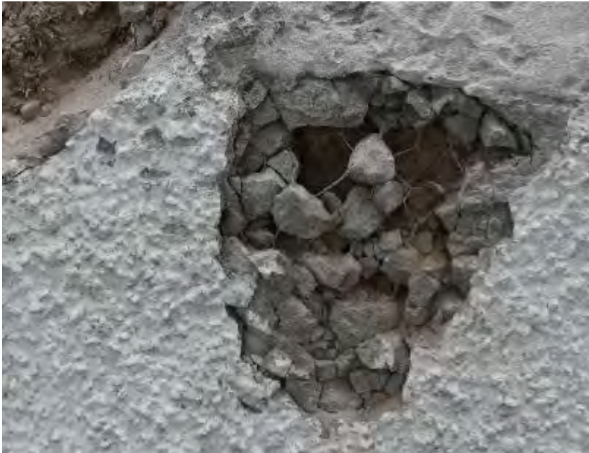
Figure 6: The cement render was reinforced with chicken wire.
