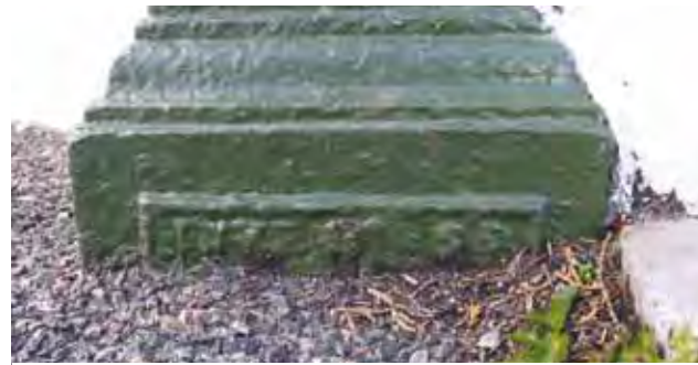
Fig. 88 Railing 13, gate post made by the Inverness Foundry (although the adjoining railing matches a design made by George Smith & Co, Sun Foundry, pattern 977)
