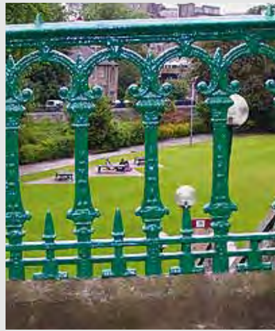
Fig. 289, Union Terrace, Aberdeen Unmarked but probably made by Walter MacFarlane & Co, pattern number 1126 This variation differs slightly from the Stornoway example by the addition of a handrail instead of little finial detailing along a top rail. Also unlike the Stornoway example, the lower rail and feet are either hidden within the supporting plinth or absent altogether. Image courtesy of The Scottish Ironwork Foundation
