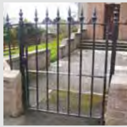
Gate 5 Manufacturer unidentified
