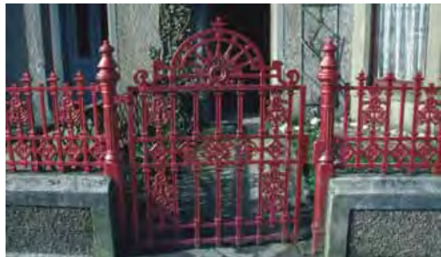
Fig. 375 Railing 27 and Gate 27 King Harald Street, Lerwick Image courtesy of Shetland Museum and Archives
