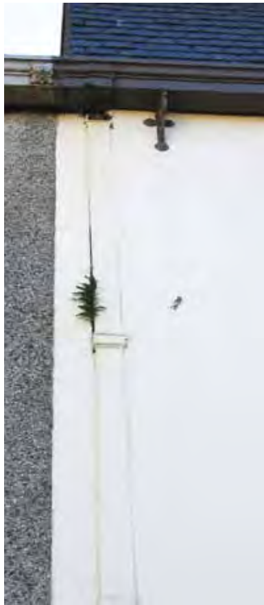
Fig. 209 Downpipe which has been installed flush with the building façade
