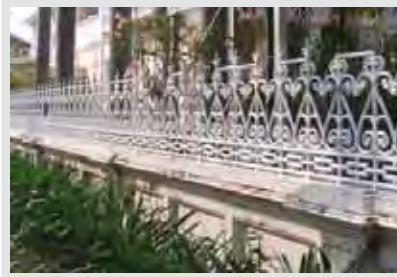
Fig. 309, Leith Street, George Town, Penang, Malaysia, Made by Walter MacFarlane & Co, pattern number 213 Image courtesy of The Scottish Ironwork Foundation
