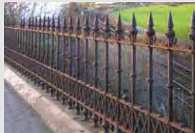
Fig. 304, Rail Bridge Ramps, Magdalene Green, Dundee Made by Walter MacFarlane & Co, pattern number 464 Image courtesy of The Scottish Ironwork Foundation
