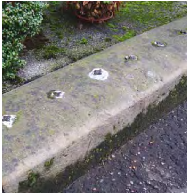
Fig. 33 Railing stubs in the tops of cope stones are a common sight in Scotland
