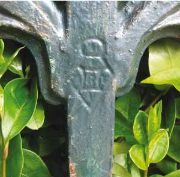
Fig. 99 Railing 26, this date stamp is hidden beneath layers of paint
