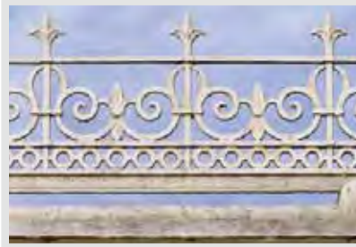
Fig. 282, Valley Gardens and Montpellier Gardens, Harrogate, North Yorkshire Unmarked but probably made by Walter MacFarlane & Co, pattern number 145. This example shows the design being used as cresting. Image courtesy of The Scottish Ironwork Foundation
