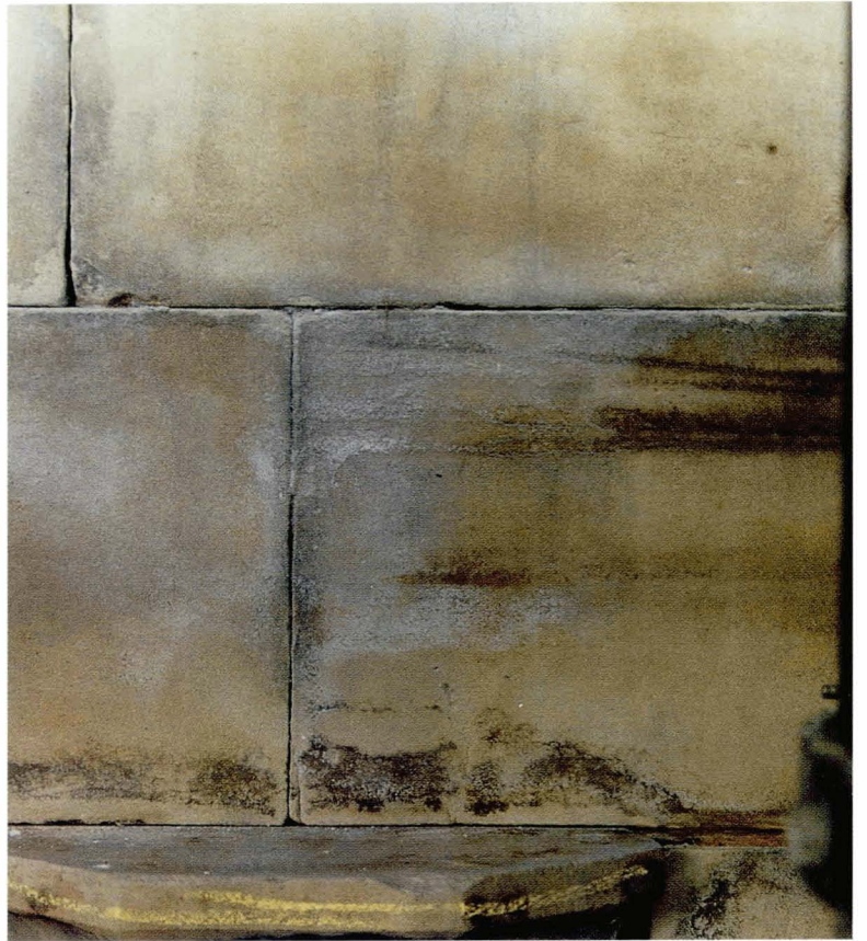
Plate 5.6 Efflorescence shortly after cleaning.
