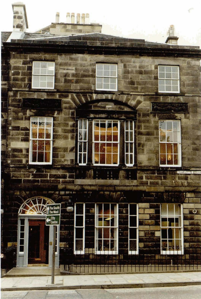
Plate 3.17 Soiled sandstone facade.
