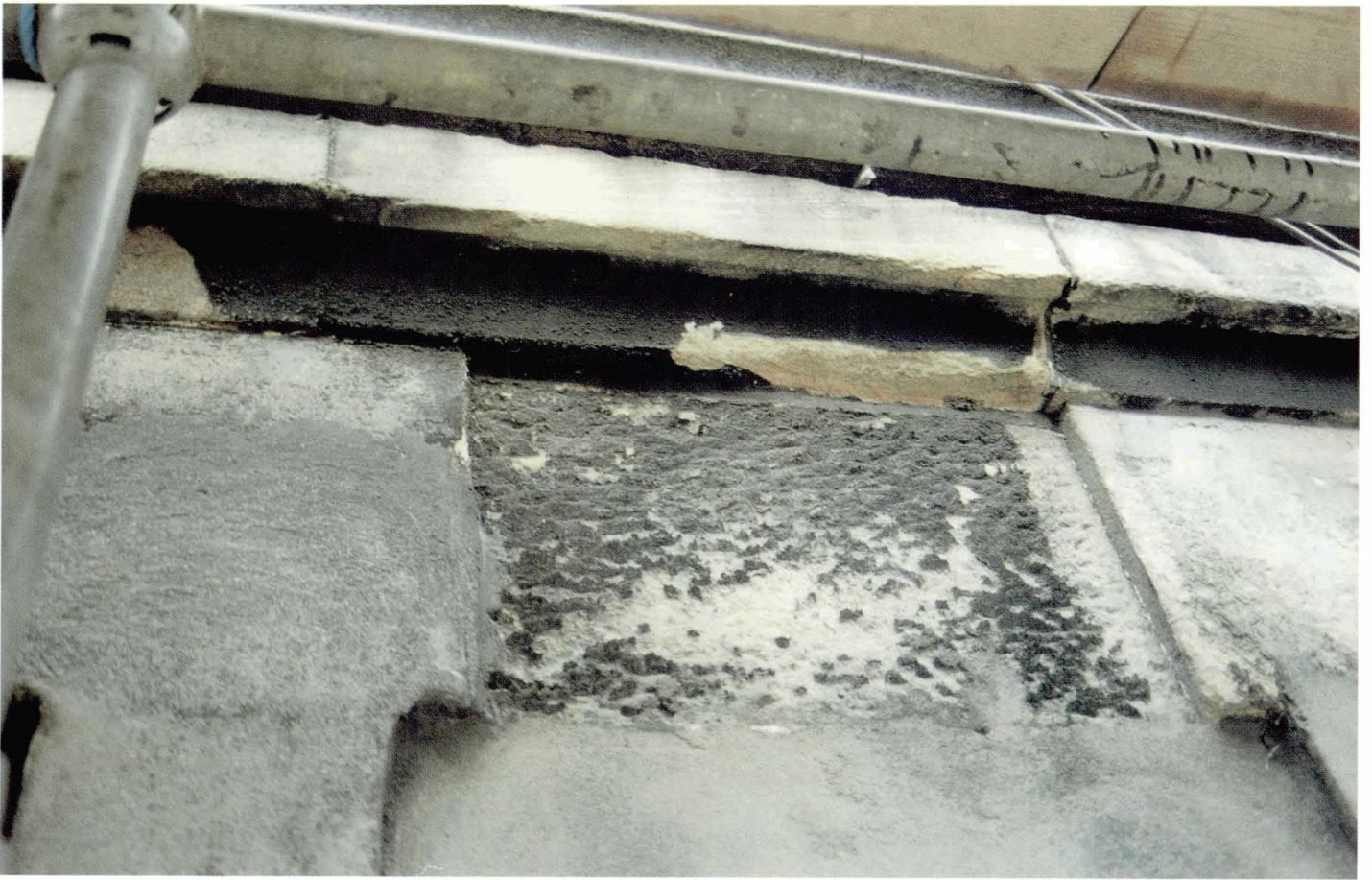
Plate 4.7 Decayed sandstone with spalling, soiled surfaces before cleaning.
