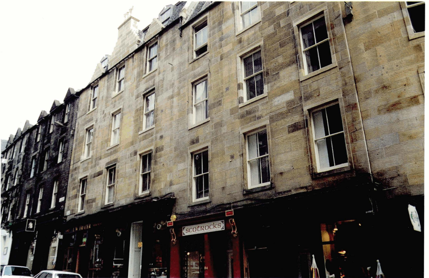
Plate 4.22 Sandstone building cleaned by low pressure grit blasting. Some soiling is still visible on the facade.
