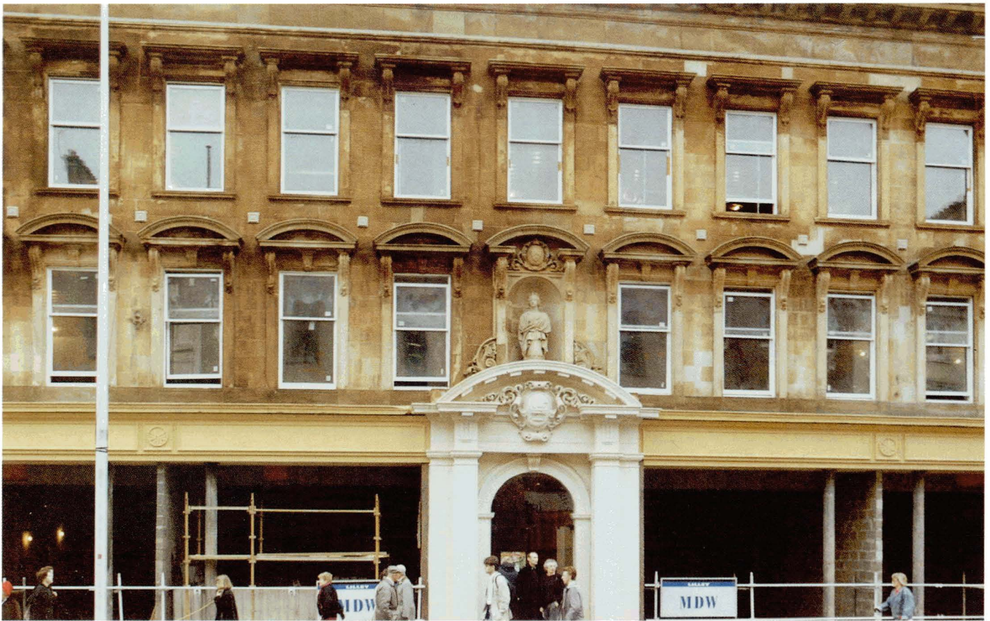
Plate 5.2 Staining caused by the migration of iron from within the stone to the stone surface.
