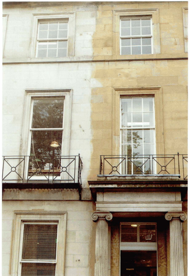
Plate 3.14 Differences in the colour of individual stones in a facade can be detected after having been cleaned by two different methods.
