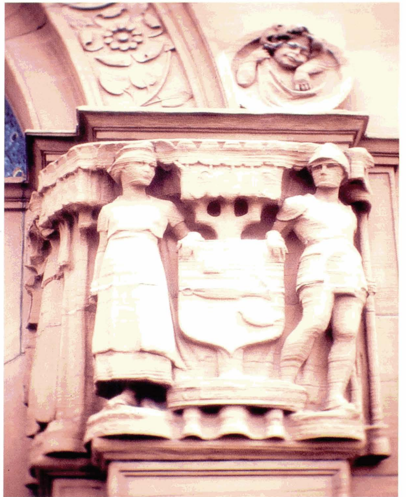
Plate 4.4 Damage to detailing caused by dry grit blasting.
