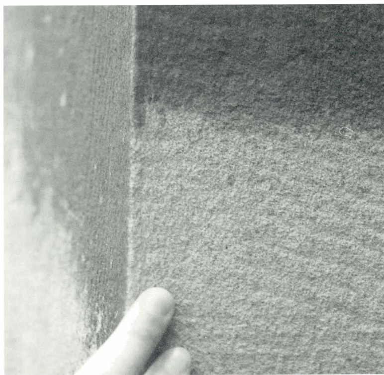
Plate 4.17 Sandstone partially cleaned using low pressure grit blasting. No apparent erosion along edge of the stone.
