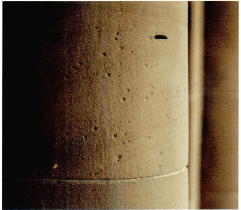
Plate 5.1 Pitting of a sandstone surface caused by removal of calcite by acid cleaning.
