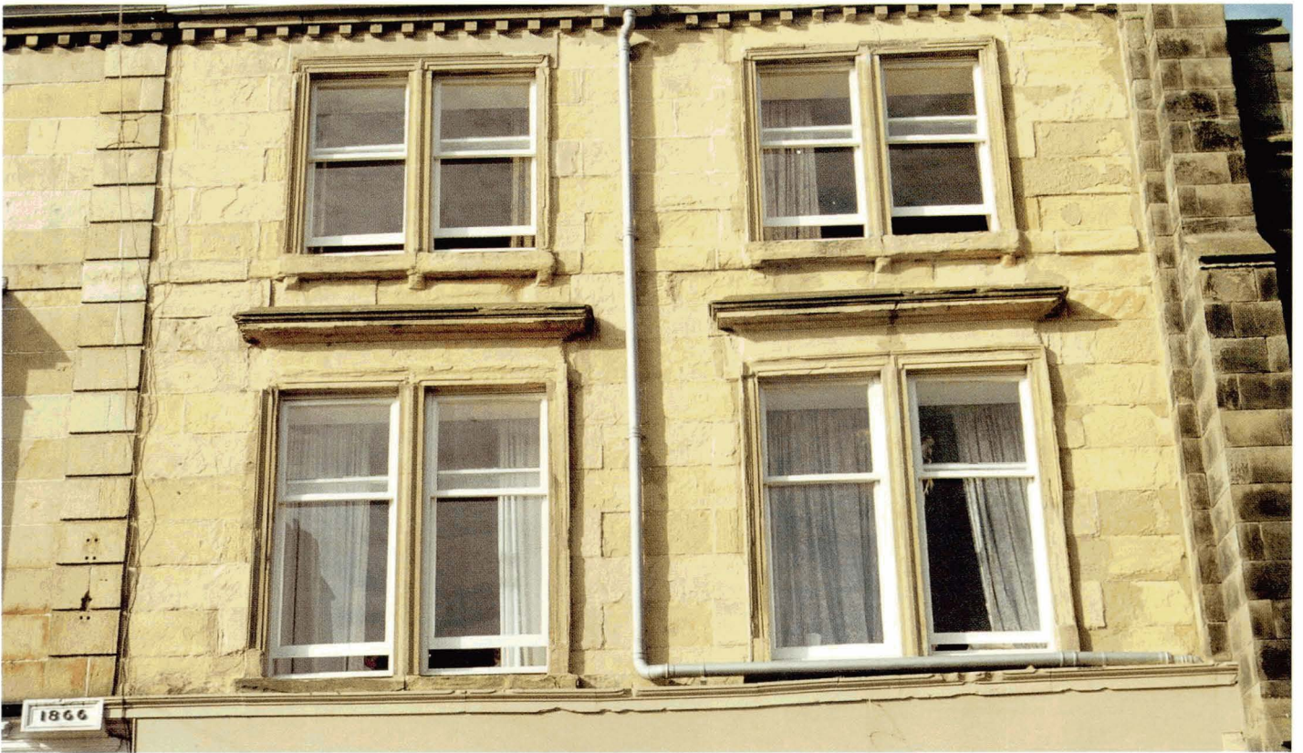
Plate 4.3 Damage to a sandstone building caused by dry grit blasting.
