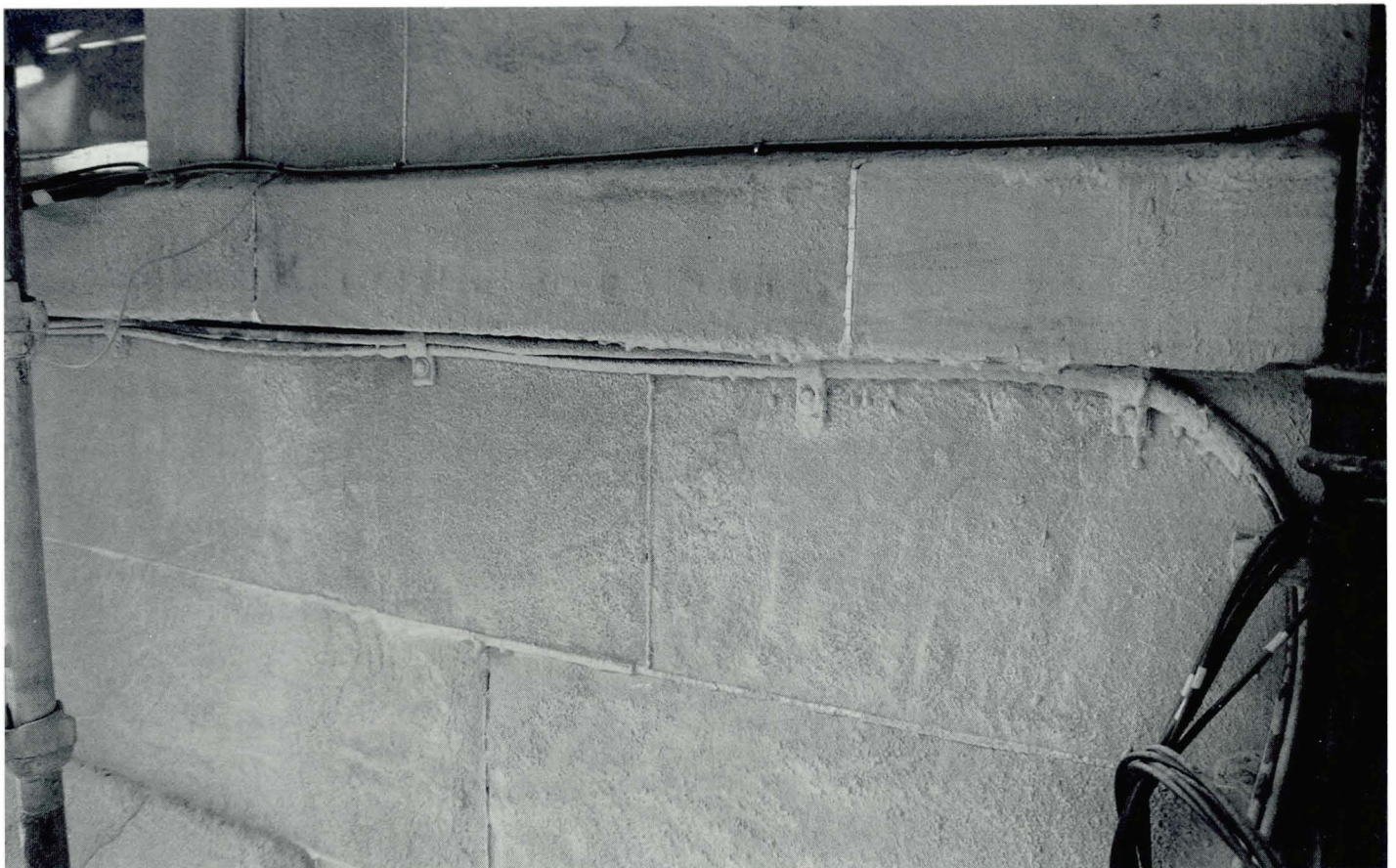
Plate 4.12 After cleaning (same area as above). Following cleaning virtually all soiling has been removed, but there is a thick crusting of loose dust and debris from wet grit blasting coating the surface.
