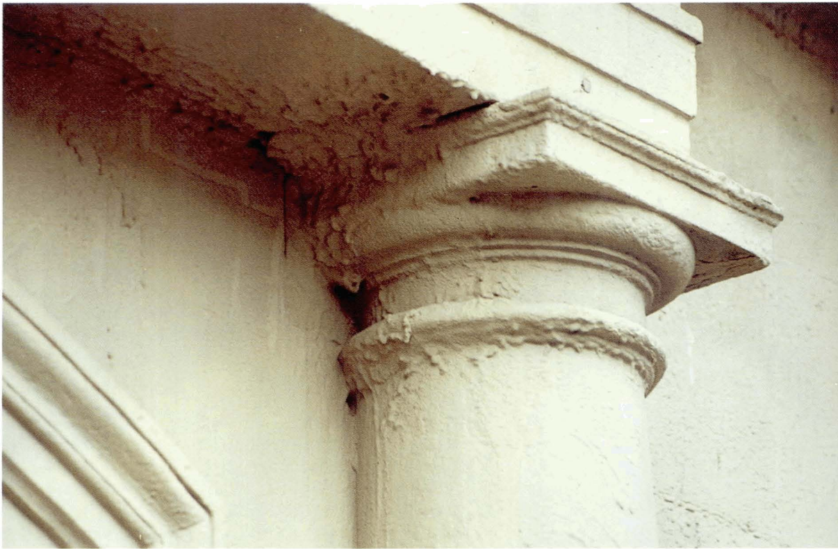
Plate 4.14 Hardened rock dust/grit deposited on this stonework as a result of wet grit blasting is disfiguring the architectural detailing.
