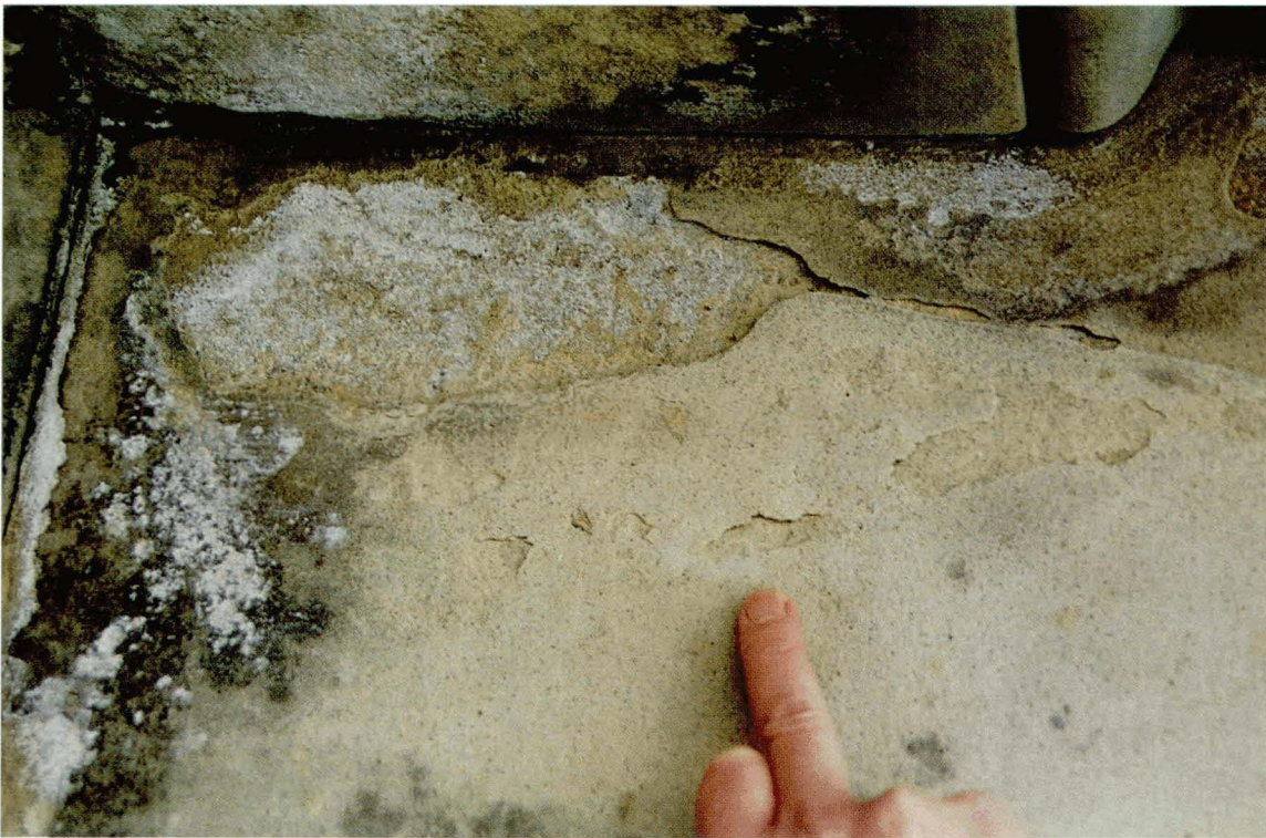
Plate 5.8 Efflorescences exacerbate the problem of contour scaling.
