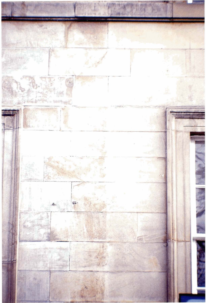
Plate 5.9 The effect of two different chemical cleaning regimes on a sandstone facade.
