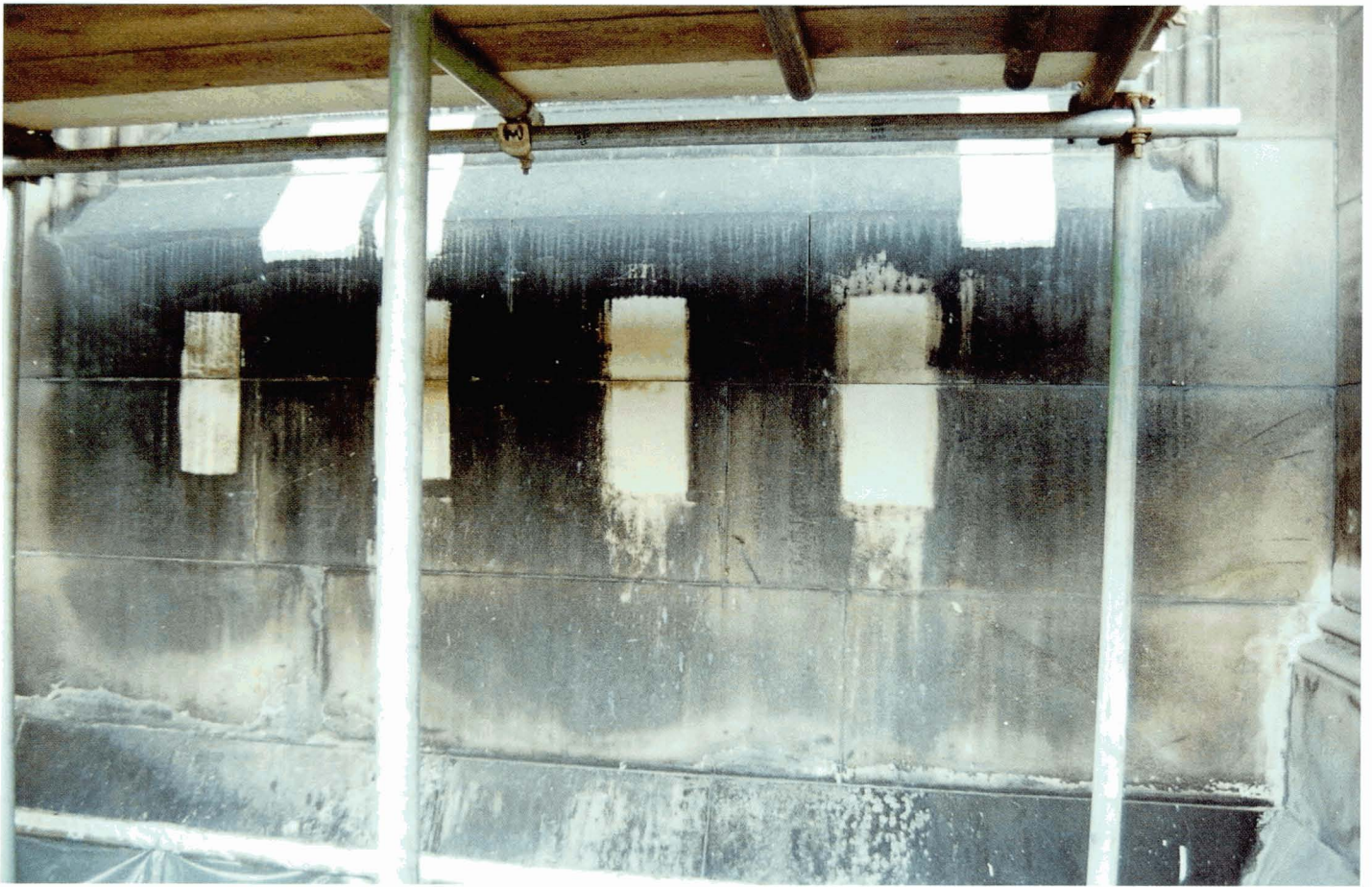
Plate 5.12 Chemical cleaning test panels. Heavily soiled sloping area has also been test cleaned.
