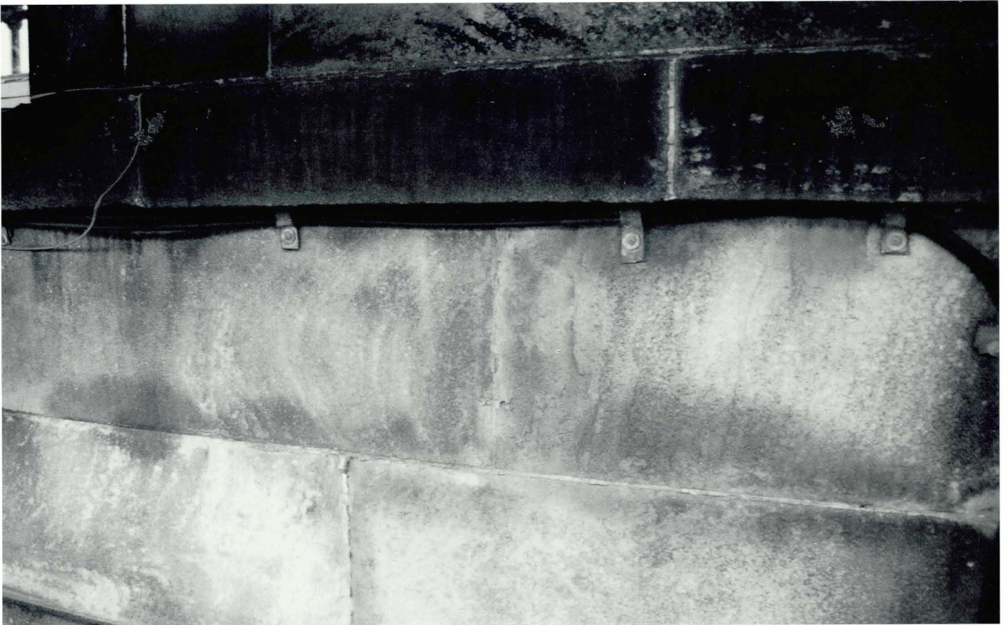
Plate 4.11 Heavily soiled sandstone prior to wet blast cleaning. There is severe soiling on the exposed ledge and typical soiling of smooth, vertical stonework under the ledge.
