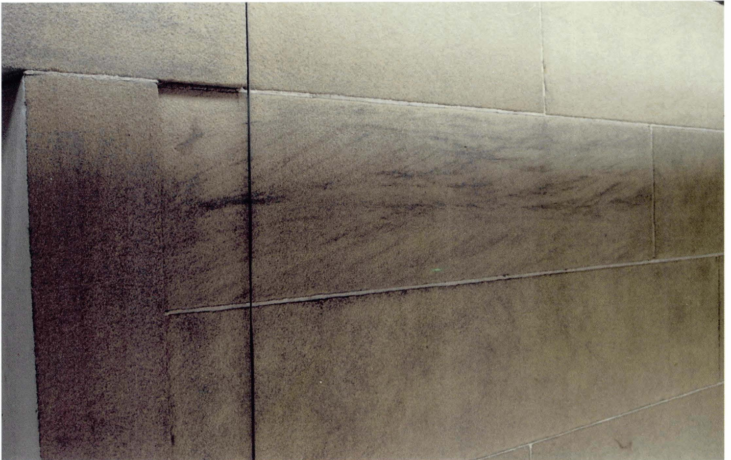
Plate 4.2 After cleaning (same area as above). Most soiling has been removed. Some ingrained soiling remains.
