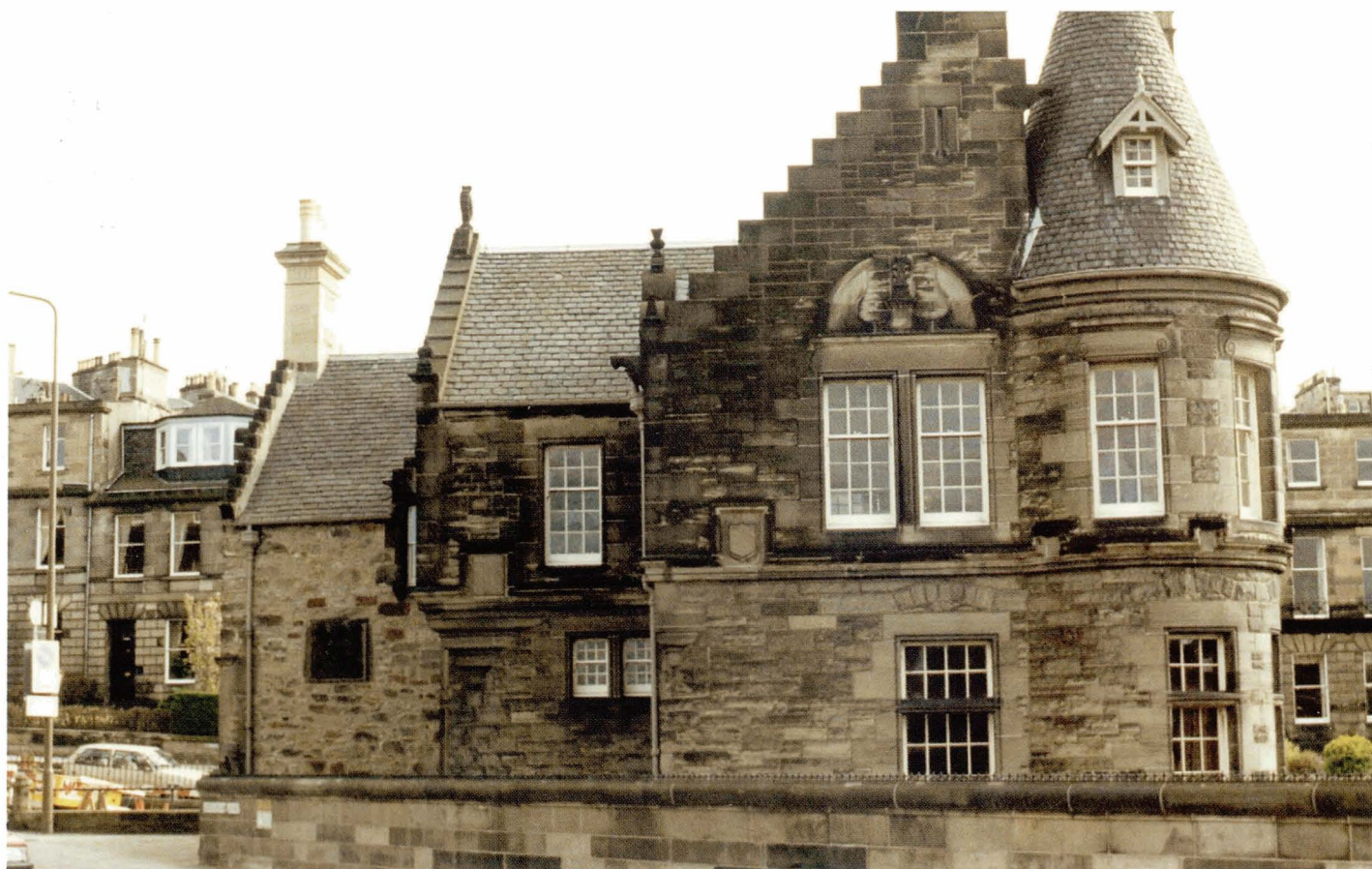
Plate 3.26 This building has soiled at different rates across its facade. The upper gable end is heavily soiled, obscuring stone colour and detail. Lower sections of the building are less heavily soiled and are aesthetically more pleasing.
