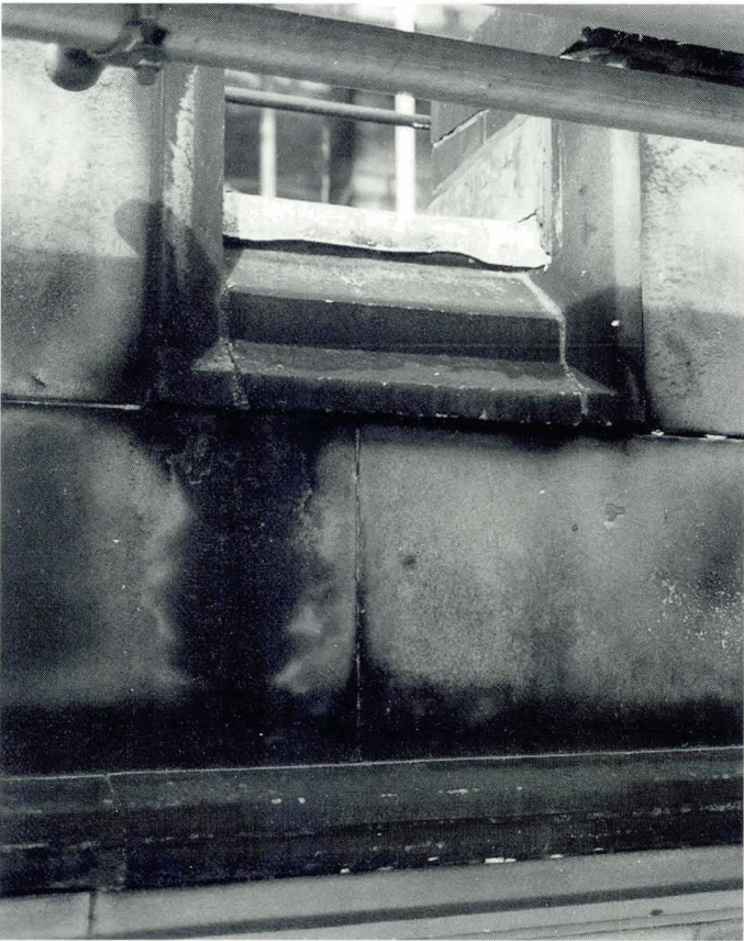
Plate 5.23 Before chemical cleaning. Intense soiling in areas of water run-off.
