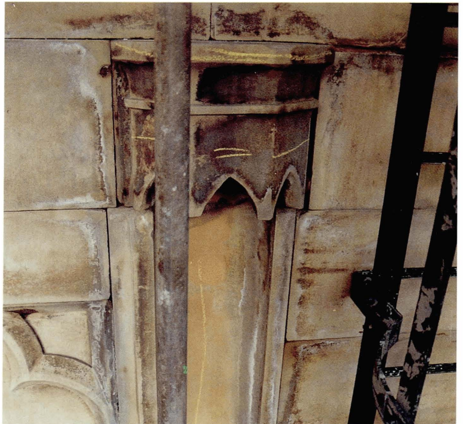
Plate 5.5 Efflorescences following chemical cleaning occurring in the same places as iron staining and residual soiling. These are areas where capillary forces during wetting/drying cycles have concentrated soluble materials at the surface.
