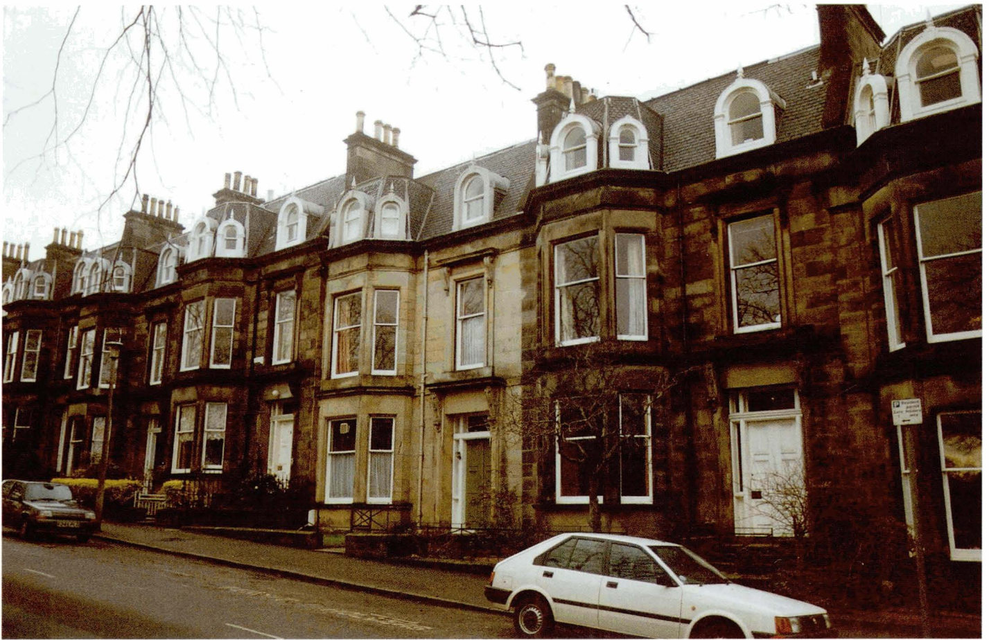
Plate 3.2 The cleaning of the single facade has compromised the unity of this terrace.
