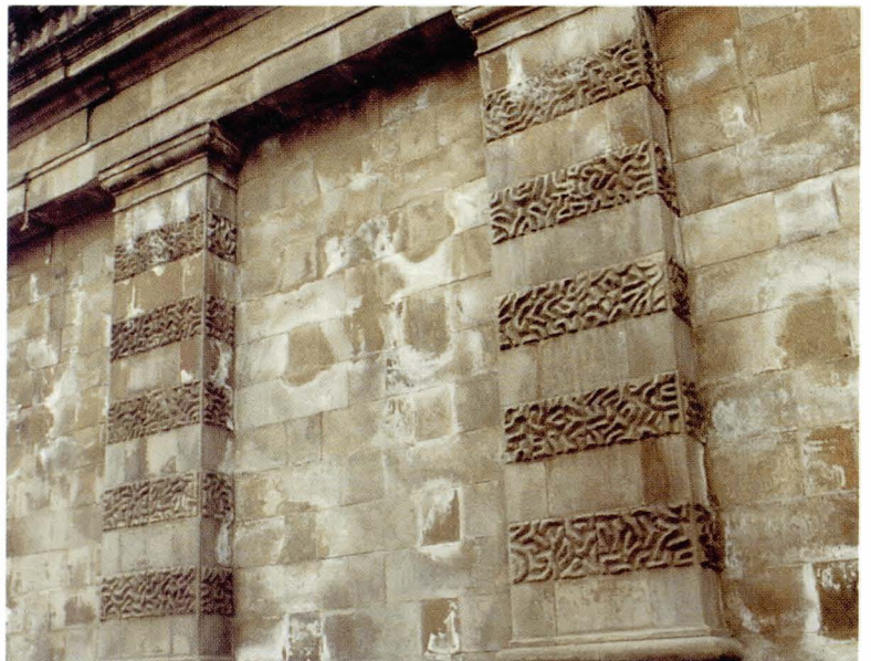
Plate 5.3 Extensive efflorescences following chemical cleaning.
