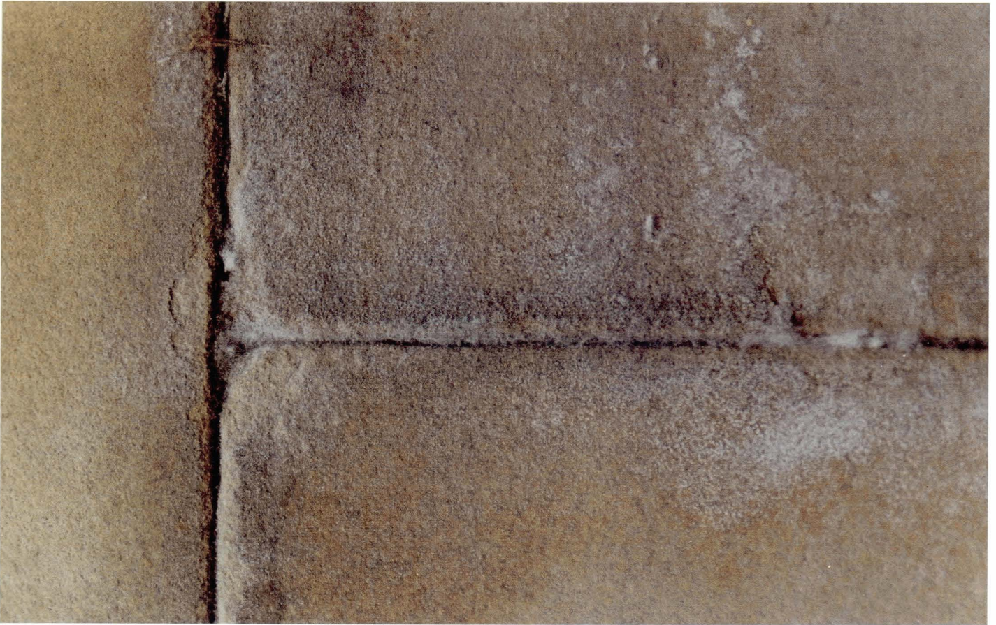
Plate 5.4 Intense efflorescence of sodium sulphate around an open joint after chemical cleaning.
