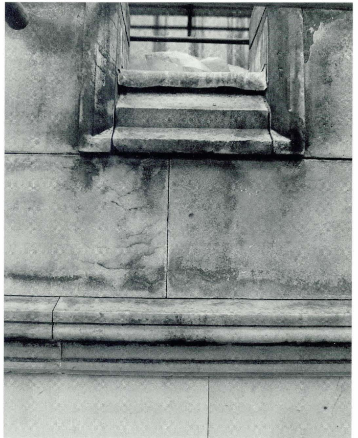
Plate 5.24 After chemical cleaning (same area as plate 5.23). Some ingrained soiling remains in the area affected by water run-off.
