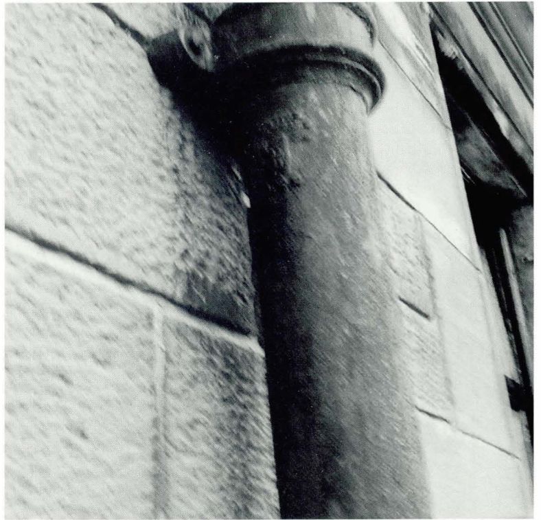
Plate 5.20 After chemical cleaning. Soiling retained behind a drainage pipe where access by cleaning chemicals was difficult.
