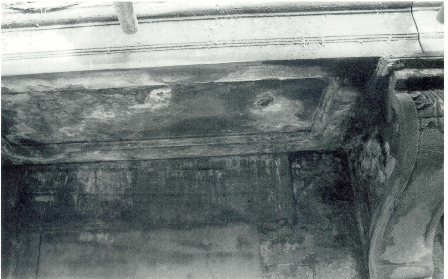
Plate 5.18 Area of sandstone before cleaning. Efflorescence and soiling where stone remained damp for long periods due to a leaking pipe.
