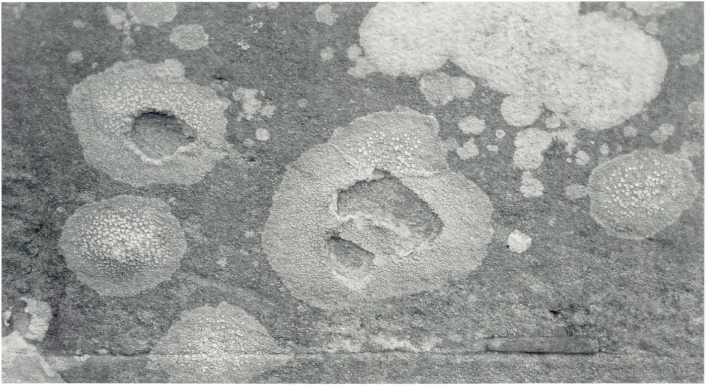
Plate 2.3 Lichen causing blistering and decay on a stone surface.
