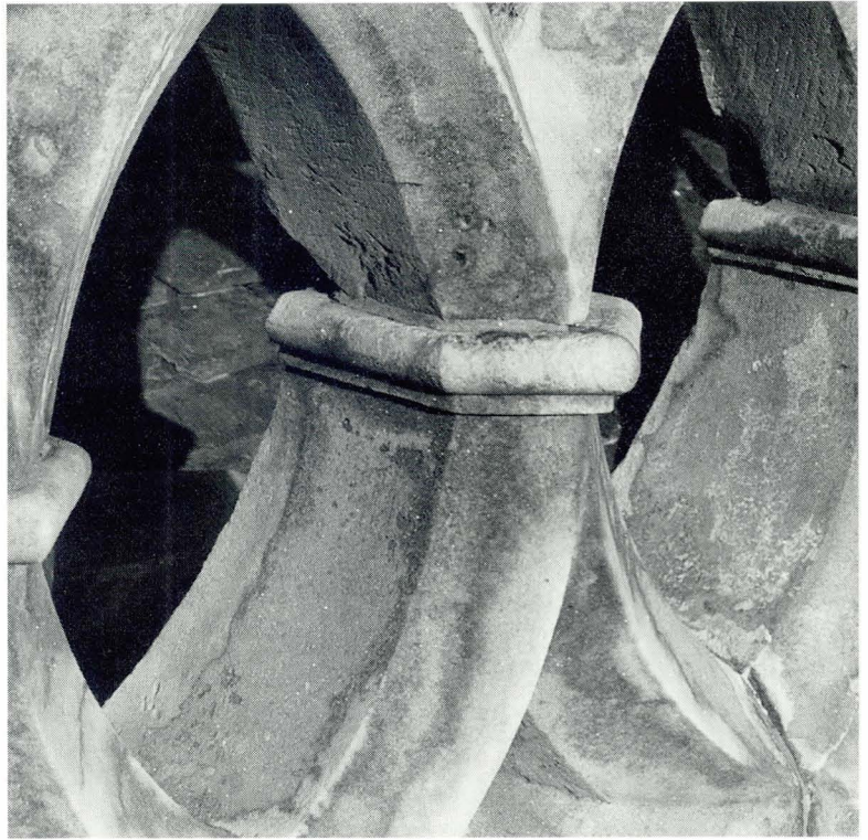
Plate 5.25 After chemical cleaning. Part of this balustrade shows deeply ingrained soiling in an area of very exposed stonework. Such soiling is very difficult or impossible to remove without excessive damage to the fabric of the stone.
