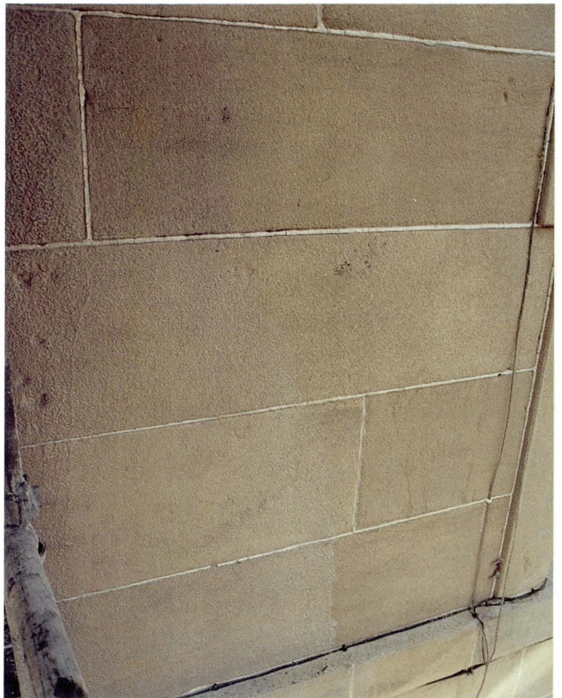
Plate 4.15 Debris wash over on to the next facade after wet grit blasting.
