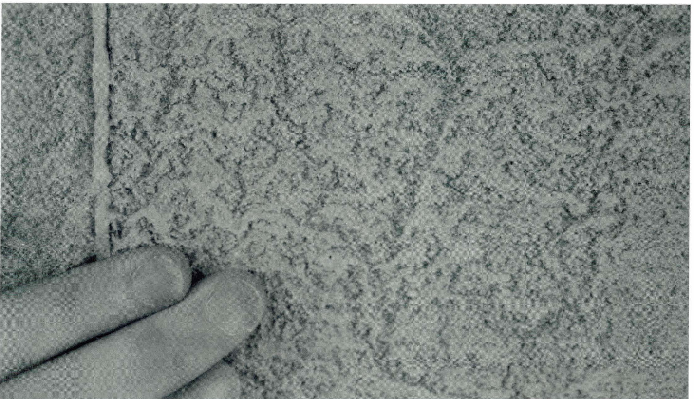
Plate 4.13 Dust and debris coating the sandstone surface after wet grit blasting.
