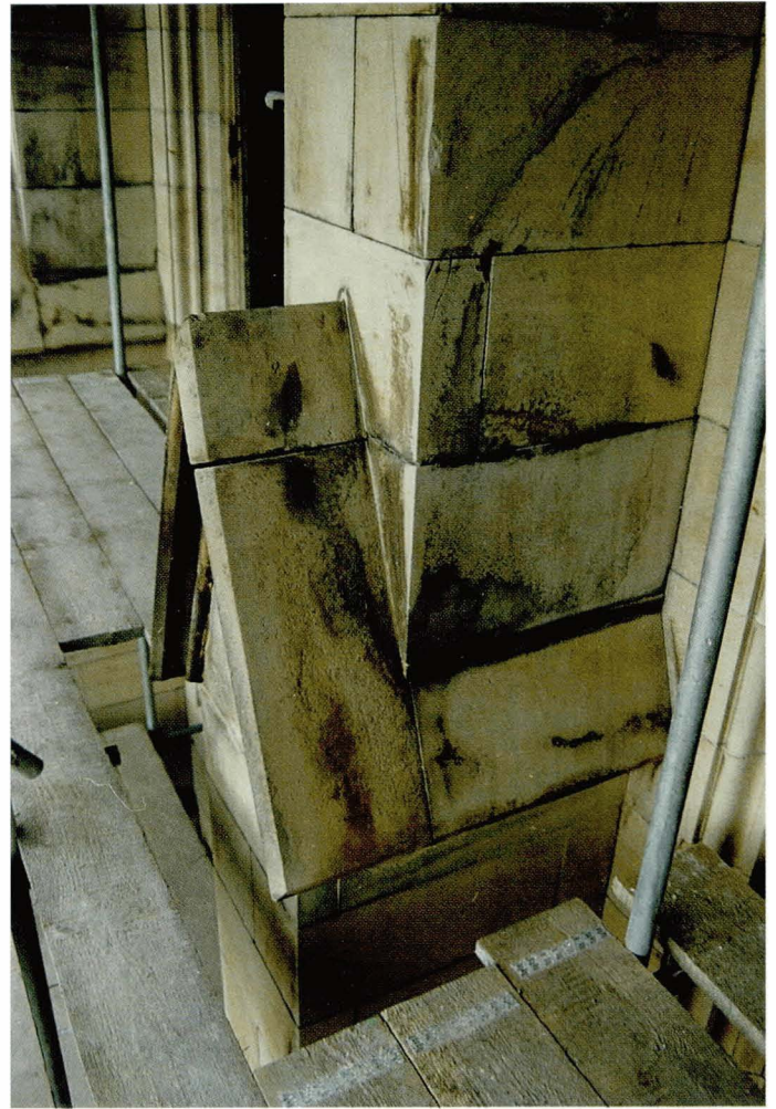
Plate 5.11 After cleaning (same area as Plate 5.10). Note residual soiling reflects the pattern of organic growths prior to cleaning. Areas affected by biological growths are cleaner than those which were unaffected by biological growths.
