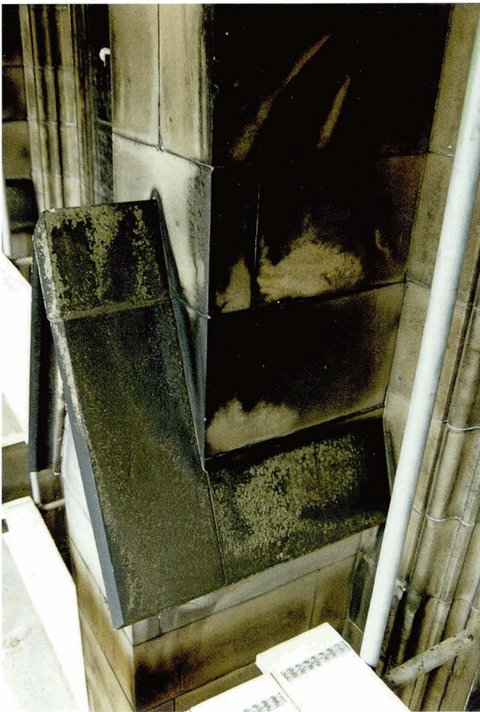
Plate 5.10 Before cleaning. Typical soiling pattern of sloping stonework. The higher moisture content of the exposed stone has attracted a high degree of soiling and algal growth.
