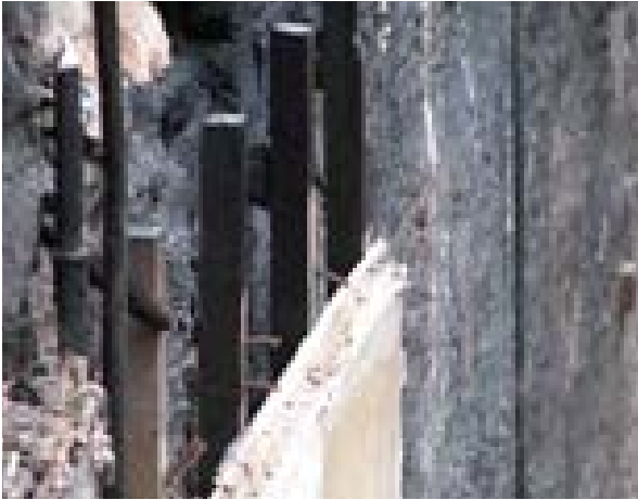
Illus 17 This post-fire image from a category A listed building clearly illustrates the gap that exists behind traditional lath and plaster walling (essential for ventilation)
