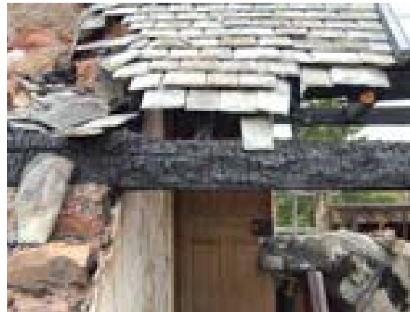
Illus 15 This compartment wall was compromised by a structural roof timber travelling through it
