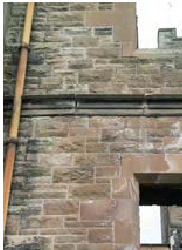
Illus 37 Expansion of the internal beams has applied pressure to the external walls, causing large cracks along a section of the stringcourse
