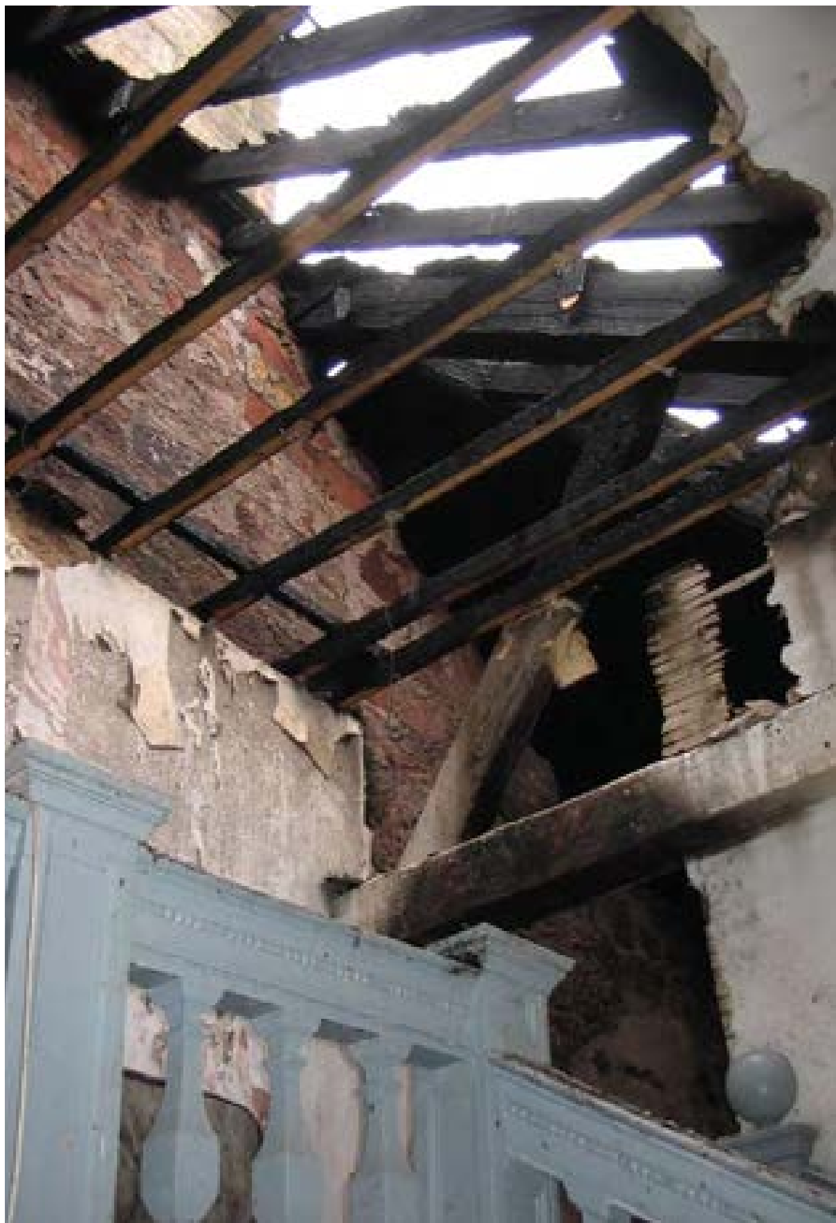
Illus 42 In this category B listed building, sub-divided into flats, a fire is believed to have been caused by faulty electrical services in the attic. Early detection restricted damage to the roof
