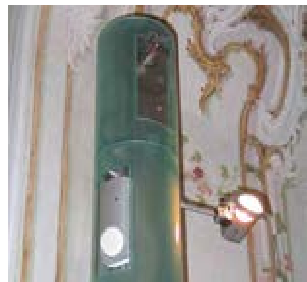
Illus 56 Reversibility - In this highly decorated Austrian palace interior, a contemporarily detailed floor fixed 'pole' houses a sprinkler head, electrical services and emergency lighting – thus providing an innovative and reversible solution avoiding damage to historic wall finishes which conventional installations give rise to © Stewart Kidd
