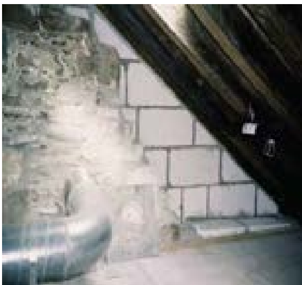
Illus 47 Examples of fire stopping to improve compartmentation © Stewart Kidd
