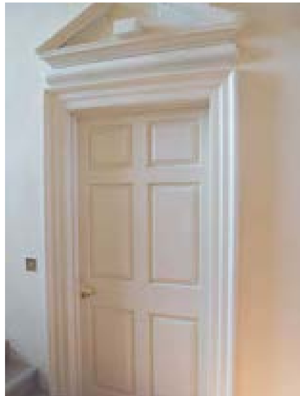
Illus 20 Original Georgian doors whose retention was facilitated by partial sprinklering of the property
