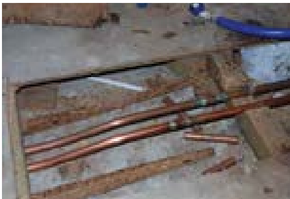
Illus 29 When notching structural elements, such as floor timbers, for the installation of services fire stopping must also be addressed © Stewart Kidd
