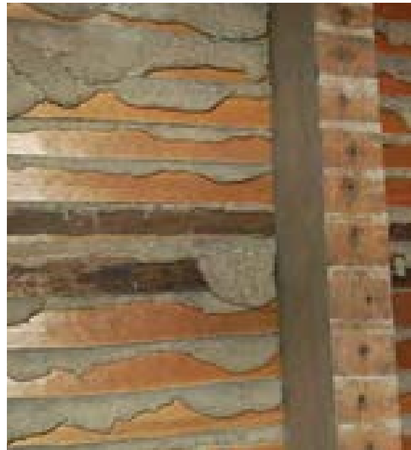
Illus 35 The back of traditional lath and plaster showing the wooden lattice structure that provides a key for the applied plaster
