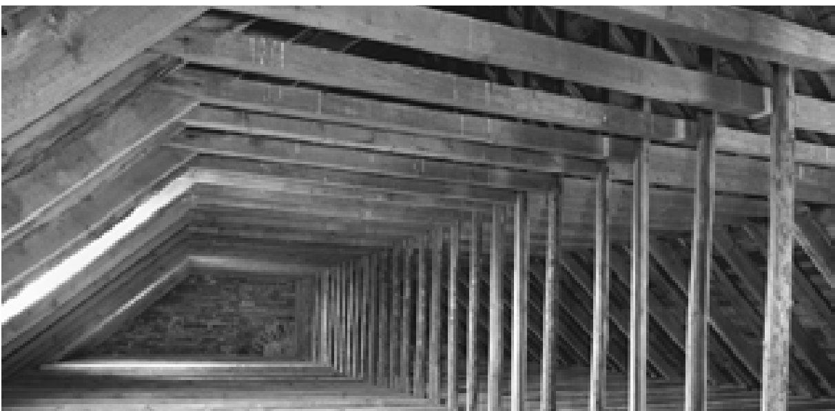
Illus 26 Large attic spaces with no compartmentation are common and facilitate the rapid spread of fire © Crown Copyright: RCAHMS. Licensor www.rcahms.gov.uk
