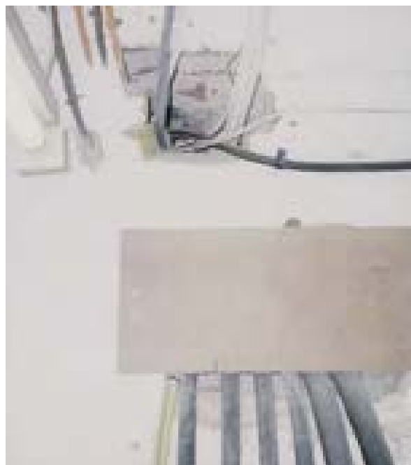
Illus 14 The haphazard installation of services can compromise a compartment wall © Stewart Kidd
