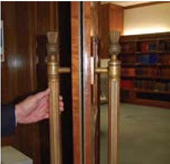
Illus 22 In the upgrading of these double doors in a reading room at the National Library of Scotland, cold smoke seals were run along the stile
