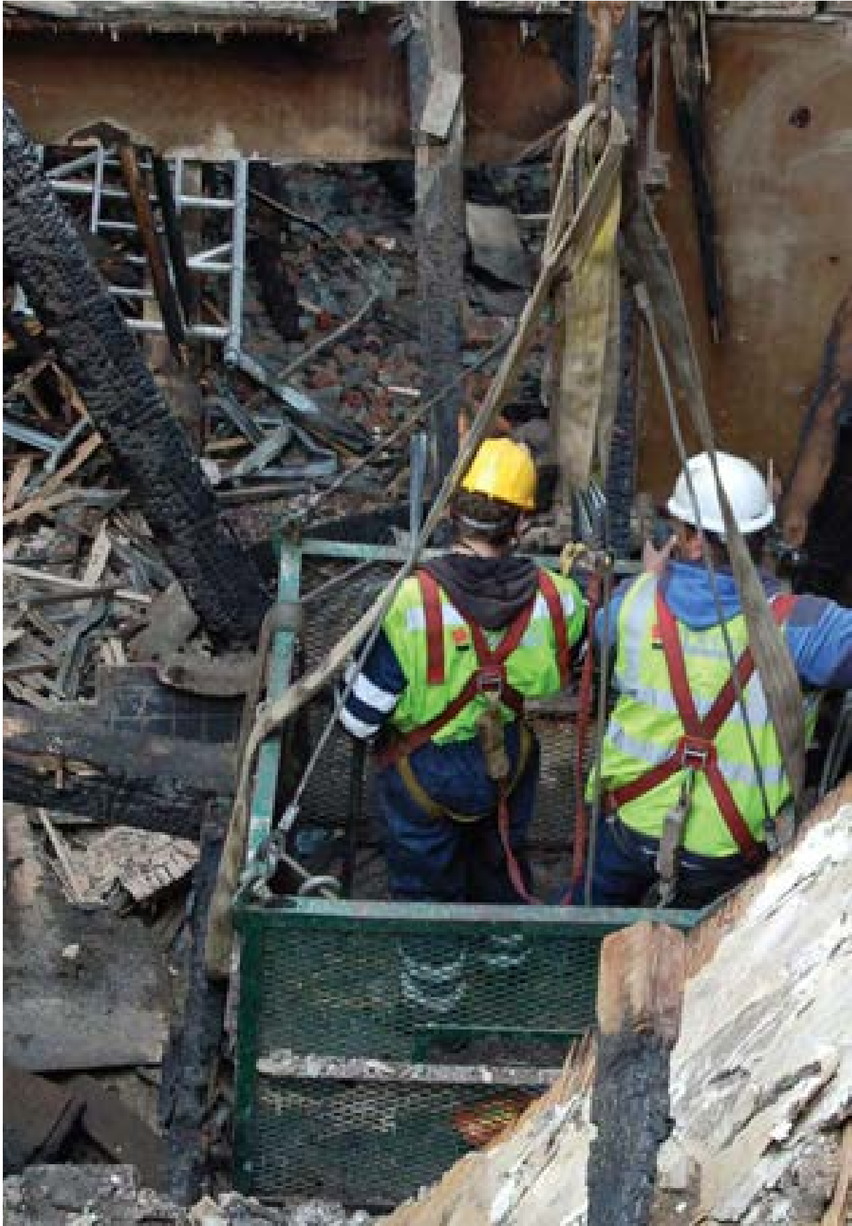
Illus 51 The sensitive introduction of fire measures into traditional buildings can help prevent their destruction. This large country house, category A listed, has been totally devastated and a recovery firm has been mobilised to remove the debris
