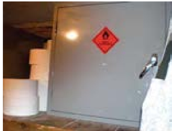
Illus 64 To control an identified risk, flammable liquids should be stored in a proper flammable liquid storage cabinet © Stewart Kidd
