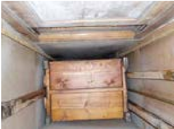
Illus 28 Dumb waiters, often disused, provide a large hidden passage that can aid the rapid travel of fire between floors © Stewart Kidd
