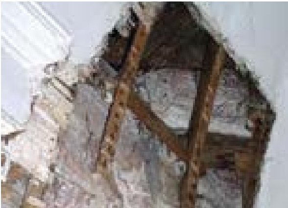
Illus 25 Substantial hidden void above a coombed ceiling in a traditionally constructed building. Voids can aggravate fire spread and should be considered when assessing risk
