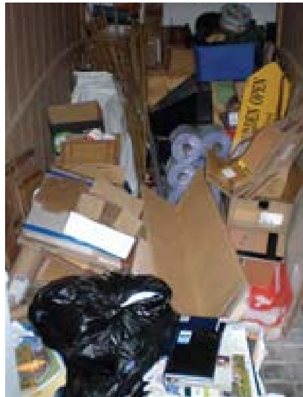
Illus 41 In this heritage visitor attraction, this storage area presents a fire hazard
