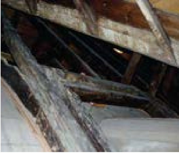
Illus 24 Attic roof void with the additional fuel loading of a timber vaulted dome, Culross Palace, Fife © Stewart Kidd (by kind permission of the National Trust for Scotland)
