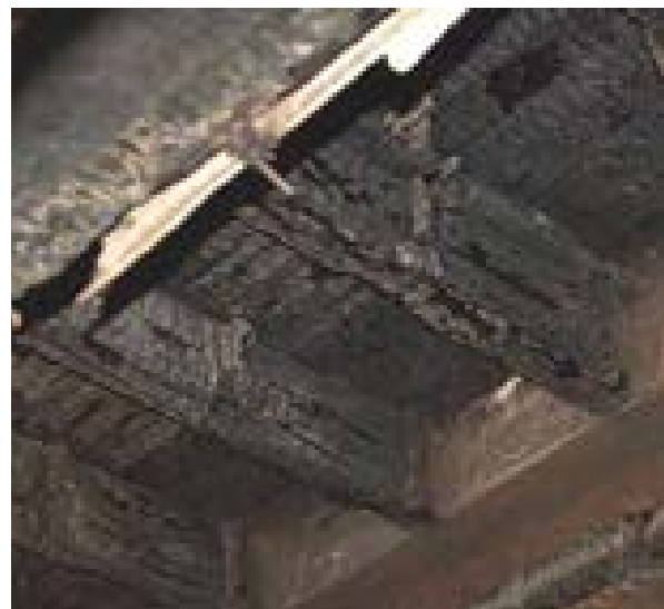
Illus 33 Due to their thickness structural ceiling timbers can burn slowly and perform their function for a long period
