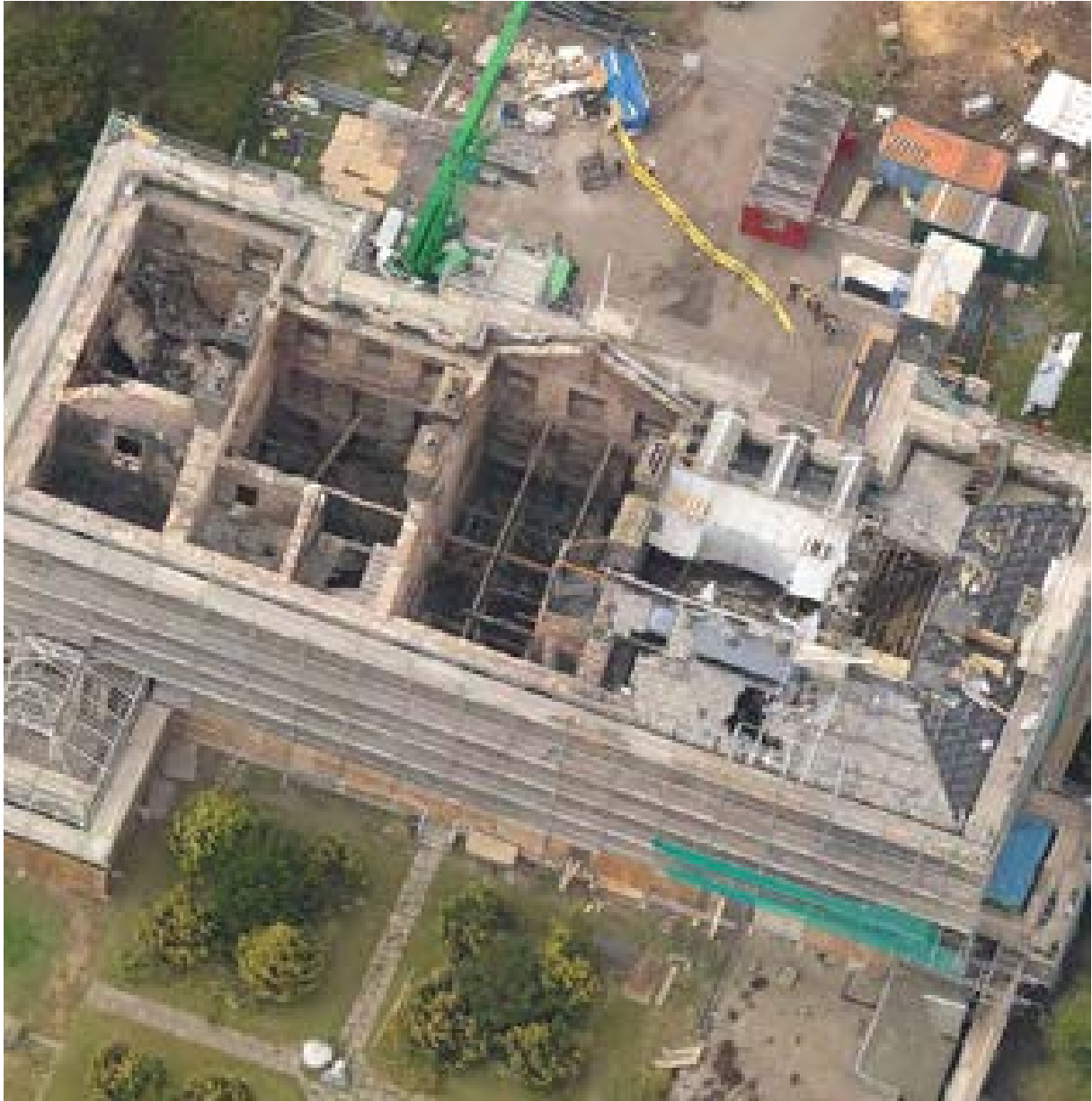
Illus 13 Aerial view of Leslie House, a category A listed mansion, that was severely damaged by fire during sub-division to luxury flats © Crown Copyright: RCAHMS. Licensor www.rahms.gov.uk
