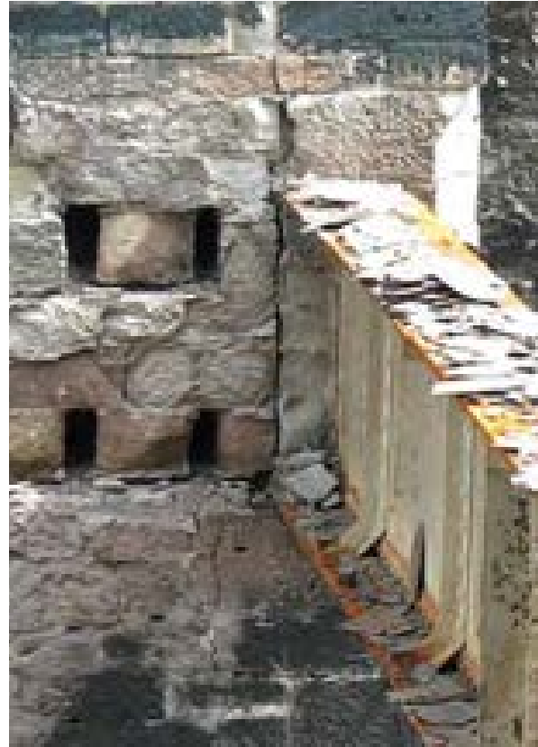
Illus 36 During a fire, expansion of the girders has caused movement in the walls of this listed property
