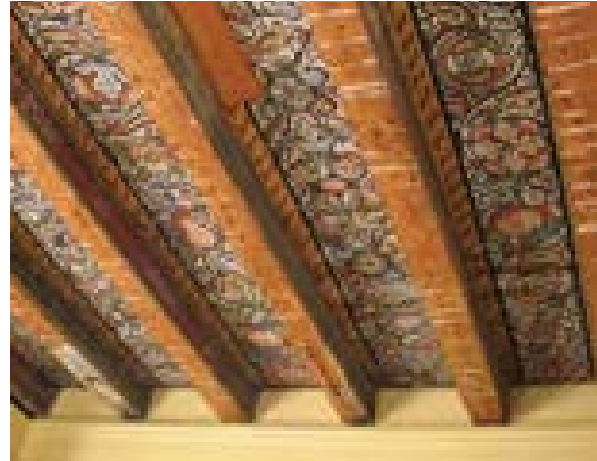
Illus 18 A traditional technique in early buildings was to decoratively paint the underside of floorboards. Although this offers little fire resistance, where such decoration survives it is important to retain it
