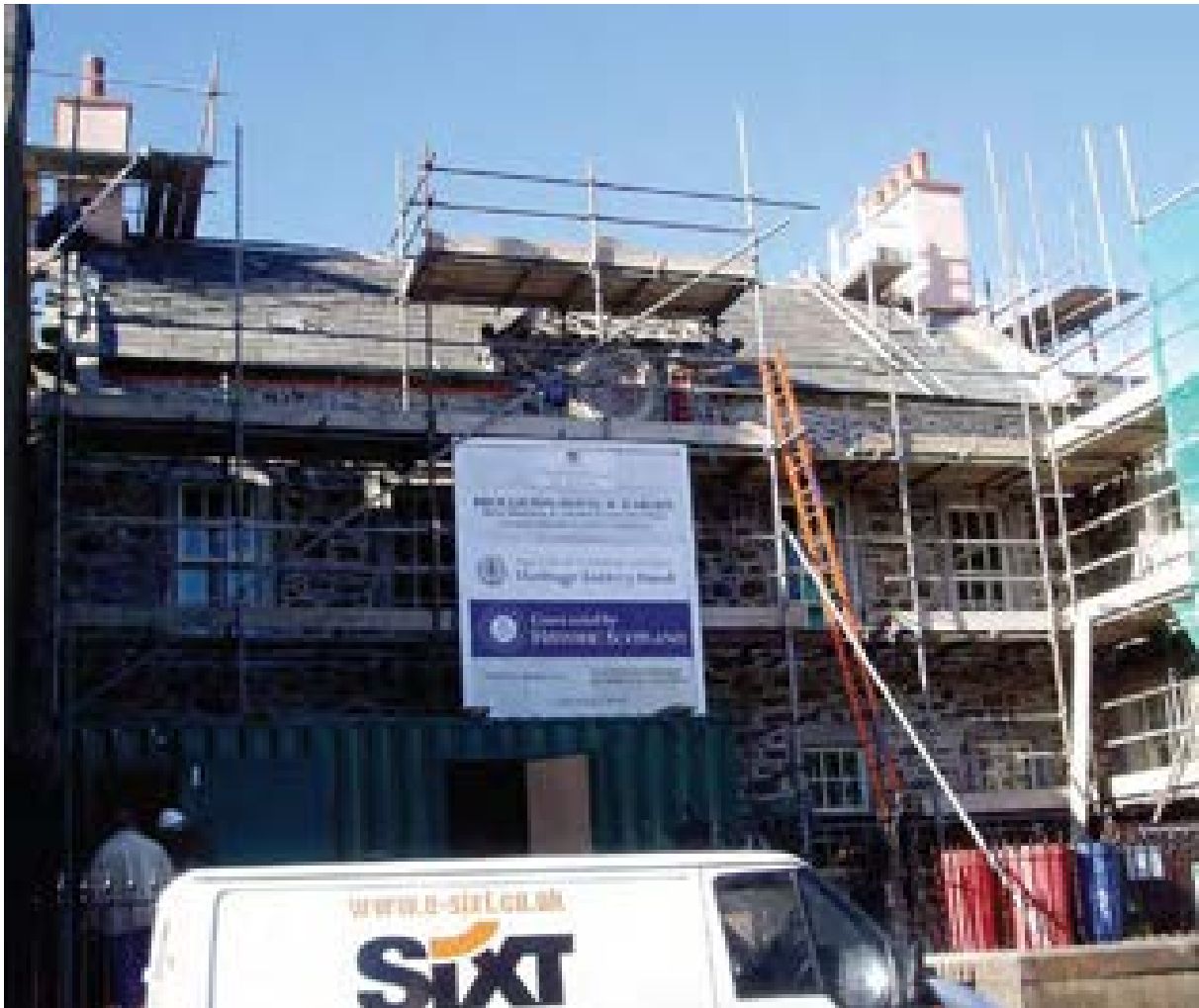
Illus 49 Statistics suggest that traditional buildings are at greater fire risk during construction works and consequently additional controls and procedures should be implemented to minimise risk © Stewart Kidd
