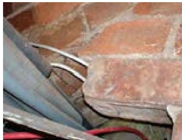
Illus 16 The lack of stopping around service installations has adversely affected the compartmentation
