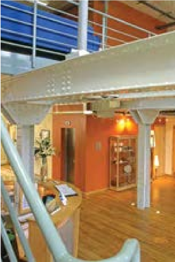
Illus 38 In industrial conversions, such as this pictured, it is common for the metal elements to be coated with intumescent paints. This is the Scottish Borders Enterprise business gateway in Ettrick Mill, Selkirk, 1836-1850, where steel was inserted around ground floor machinery in the early 20th century. The conversion lifted part of a timber floor to make a light reception area
