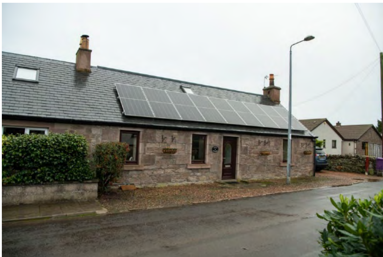
Figure 153: Terraced cottages, Watson Street, Letham, Angus. The flagstone roof has been lost.
