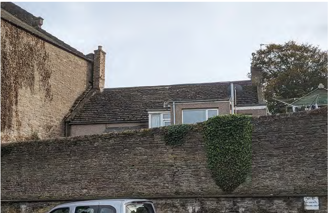
Figure 110: 2 St James Road, Forfar, Angus. Flagstone is present on the rear elevation.
