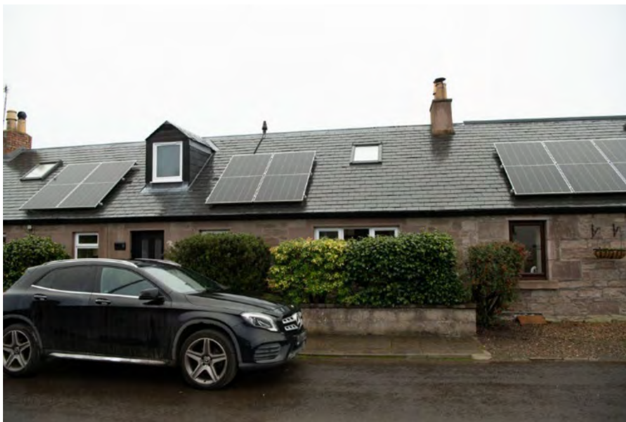
Figure 152: Terraced cottages, Watson Street, Letham, Angus. The flagstone roof has been lost.
