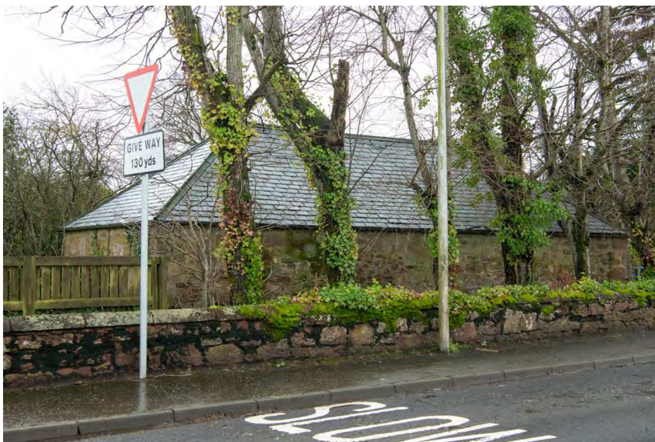
Figure 145: Weavers Cottages, Kirriemuir, Angus. The flagstone roof has been lost.
