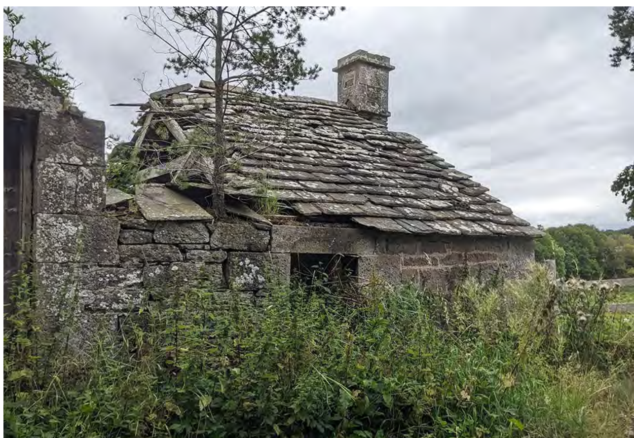
Figure 044: Partial roof remaining on derelict Kincaldrum Mill House, Angus. © Sara Carruthers.
