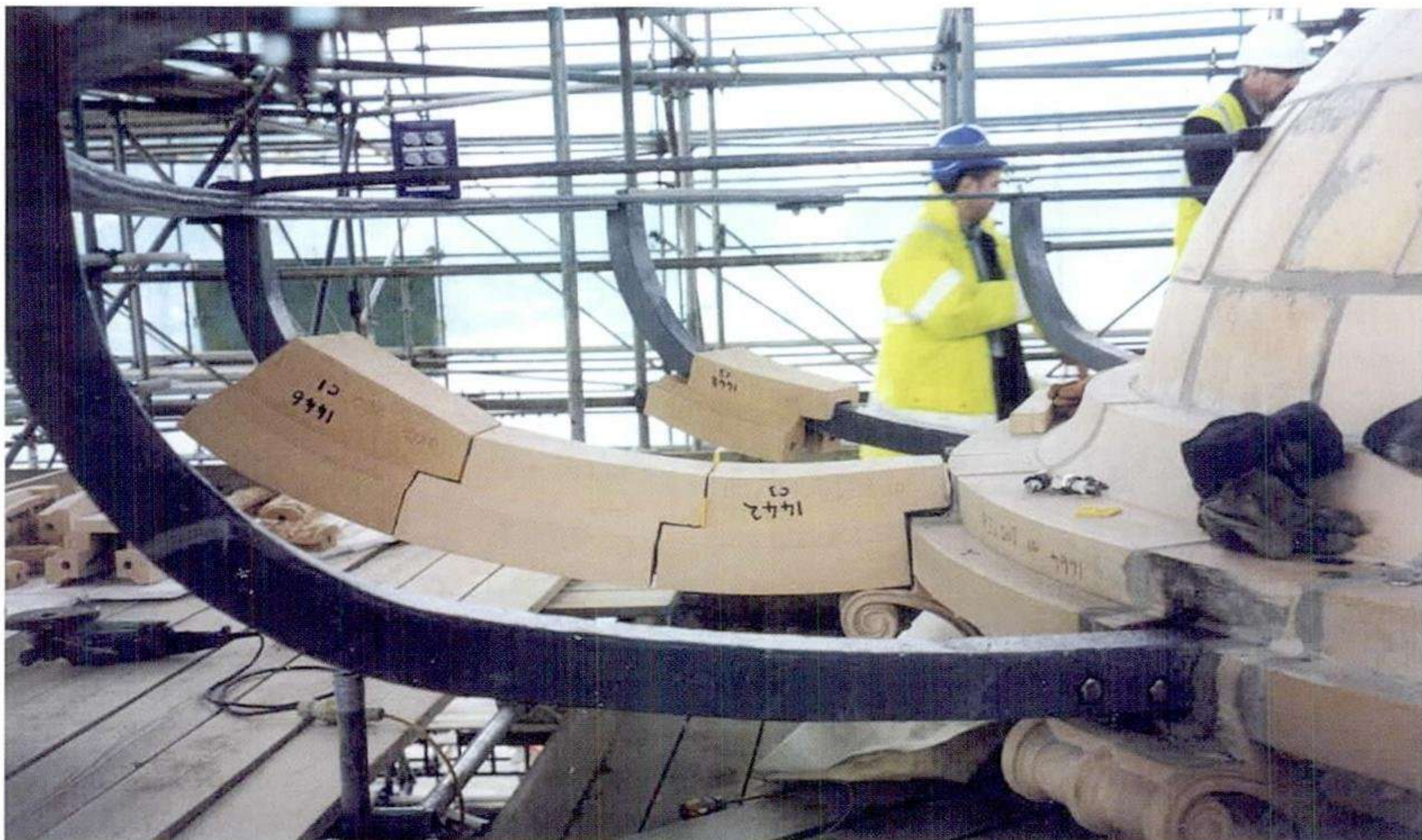
Reconstruction of the cantilevered basin began with the saddle blocks to the structural arms.
