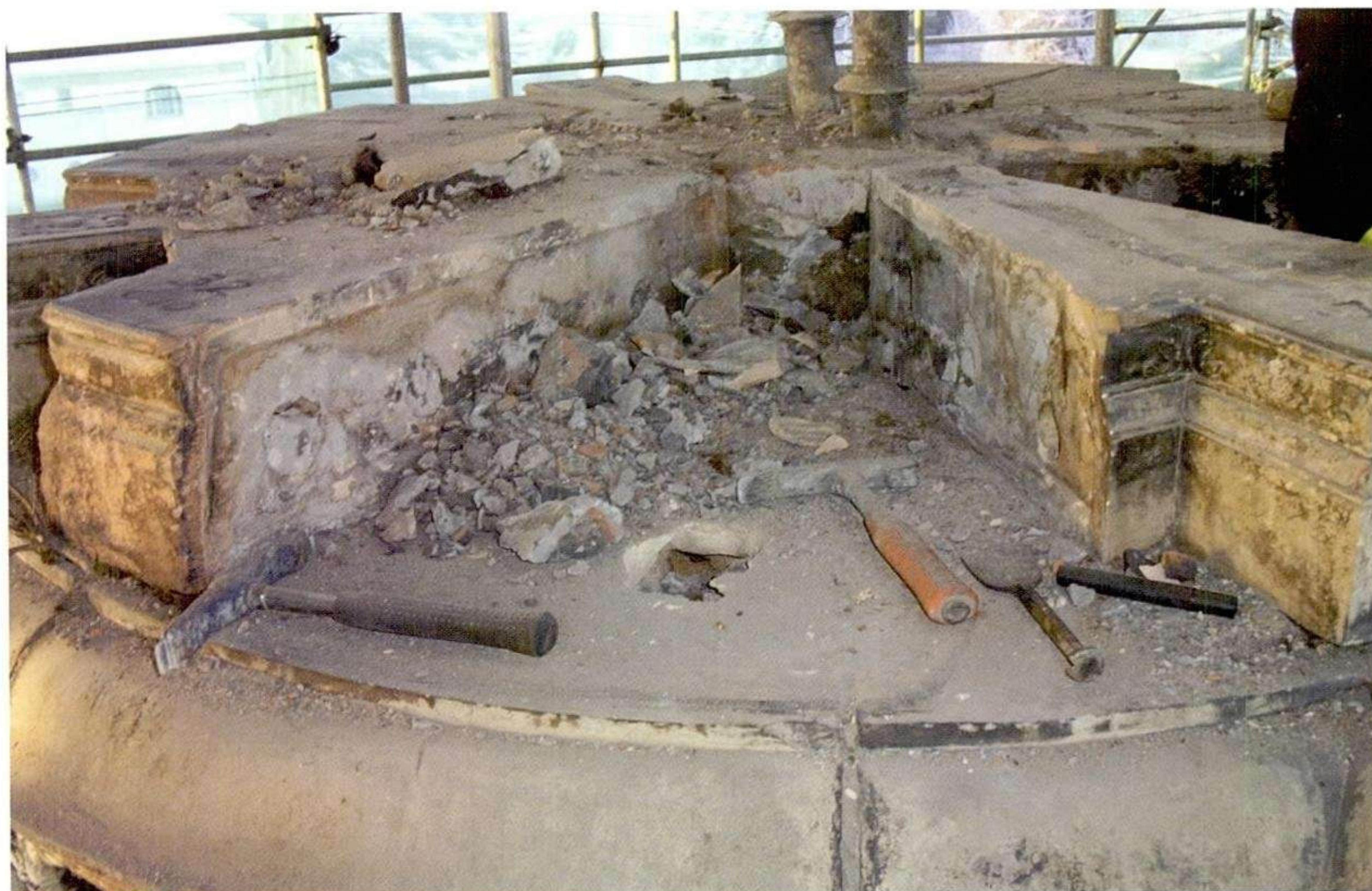
The terracotta blocks were taken down by experienced stone masons using hand held tools.
