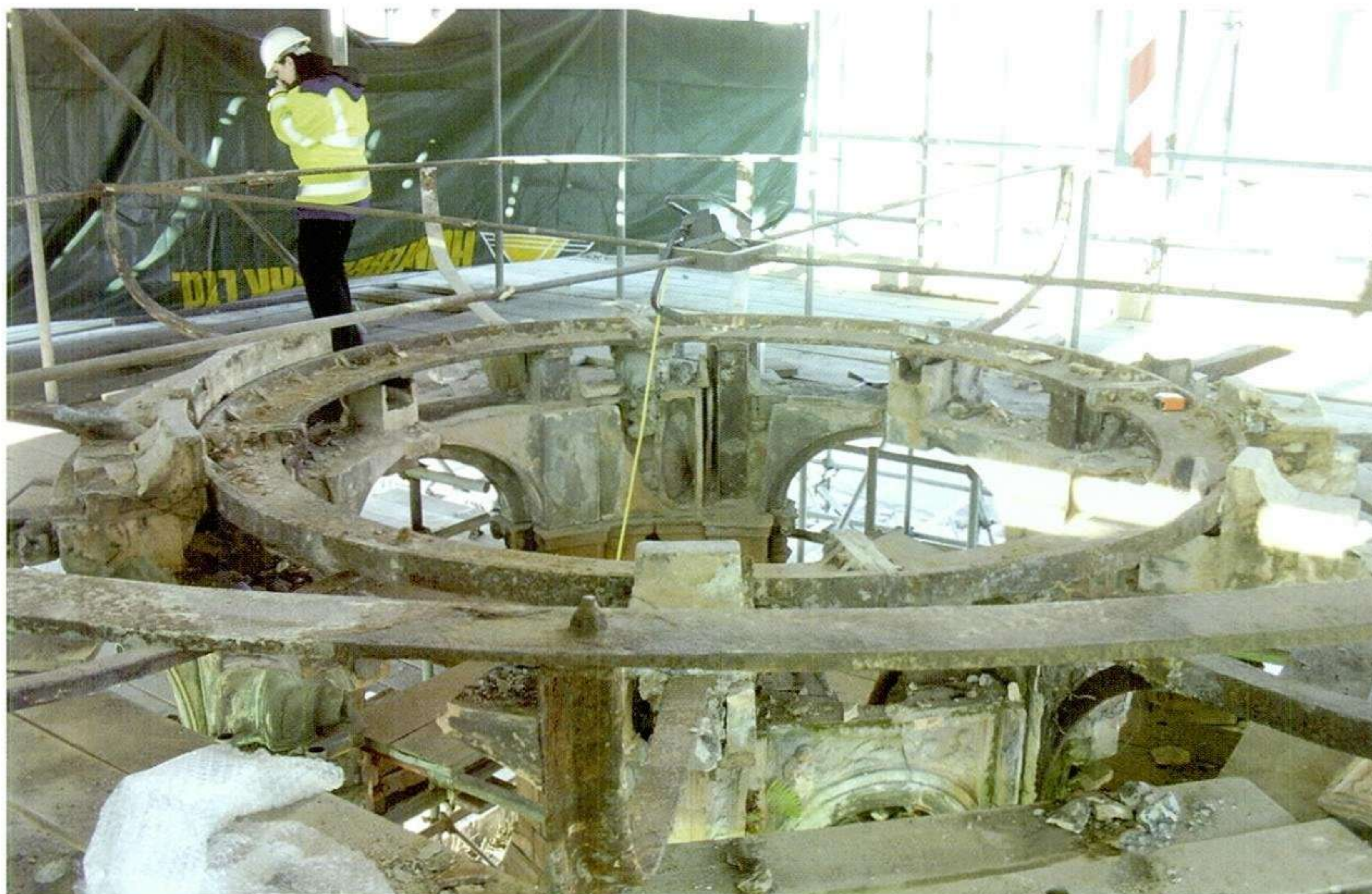
The cast iron and wrought iron frame of the cantilevered basin, exposed and prior to dismantling.
