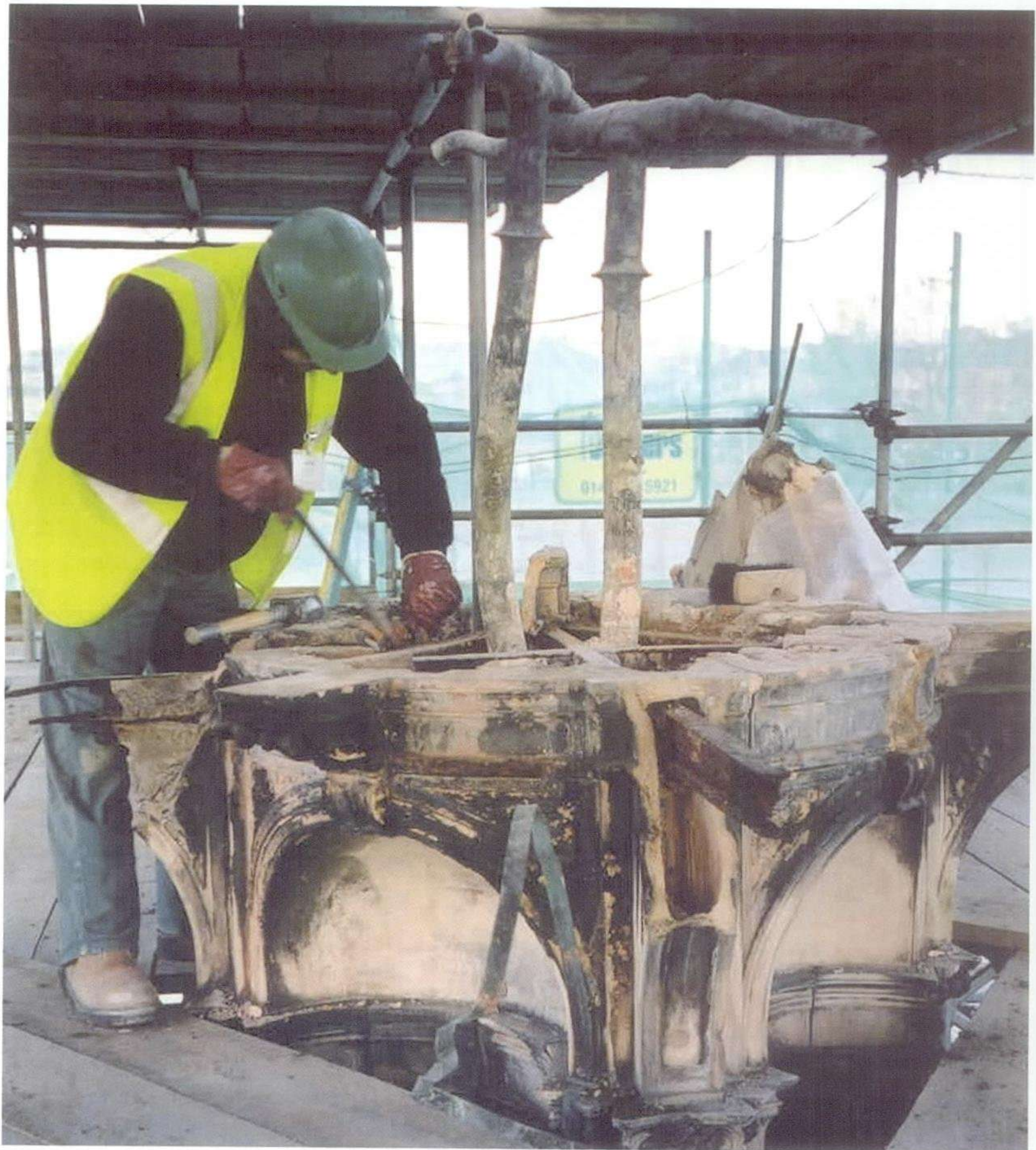
The unique reference number of each block was marked on internal faces. The dismantling process involved the careful of original plumbing and reinforcing.
