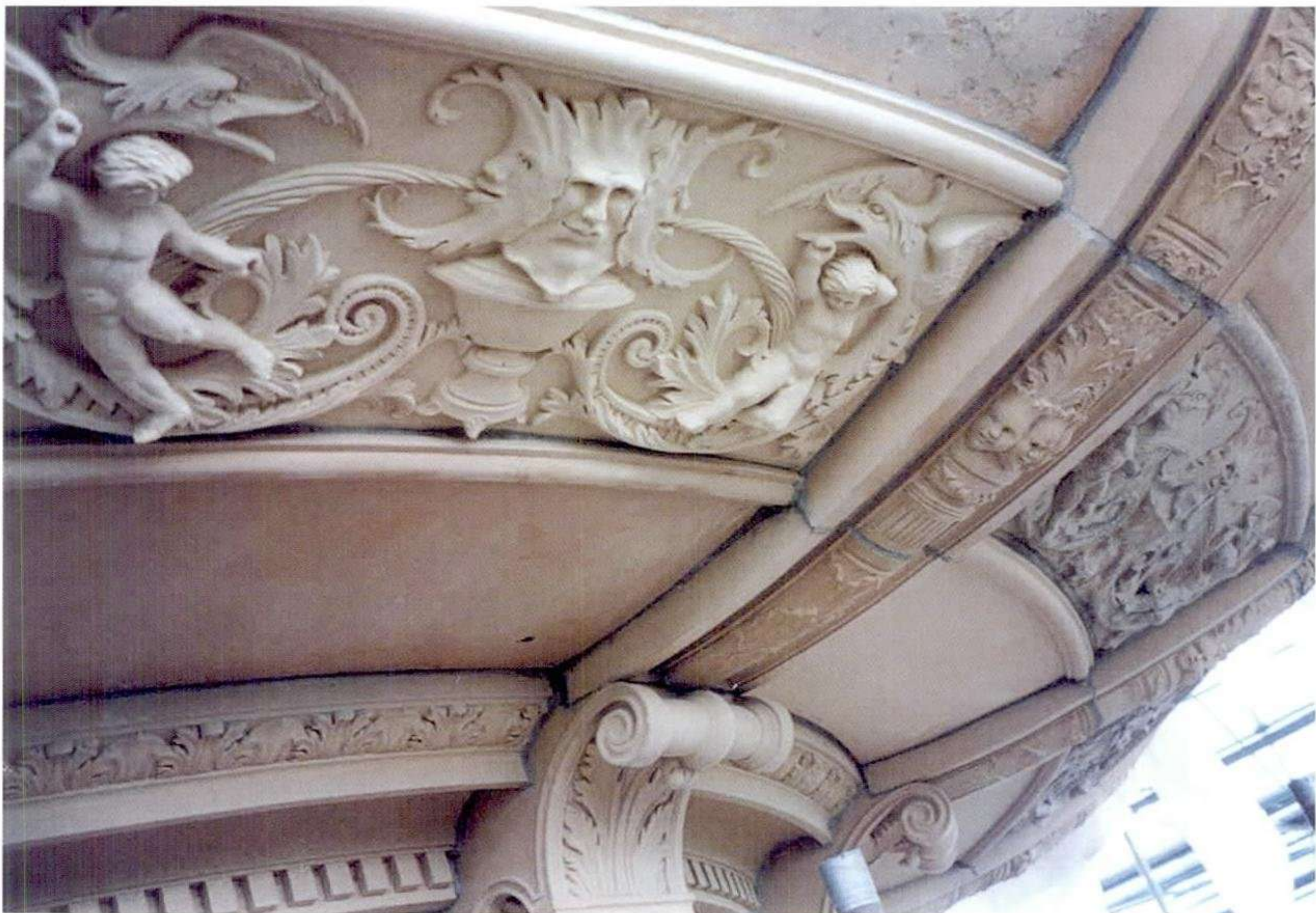
The pieces of the cantilevered basin were four different colours. Replacement terracotta reflected this diversity.
