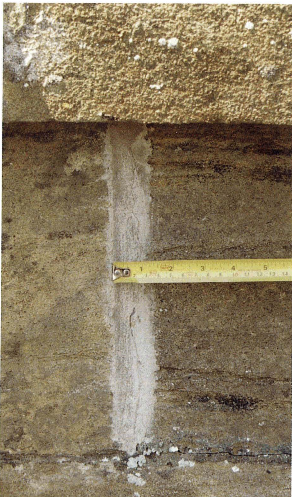
Figure 69. Poor quality repairs to ashlar jointing. Note the poor workmanship, inappropriate materials and failure to treat the cracked horizontal joint. Repairs such as these are not acceptable on a Listed Building and they may cause later problems to the façade.
