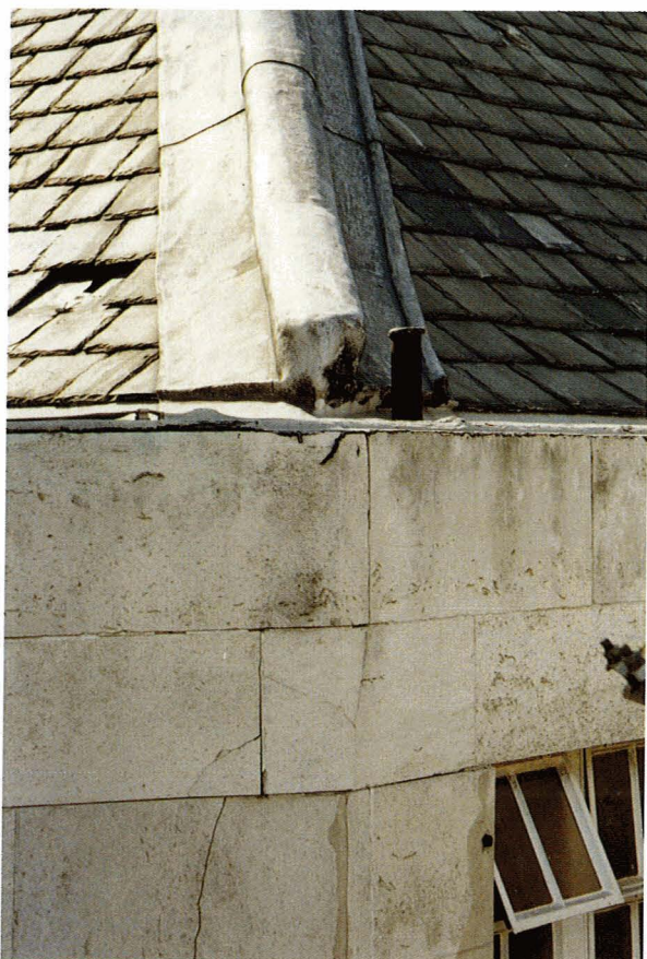
Figure 16. Cracked and displaced masonry due to corrosion resulting from poorly maintained roof.
