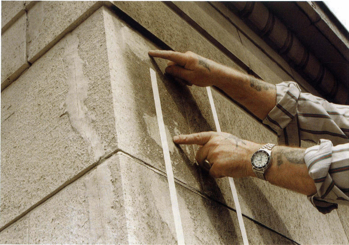
Figure 72. Repairs carried out on a Portland stone façade using stainless steel pinning. The tape marks the flanges of the underlying steel and the mason points to the pin locations.
