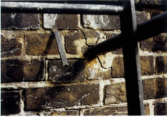
Figure 37. Photograph showing cracking of brick masonry due to corrosion of the fire escape fixing.
