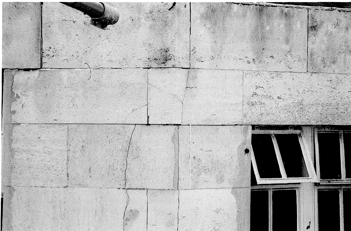
Figure 1. Cracking and stonework displacement due to corrosion of the underlying steel column.
