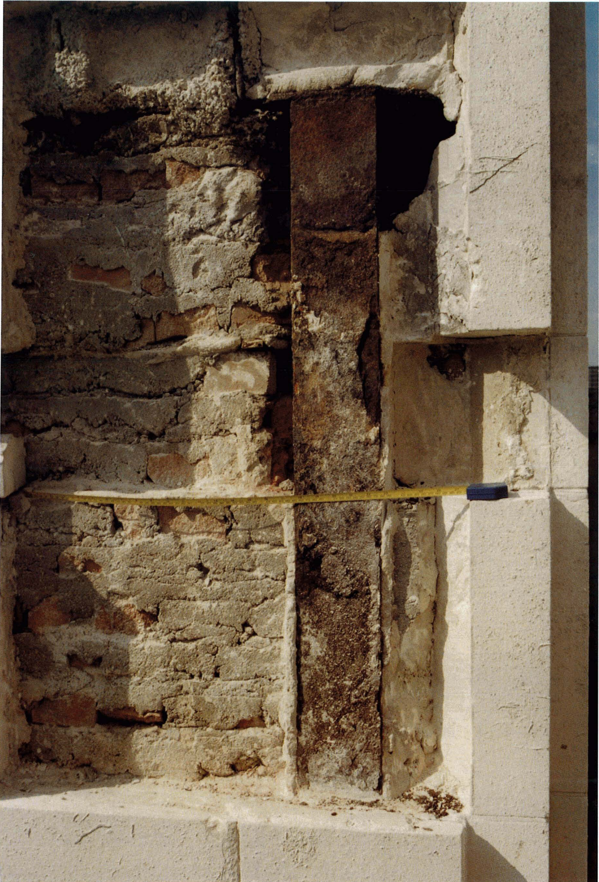
Figure 44. Removal of cracked and associated stones confirms corrosion of the column flange as the cause of cracking as shown in Figures 42 and 43.
