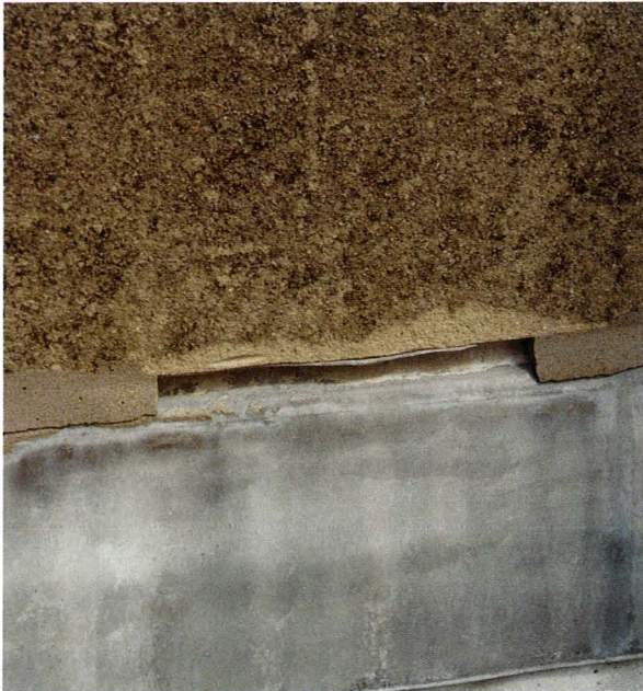
Figure 34. Poor ragging of a parapet flashing. Faults such as these can result in the rapid penetration of moisture and corrosion of the underlying steelwork due to water penetration behind the flashing.
