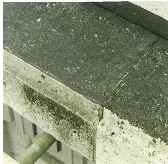
Figure 33. Closer inspection reveals failure of the bituminous waterproofing layer at ashlar joint locations due to thermal movements of the underlying masonry.
