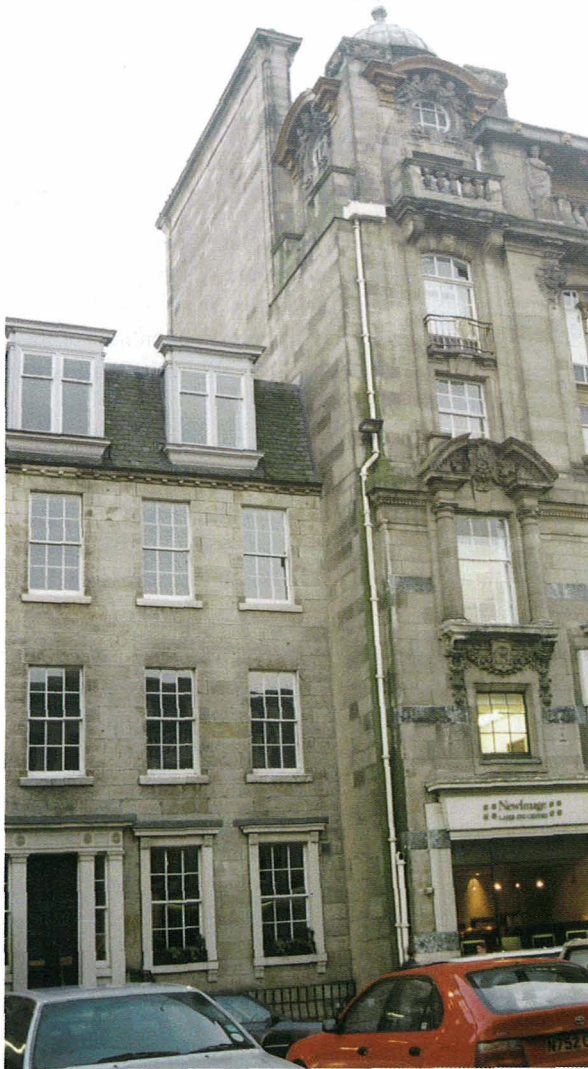
Figure 31. Biological growth around cracked rain water pipe indicating failure.
