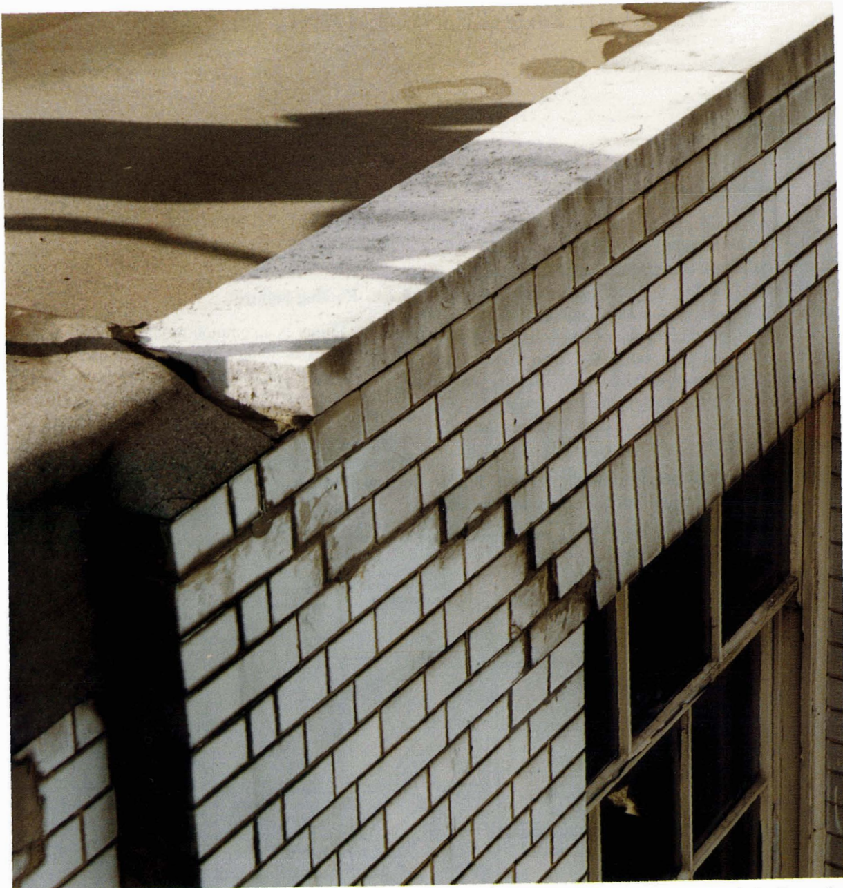
Figure 14. Severe corrosion jacking above a glazed brick window head due to water penetration through a faulty flat roof.
