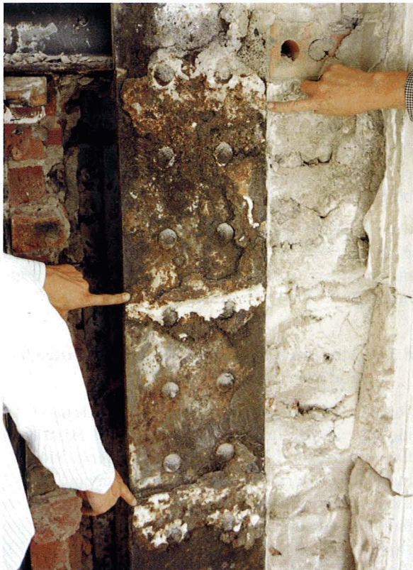
Figure 18. Opening up of a column reveals corrosion problems due to moisture ingress through cracked ashlar jointing. Note the additional corrosion product at the joint locations.
