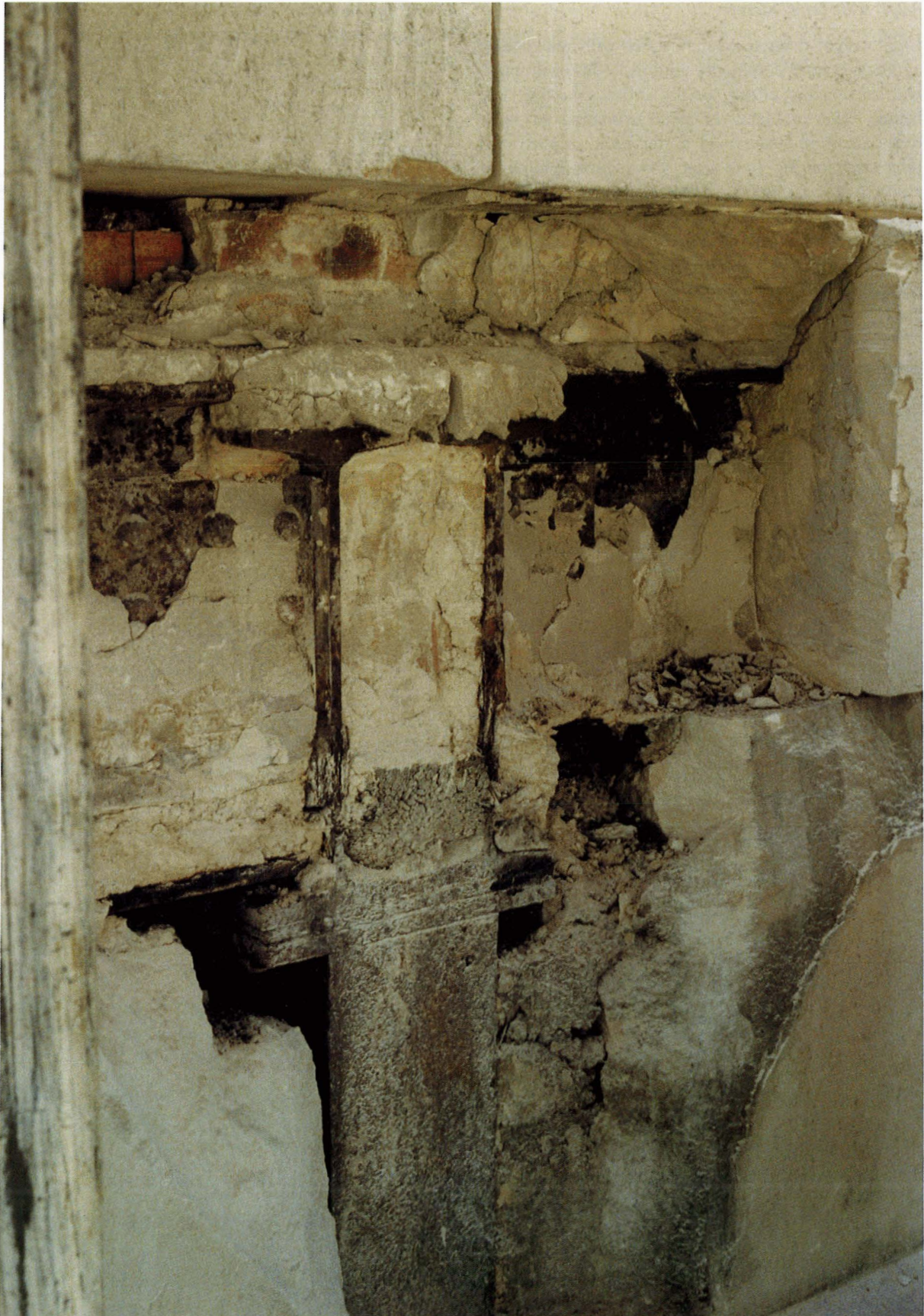
Figure 6. Mortar infilling and notched stonework around steel columns and beams. Note the large void at the plated connection due to difficulty in in-filling at the time of construction.
