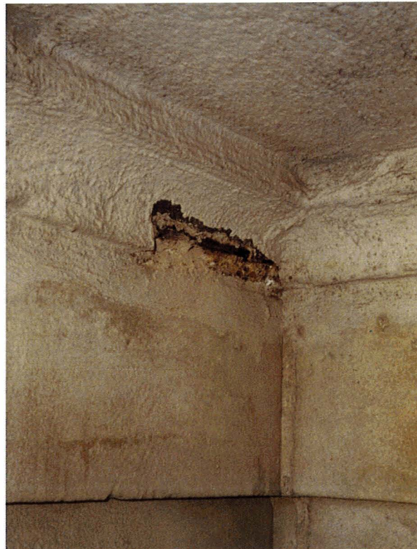
Figure 39. Spalling of a high level cornice repair due to corrosion of the mild steel fixing.
