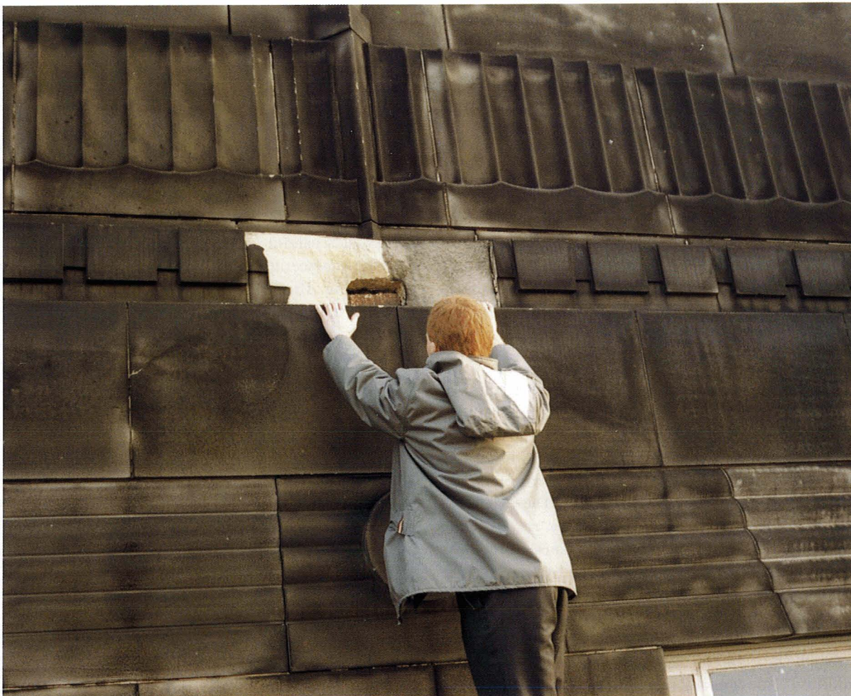
Figure 2. Large stone spall due to corrosion of the steel column. Cases such as these are clearly a potential safety problem and detailed investigations and remedial actions are required to prevent reoccurrence.
