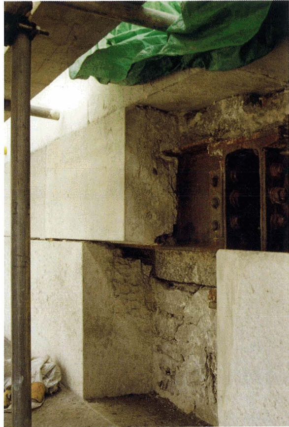
Figure 19. Moisture diffusion through the parapet stone work results in corrosion of steel work. In this case corrosion has resulted in enlargement of the joint adjacent to the lower flange.
