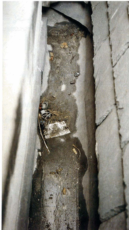
Figure 24. Blockage of rainwater outlet pipe in gutter.
