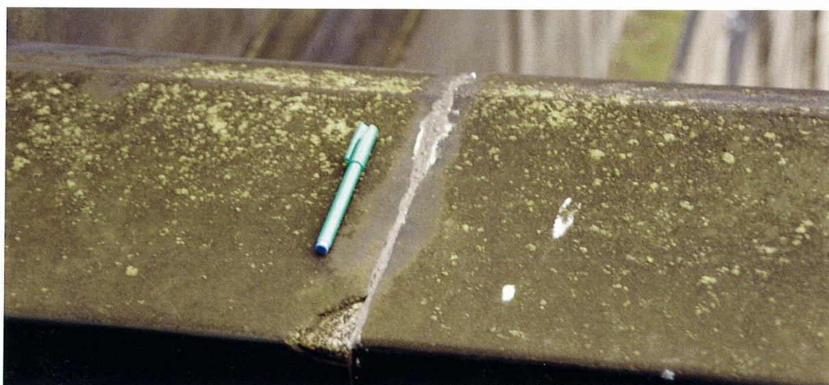
Figure 70. Sealant staining due to inappropriate materials selection on the coping stones of a sandstone parapet wall.
