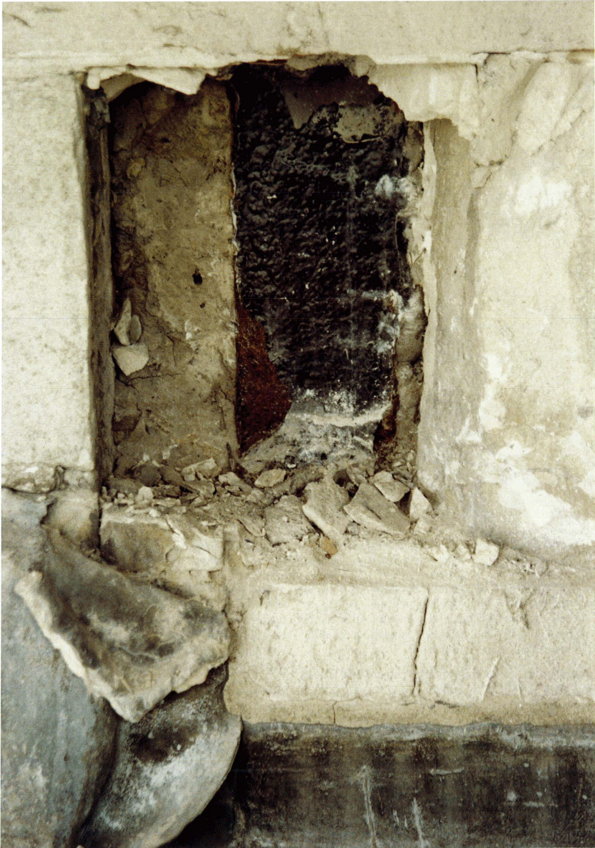
Figure 10. Bituminous paint systems such as these are rare in steel framed buildings and provide little corrosion protection.
