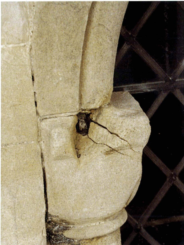
Figure 38. Damage caused by the corrosion of iron and steel fixings has been known for many years. This figure shows damage caused by the corrosion of a small iron fixing. In steel framed buildings the corrosion of any iron or steel fixings results in a similar problem. However, cracks and damage to the façade allows the direct penetration of moisture and corrosion of the steel frame.
