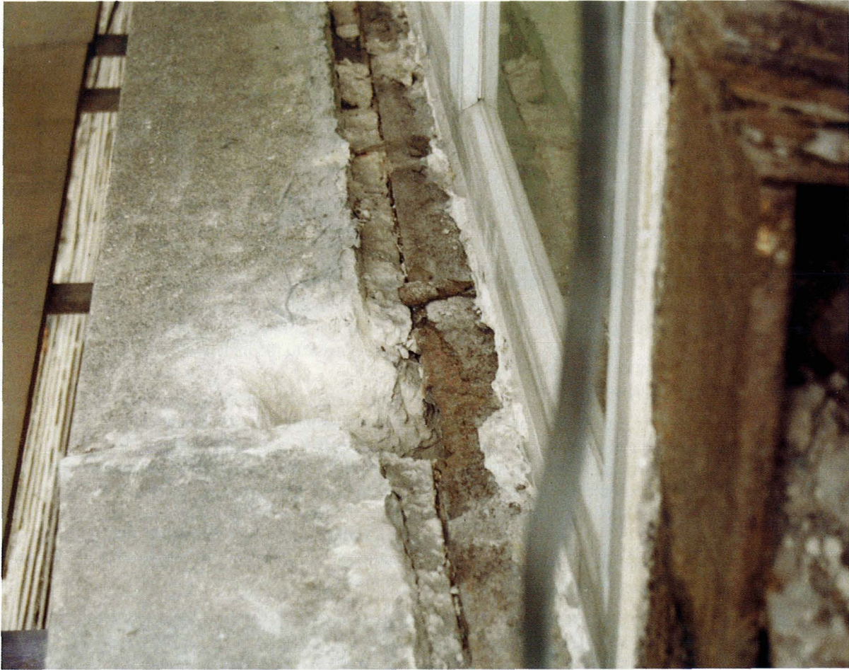
Figure 36. Poor quality window replacement can result in the penetration of water. Note - the corrosion of underlying steel work with insufficient concrete cover.
