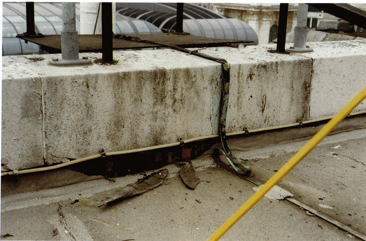
Figure 15. Failed upstand and cracked asphalt on flat roof.
