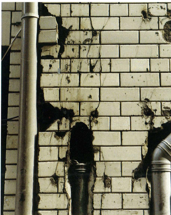
Figure 30. Failure of the glazed brick was attributable to corrosion of the steel frame resulting from leakage of the exiting rainwater pipe from within the wall.
