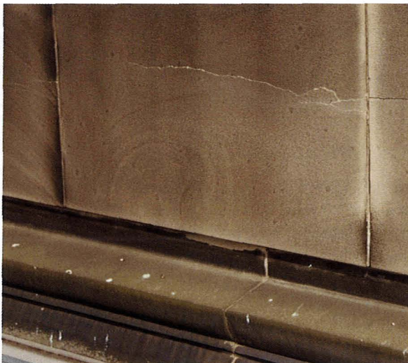
Figure 40. Photograph showing crack in a sandstone parapet. Fine cracks such as these are easily missed in binocular surveys or inspections from a distance.
