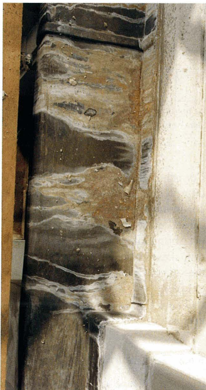
Figure 23. Staining of cornice cover flashing due to water overflow as a result of blocked guttering.
