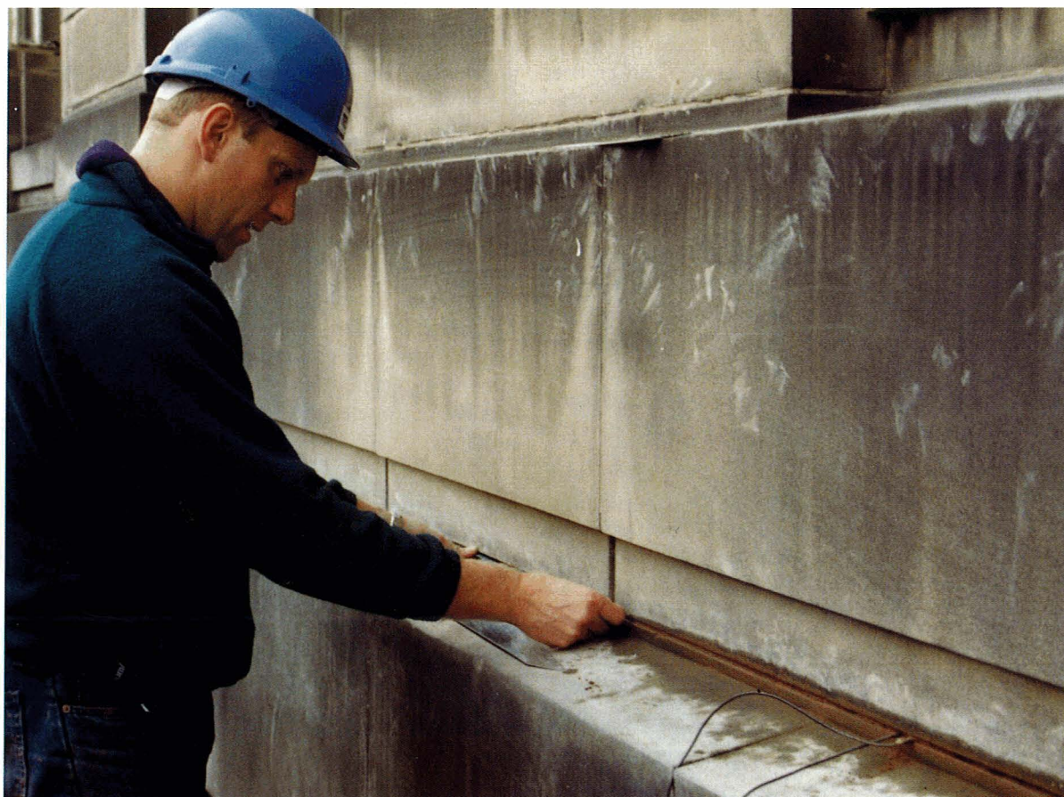
Figure 67. Installation of a mesh ribbon anode into the beds of ashlar stonework.
