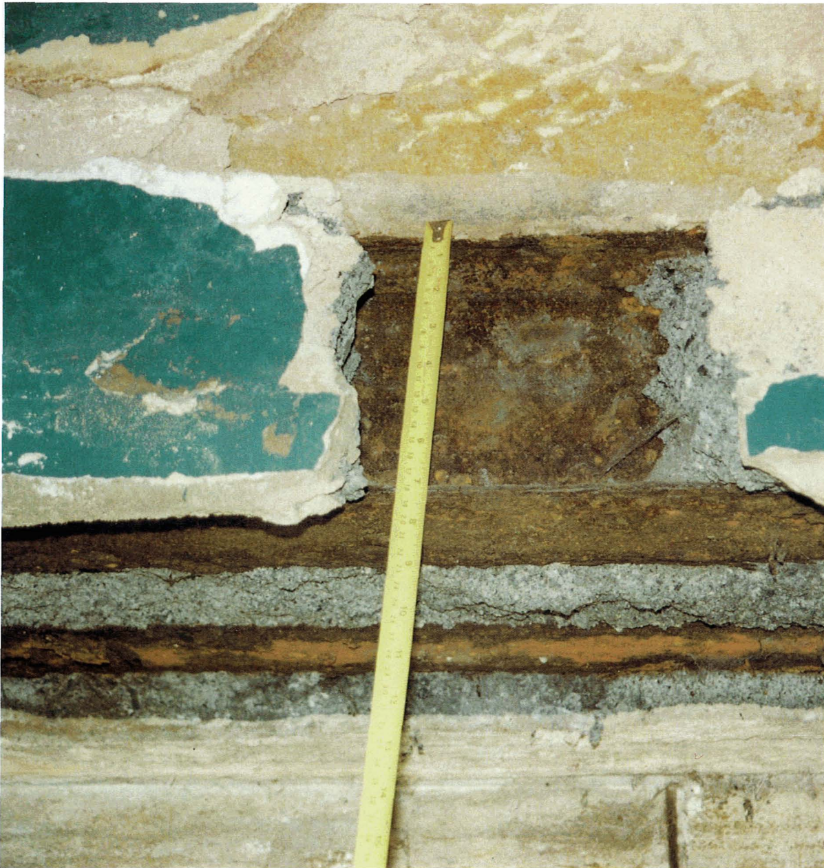
Figure 7. Severe corrosion of this double 'I' section encased in clinker concrete resulted in internal spalling of the concrete and plaster.
