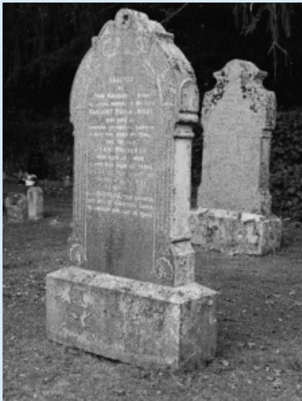
An unstable granite headstone. The gap between the base and the foundation indicates potential instability of the whole memorial. Careful examination of the joint between the slab and base reveals a hairline crack in the biological growths at this point. This headstone could be easily overturned by moderate pressure.
