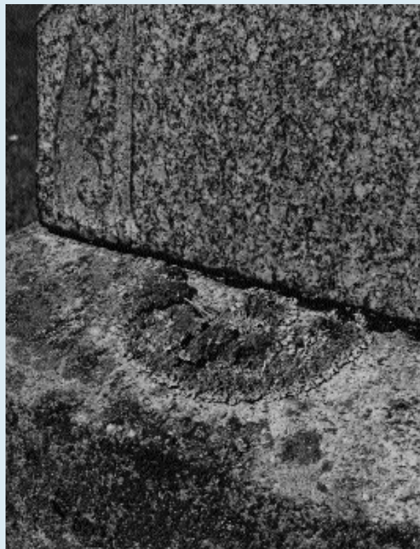
The joint between slab and base shows disruption of the biological growths and indicates movement between the slab and base.
