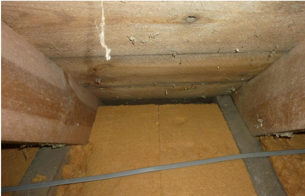
Figure 7: Wood fibre board insulation to the attic space, showing vented gap below the sarking
