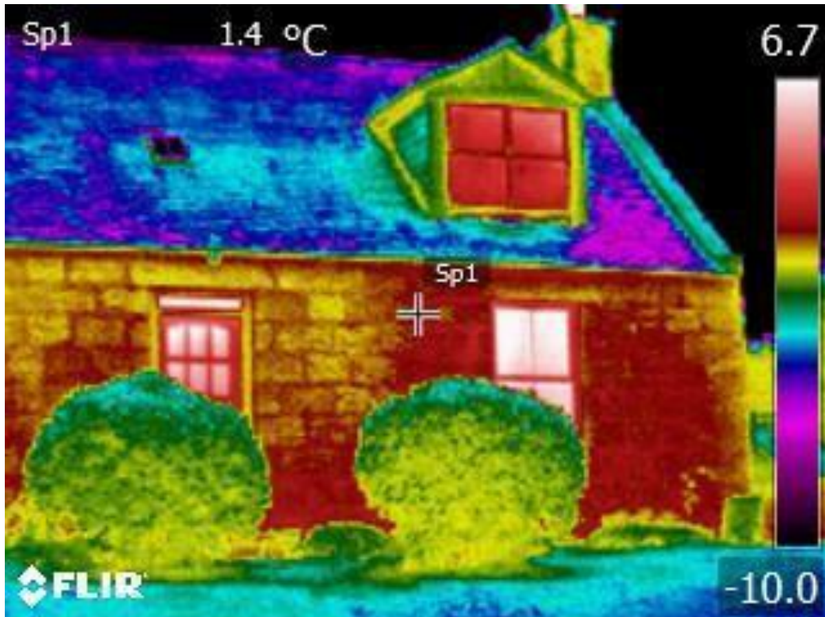
Figure 5: Thermal image of the front elevation, showing the better than expected performance of the roof. External air temperature 1.4°C
