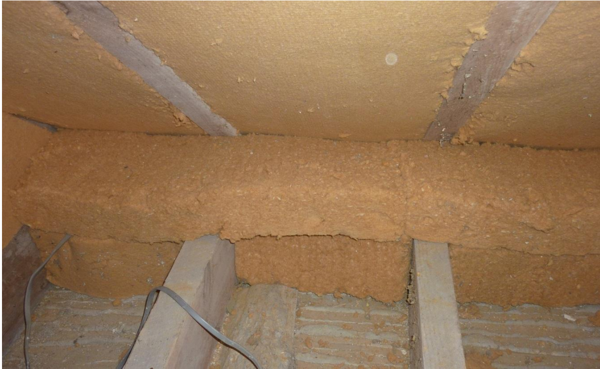
Figure 8: Wood fibre board insulation at the junction of the roof and the wallhead.
