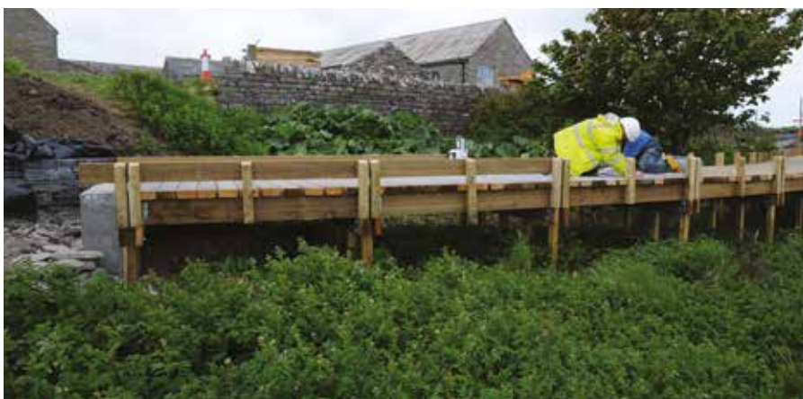
Construction of the boardwalk section of the new pathway at the Ness of Brodgar
