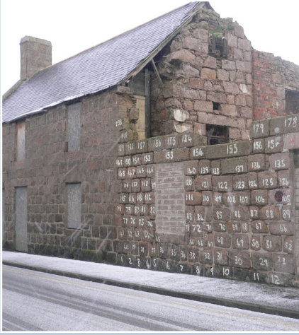
Structural instability requires the rebuilding of this wall in Peterhead. The granite stones have been numbered ready for reinstatement.
