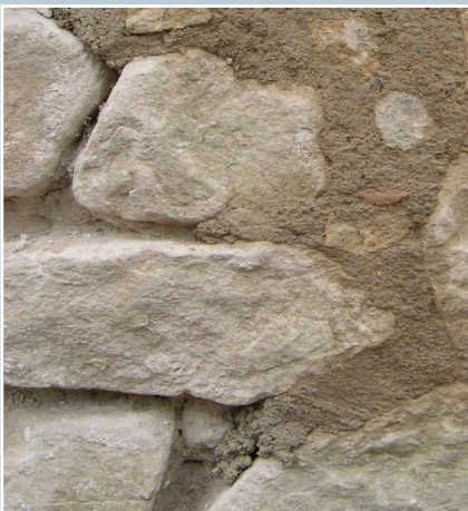
Modern lime mortar pointing, Scottish Lime Centre, Charlestown, Fife. The use of lime allows the wall to 'breathe'. Traditionally, most rubble walls had lime slaistered, or buttered, over the joint to achieve a fairly smooth finish that would erode with time. Where pointing does not alter the character of a listed building it would not normally require consent.
