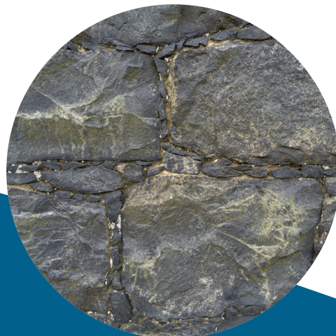
Tightly pinned mortar joints in whinstone masonry - Collinsburgh, Fife.
