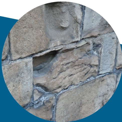
Deterioration of stonework adjacent to incompatible cement based mortar.
