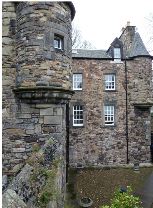
Figure 2.1. View of the rear of CS1 from the East (Source: Vicky Ingram)
