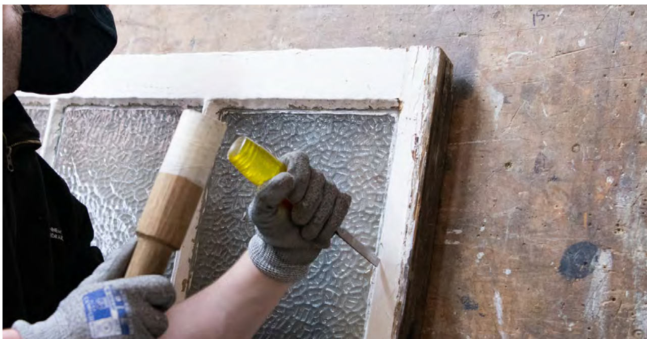
Figure 67: An apprentice joiner at our Stirling Depot repairs a timber window frame. Timber is often removed and replaced when it could easily be repaired.
