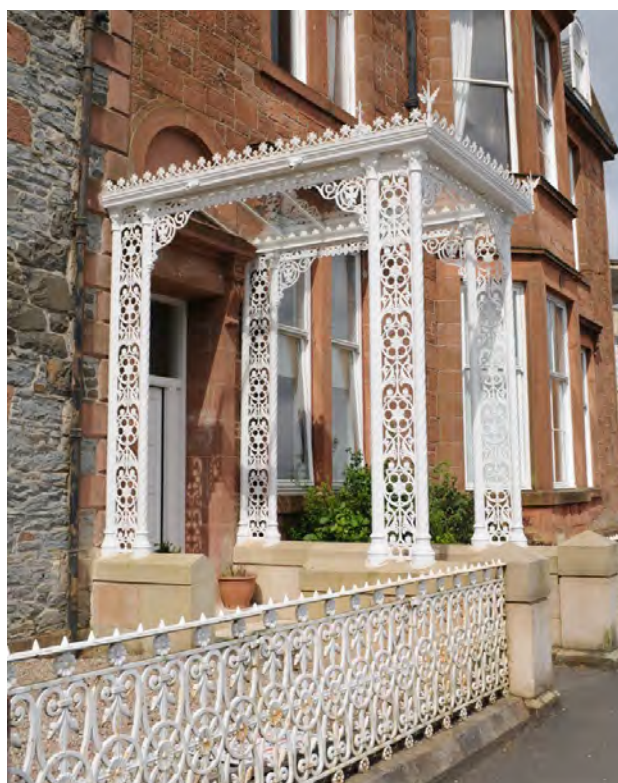
Figure 19: Cast iron was used extensively for railings and other decorative items. This example is from the Isle of Bute.
