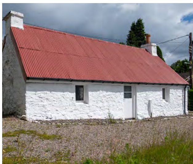
Figure 12: Sunnybrae Cottage, an earth-mortared building in Pitlochry. Earth-cored or earth-mortared buildings are often misidentified or overlooked.
