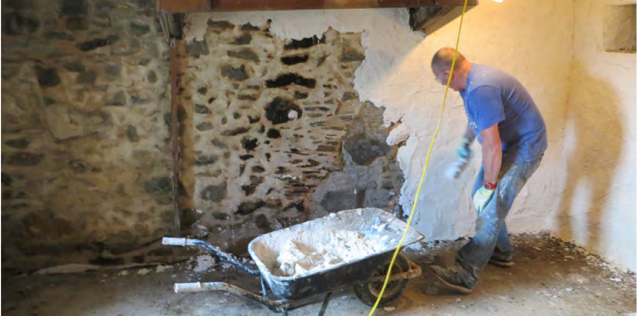
Figure 32: First coat of insulated lime plaster being applied at Downie's Cottage near Braemar. Lime coatings can be used to improve building resilience and energy efficiency.
