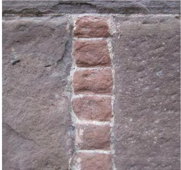
Figure 35: It is important that mortar specifications deliver appropriate performance, behaviour and aesthetics based on an understanding of the original.
