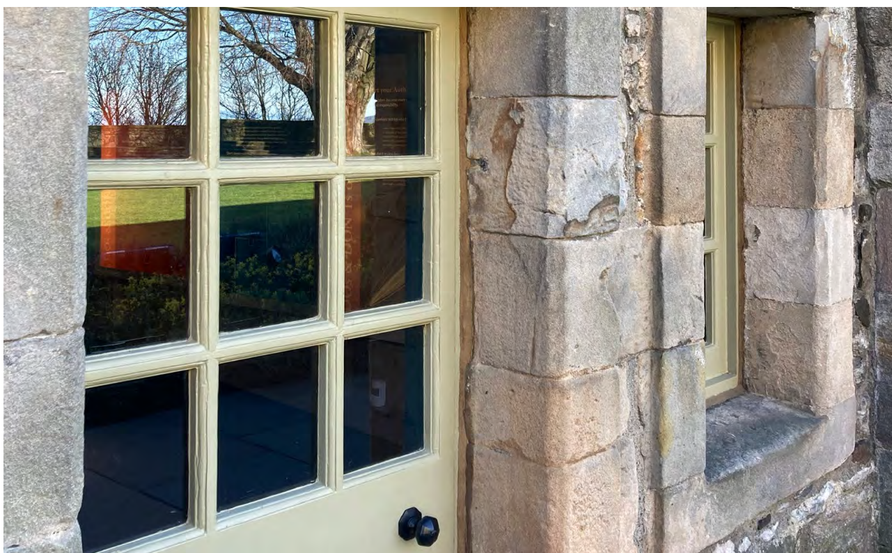
Figure 41: Linseed paint has been used for redecoration of windows and doors at Stirling Castle.
