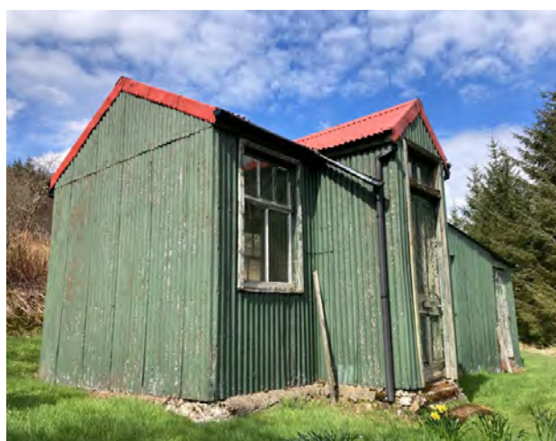
Figure 20: Scotland was a world leader in producing and exporting corrugated iron during the 19th century. This example was a school in the Scottish Borders. © Sanne Roberts
