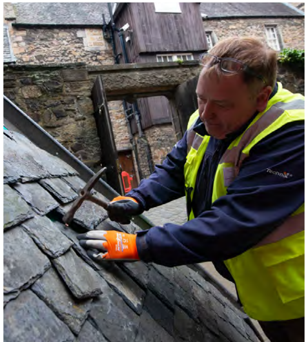
Figure 53: The loss of distinctive Scottish slate roofs risks the disappearance of the specific skills and knowledge needed to lay them.
