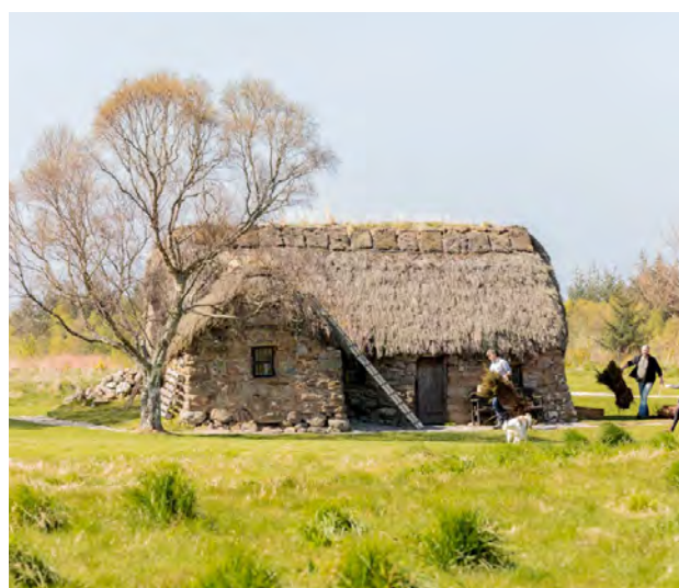
Figure 55: A heather-thatched cottage at Culloden under repair. Thatched roofs require regular maintenance to keep them in good condition. © Malcolm McCurrach
