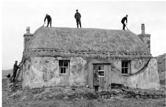
Figure 61: These crofters are re-thatching a croft on the island of Eriskay. In the past, thatching was traditionally undertaken by local owners or communities. Today, owners and thatchers are often based outside the local area – meaning extra care must be taken to preserve regional detailing and materials.
