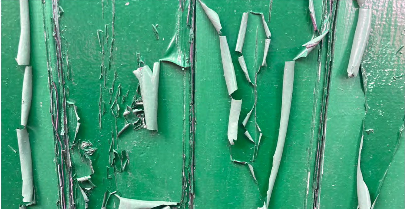
Figure 42: Poor preparation or specification can lead to premature failure and increase the environmental impact of paint. © Sanne Roberts
