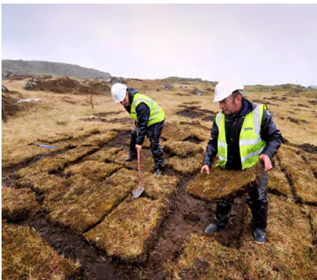
Figure 16: Cutting turf by hand is labour intensive and is not sustainable at a larger scale. © Donald MacLeod
