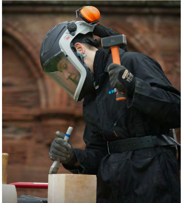
Figure 52: Apprentice stonemason at work. Replacement stone should be carefully chosen to match both the aesthetics and performance of the existing stonework, taking account of petrographic matching and how the stone will weather. © Rob McDougall
